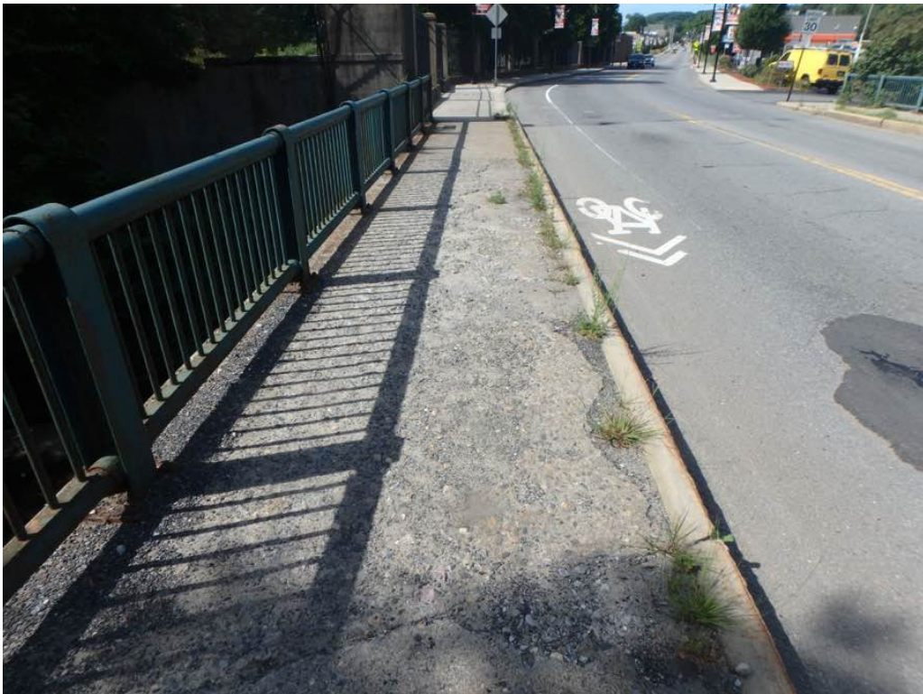
Photo 12: Heavy scaling to the East sidewalk, span #1.
