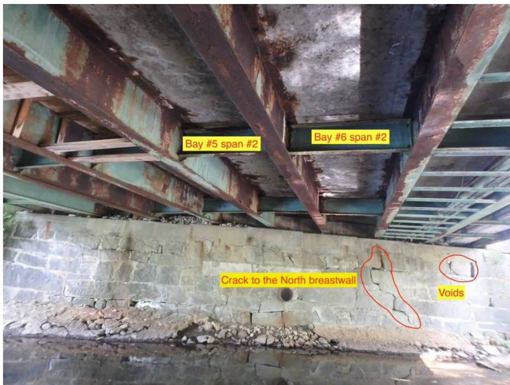
Photo 7: Bays #5 and #6 of span #2. Note crack and voids to the North breastwall.
