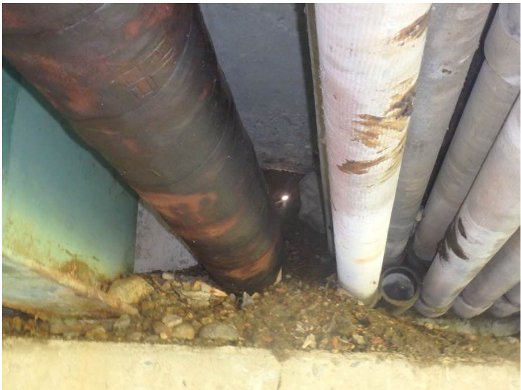
Photo 29: Fill from utility cutout at the South end of bay #1 in span #1. Note daylight.
