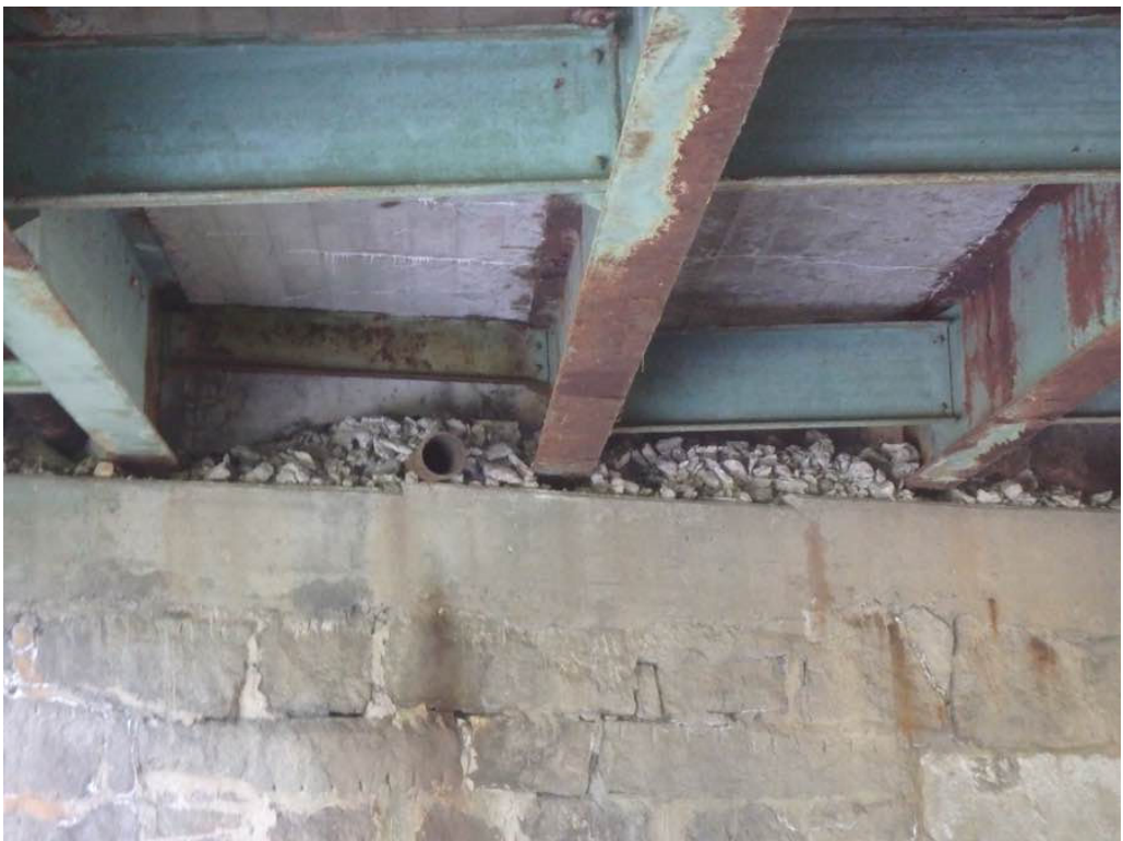
Photo 28: Debris on top of the North bridge seat in bays #2 - #4.
