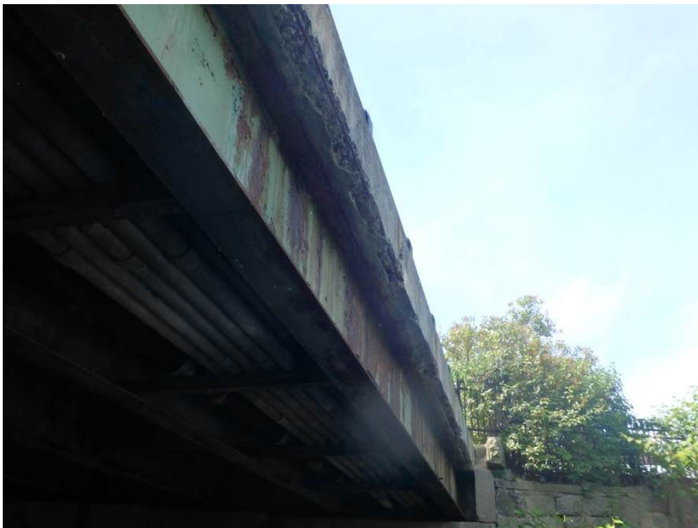
Photo 10: Typical spalls to the deck overhang at the West fascia, span #1.
