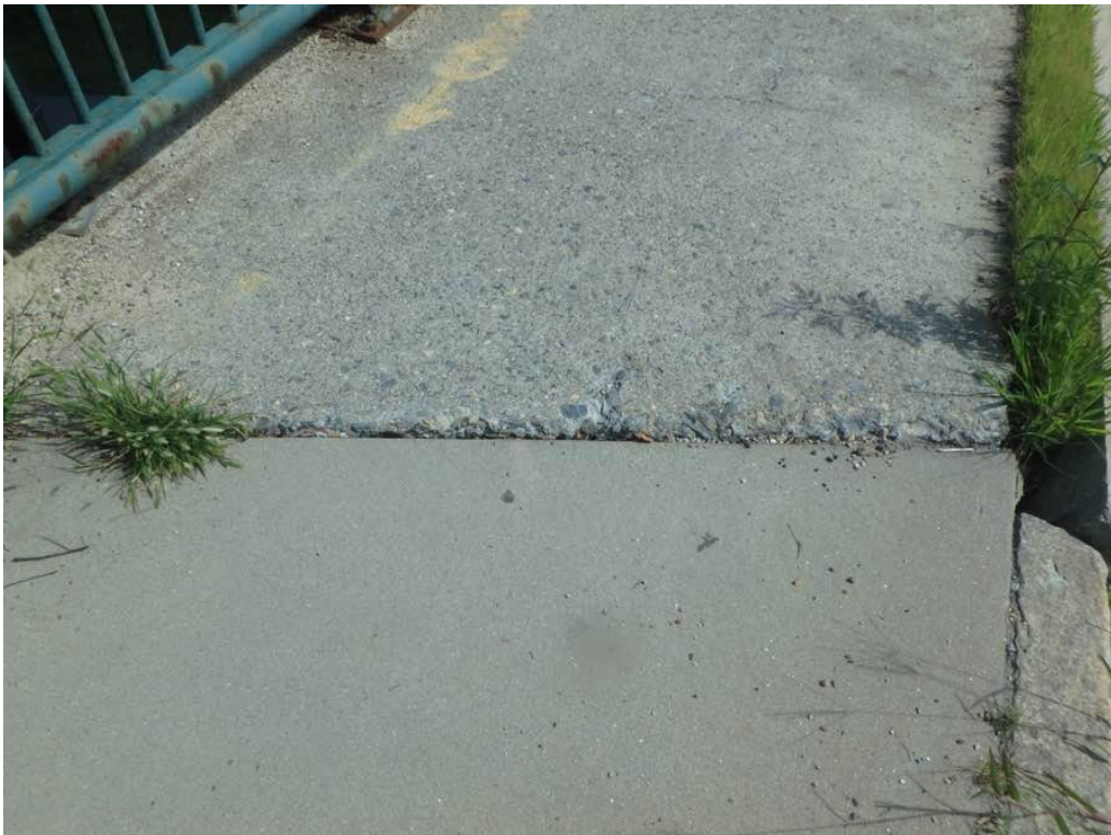
Photo 20: Southwest approach sidewalk settlement.
