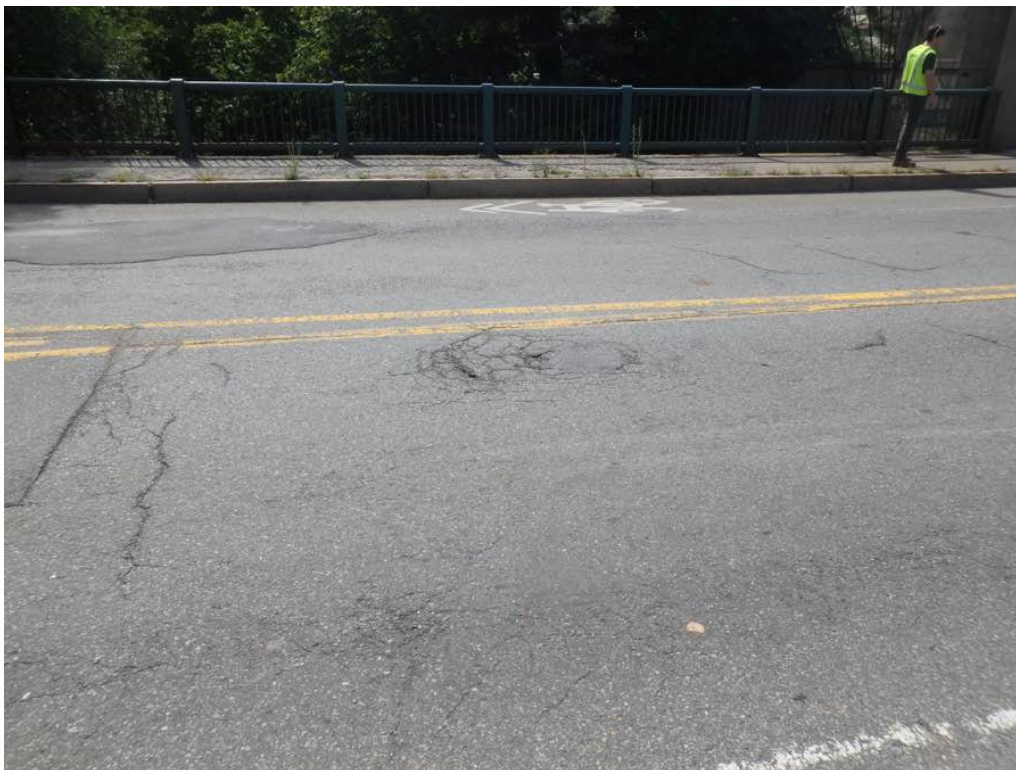
Photo 3: Cracking to the wearing surface at midspan of the structure.
