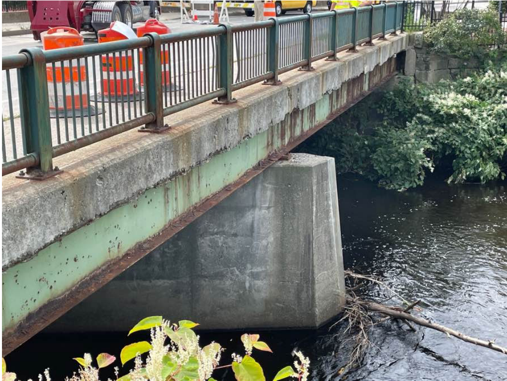
Photo 3: Debris at upstream channel nose
