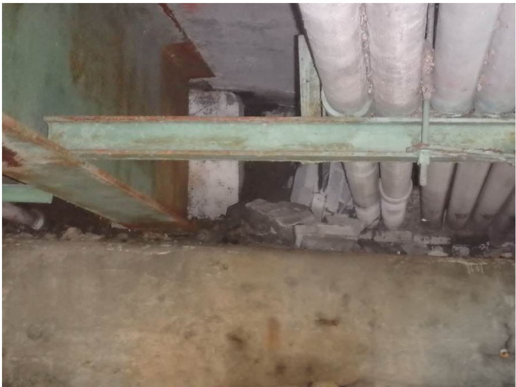
Photo 30: Collapsed brick around utility at the North end of bay #8 in span #2.
