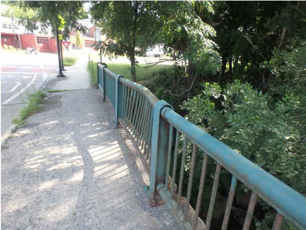
Photo 14: Bent rail at the North end of the East bridge rail.
