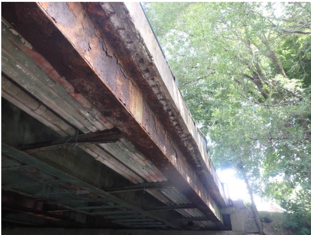
Photo 9: Typical spalls to the deck overhang at the East fascia, span #2.
