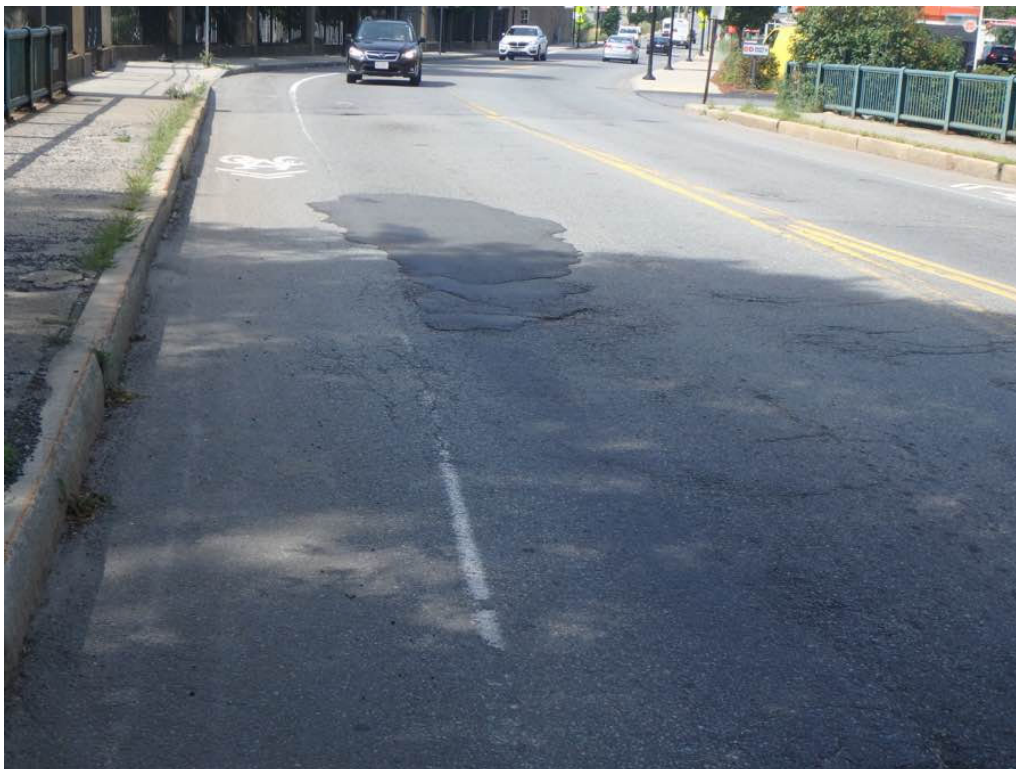
Photo 2: Large patch in the Northbound lane near midspan.
