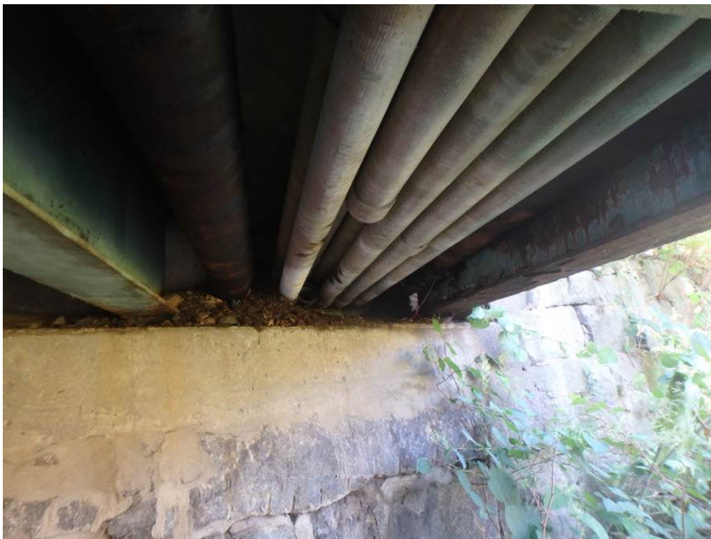
Photo 17: Missing section of the utility conduit in bay #1 near South abutment.
