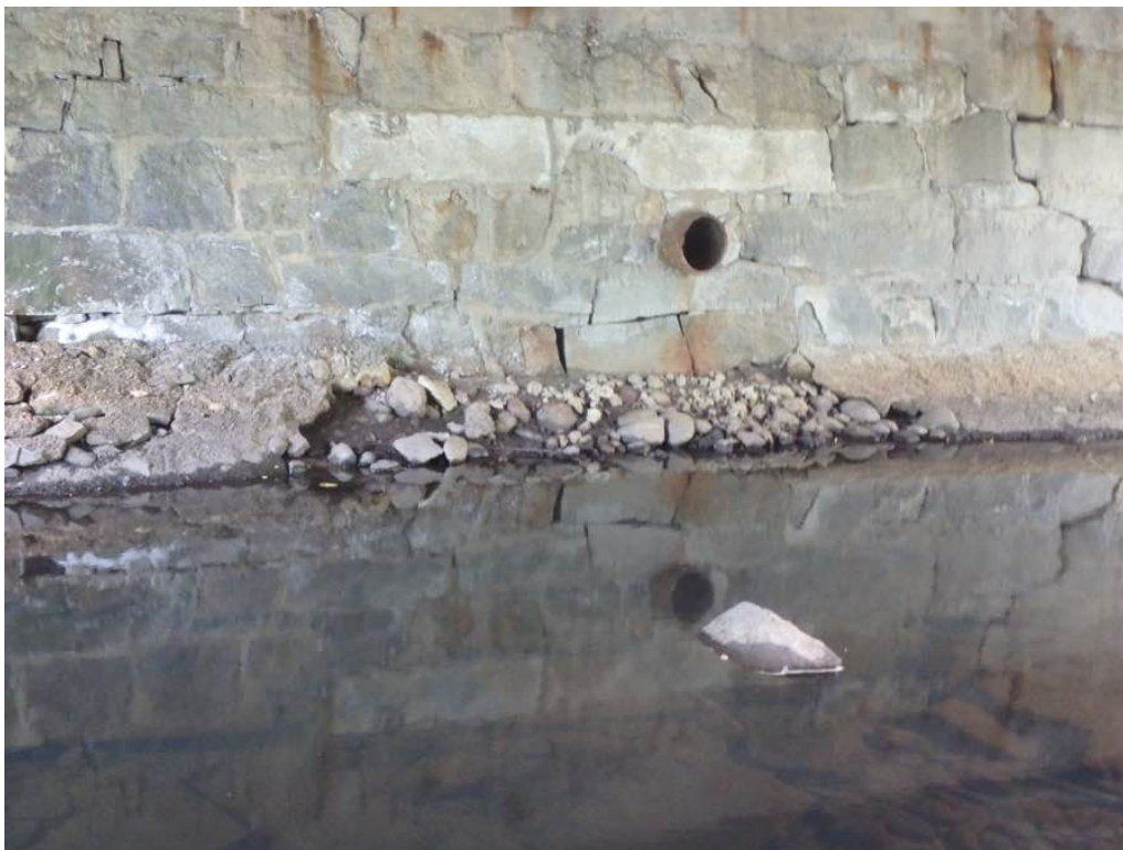
Photo 32: Missing scour protection at the North breastwall.
