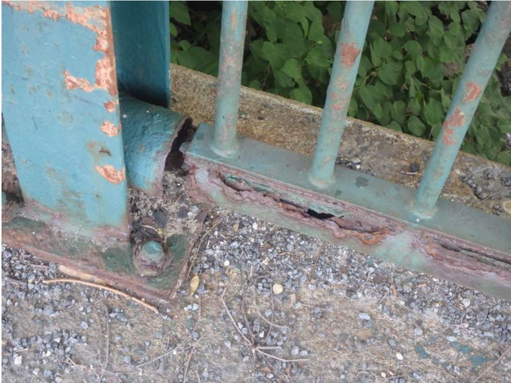
Photo 15: 100% section loss to the bottom rail of the East bridge rail at the North end.
