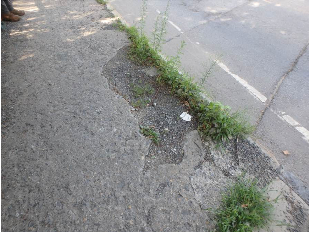
Photo 13: Spall to the North end of the East sidewalk.
