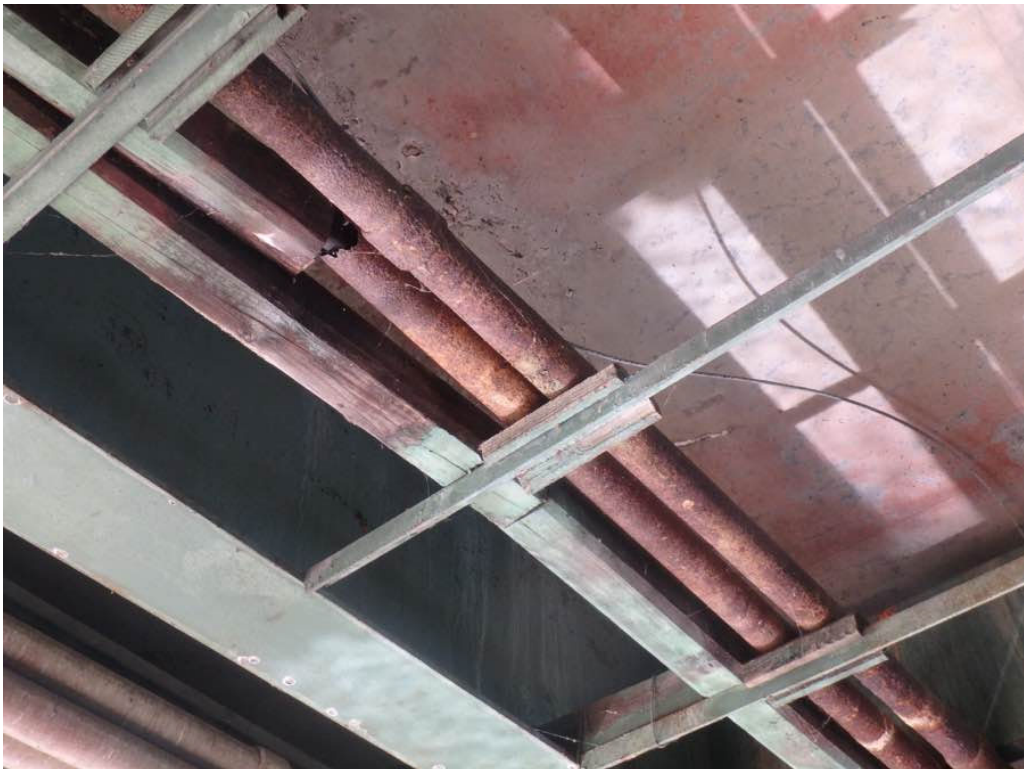
Photo 16: Typical corrosion of the utility conduits in bay #7.
