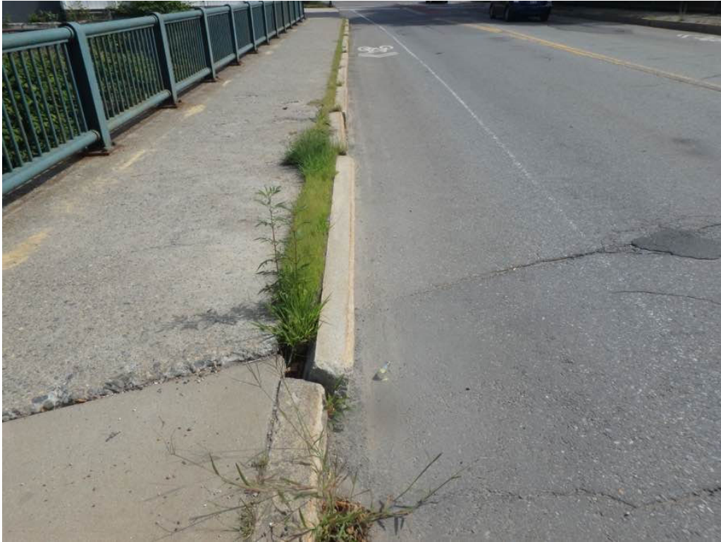
Photo 11: Loose curb stones at the South end of the West side.
