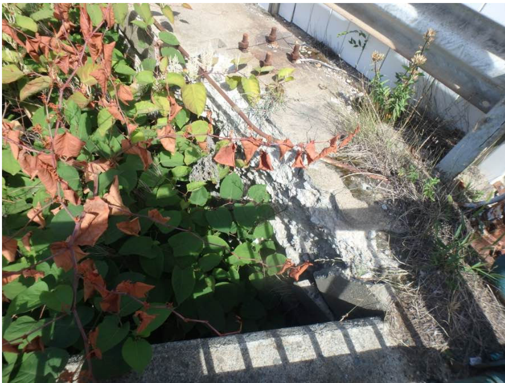
Photo 31: Heavy scaling to the top of the Northwest channel wall.
