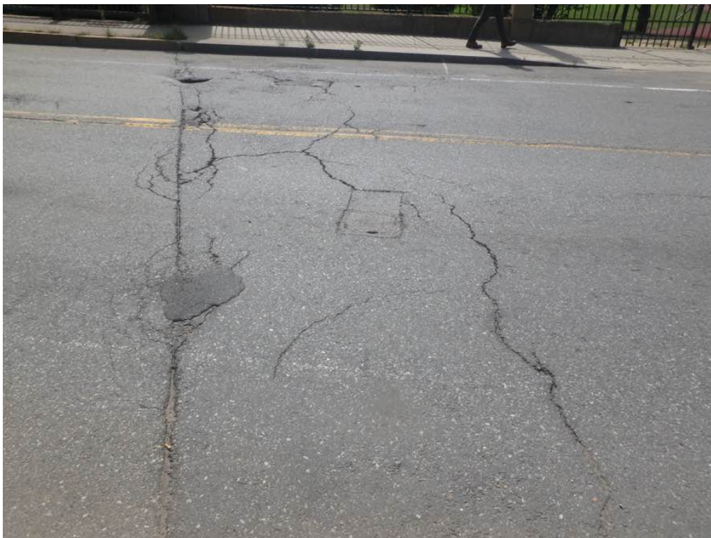
Photo 18: South approach to deck transition. Note pothole in the Northbound lane.
