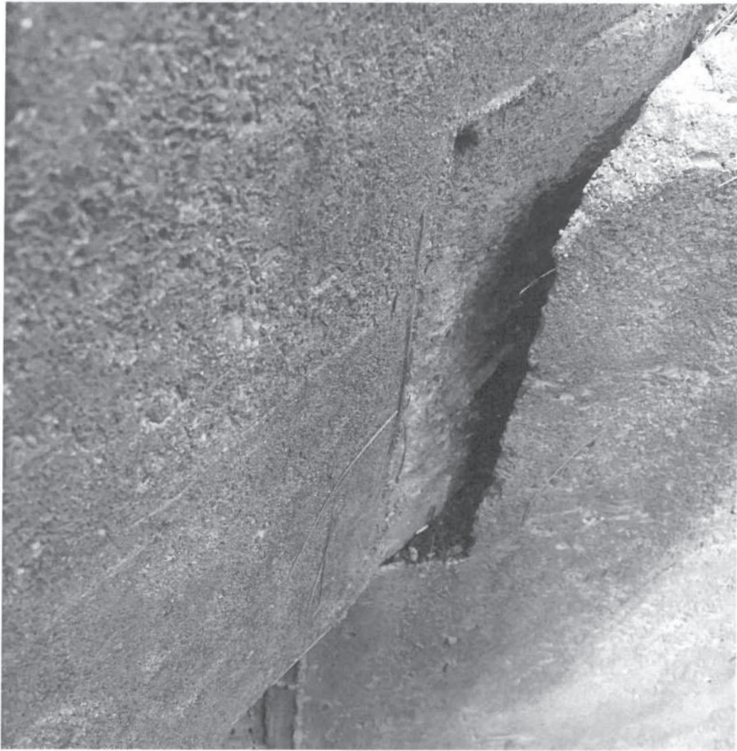
No visible caulking at joints
