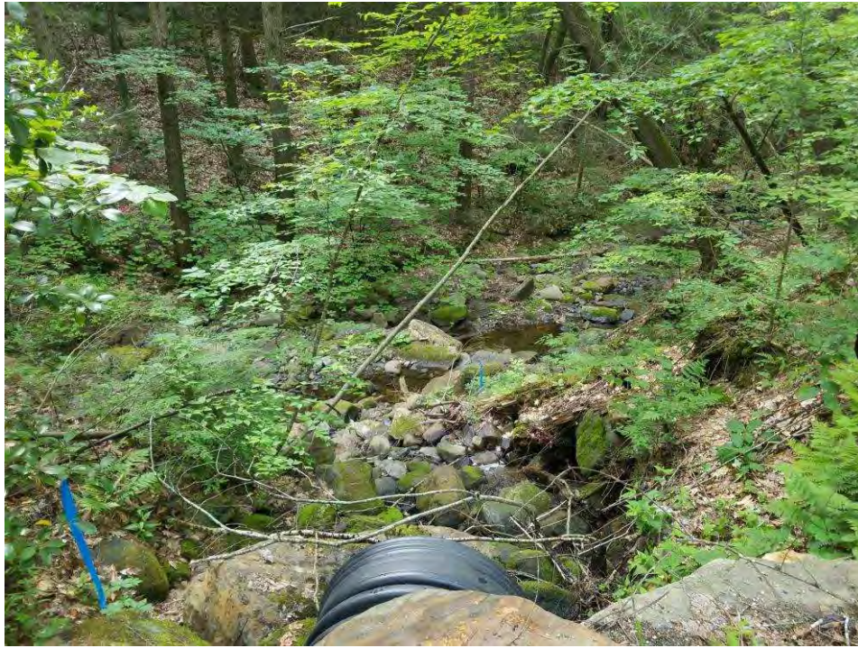
Culvert conveying flow to Oxbow Brook from the eastern side of East Oxbow Road.
