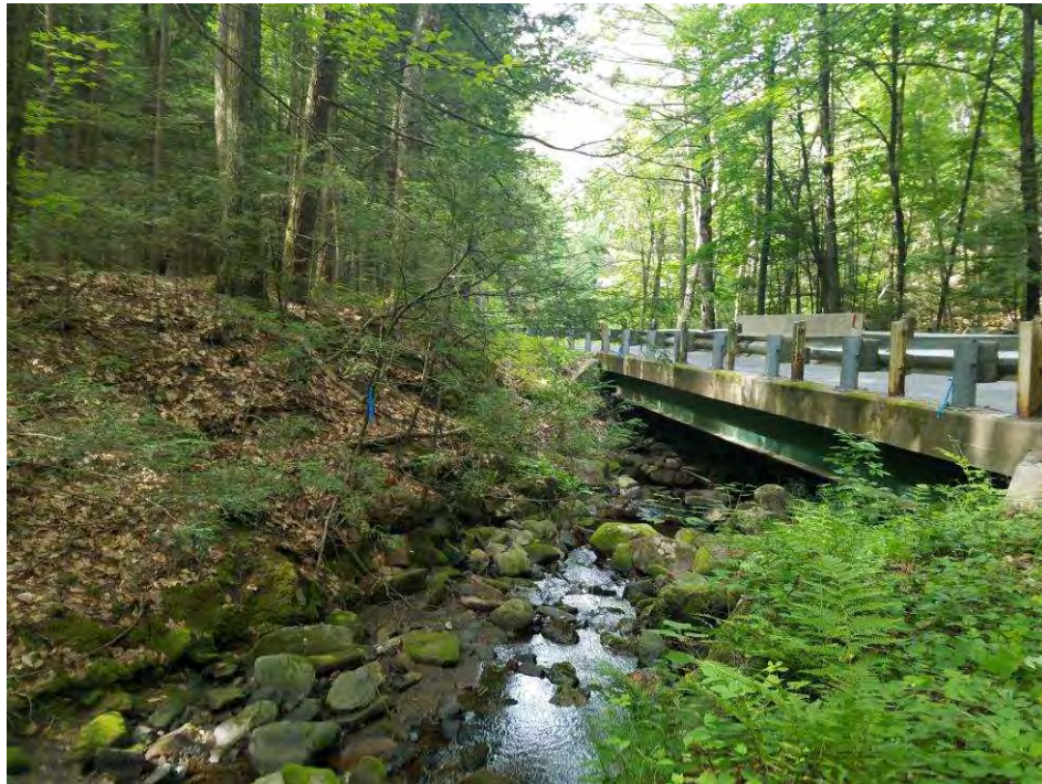
Looking south at Oxbow Brook and the bridge along East Oxbow Road.
