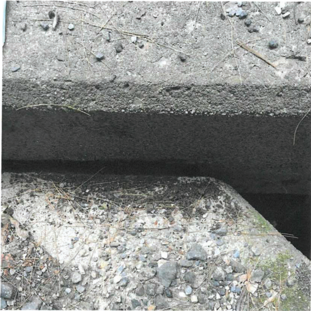
No visible caulking at joints
