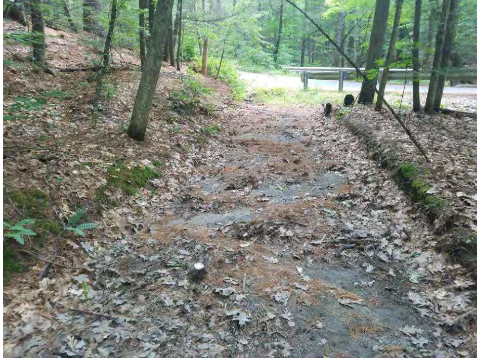
Non-jurisdictional channel conveying roadway runoff to Oxbow Brook from East Oxbow Road.
