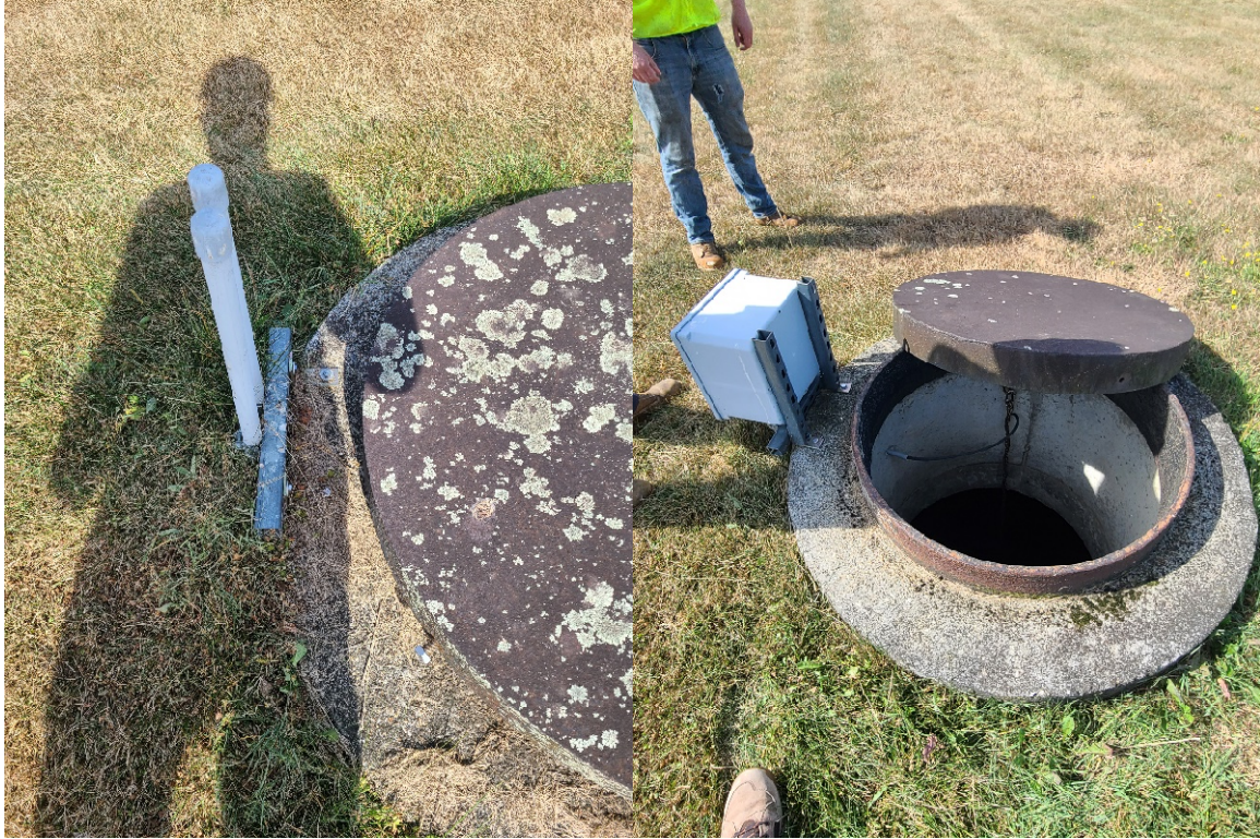
Access manholes on reservoirs with electrical conduit and junction boxes
