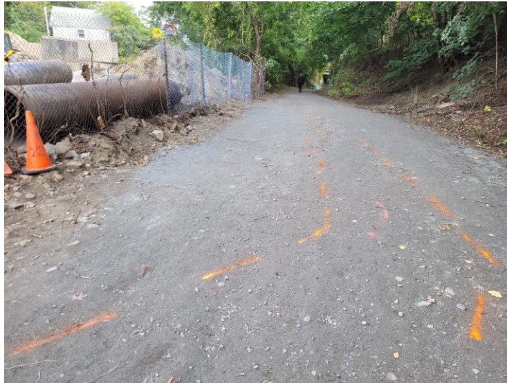
Figure 7: Photograph of Field markings- orange electric duct (facing north up eastern spur)
