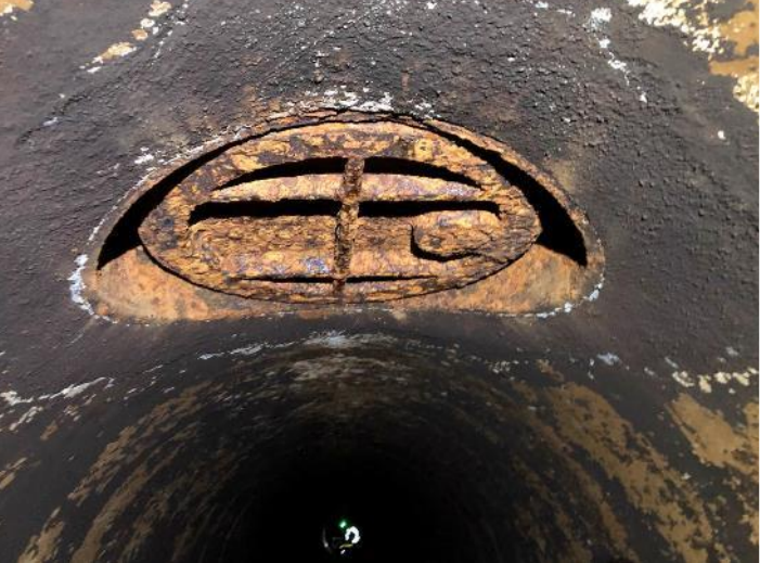
MH-7 (P6-68): Boiler Type
