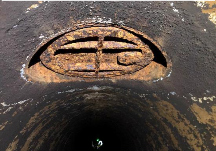
Manway 7: Boiler-Type, Corroded, Joints Old + Good
