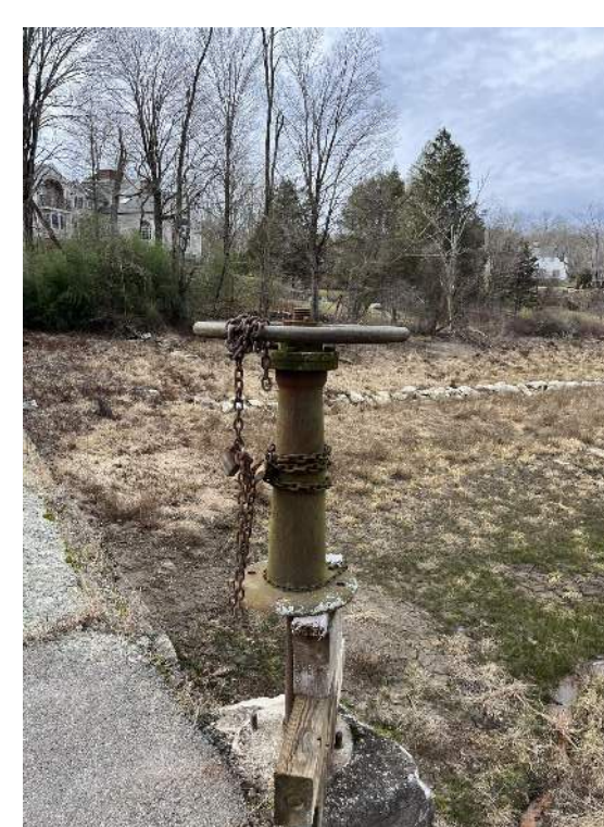
PHOTO 2 LOW-LEVEL OUTLET GATE OPERATOR
