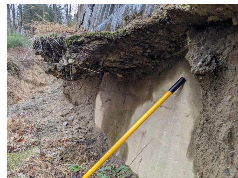
PHOTO 1 EROSION AT CONC. DAM DOWNSTREAM FACE
