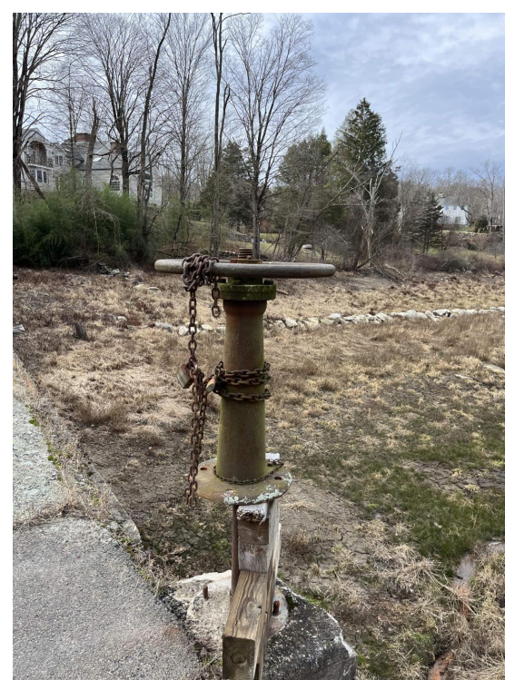
PHOTO 2 LOW-LEVEL OUTLET GATE OPERATOR
