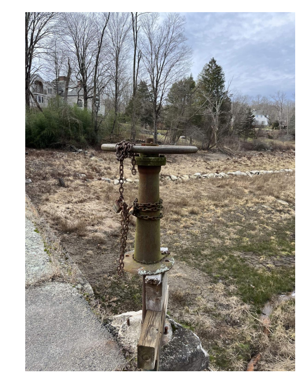
PHOTO 2 LOW-LEVEL OUTLET GATE OPERATOR
