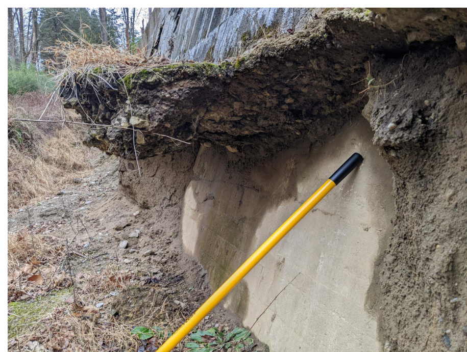
PHOTO 1 EROSION AT CONC. DAM DOWNSTREAM FACE
