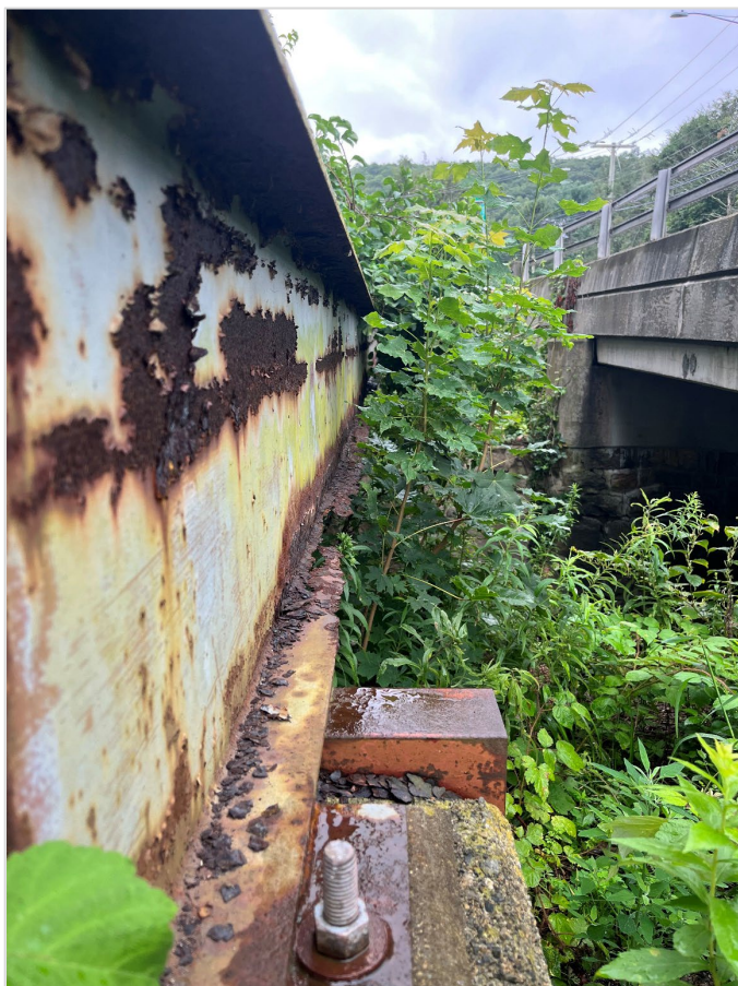
Photograph 6 – West side beam showing signs of section loss.
