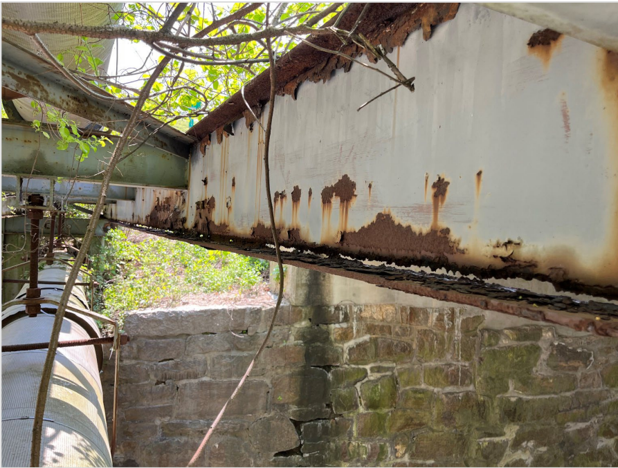
Photograph 7 – Section loss on west beam.
