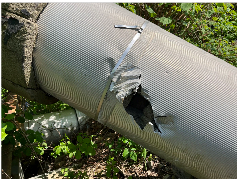
Photograph 10 – Damage to pipe insulation in isolated locations.
