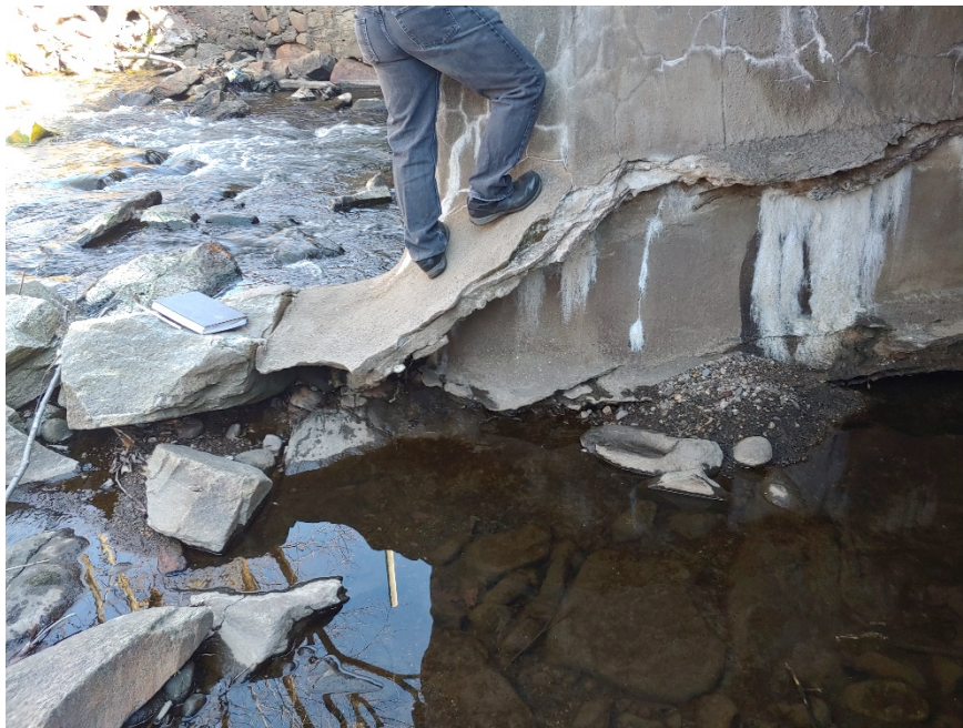
Photo 2: Photo of gunite remnants and footing of bridge on west side of bridge. West Side. Note person for scale.
