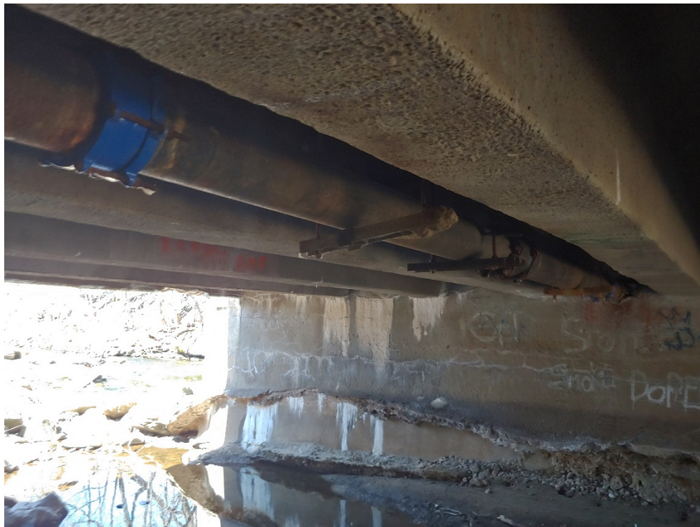
Photo 5: Underside of East Street bridge. Note uninsulated water main and gunite.
