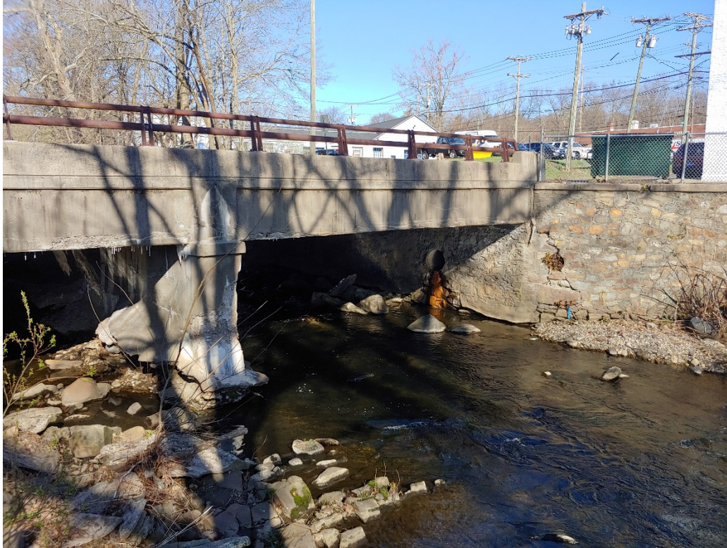
Photo 6: Gunite cover on East Street bridge. Note lead paint covered railing present in picture above parapet.
