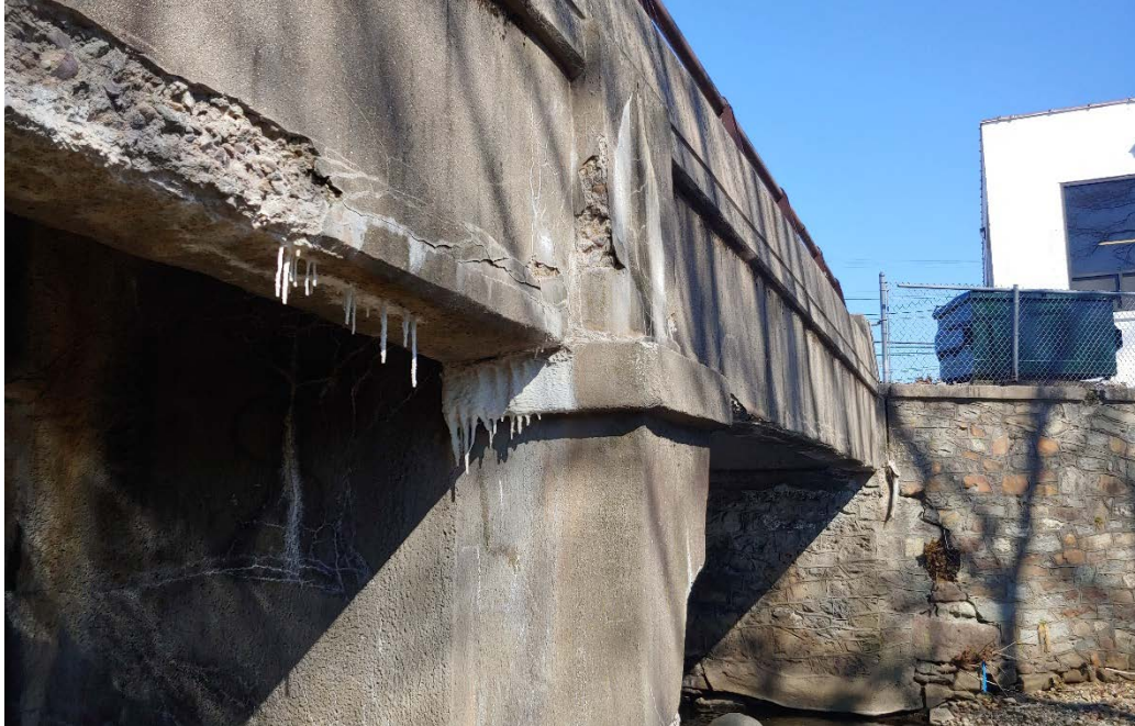
Photo 1: Photo of gunite applied to exterior of East Street Bridge (east side). Non ACM.
