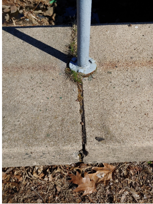
Photo 4: Wingwall railing and caulking. Caulking and paint found to contain lead.
