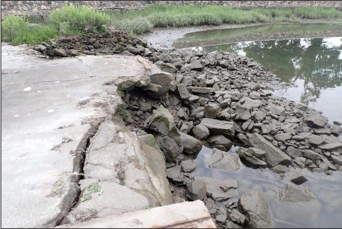
Photo 5: Erosion on left side of the dam
