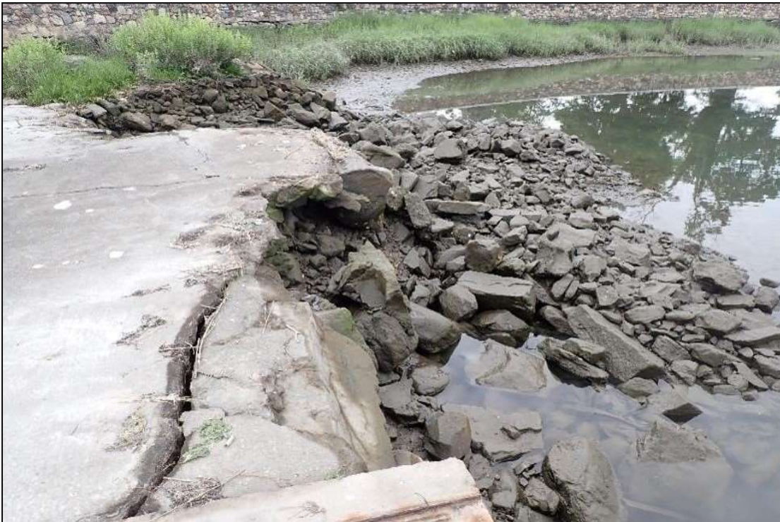
Photo 6: Crumbled Concrete Slab to Left of Fish Way
