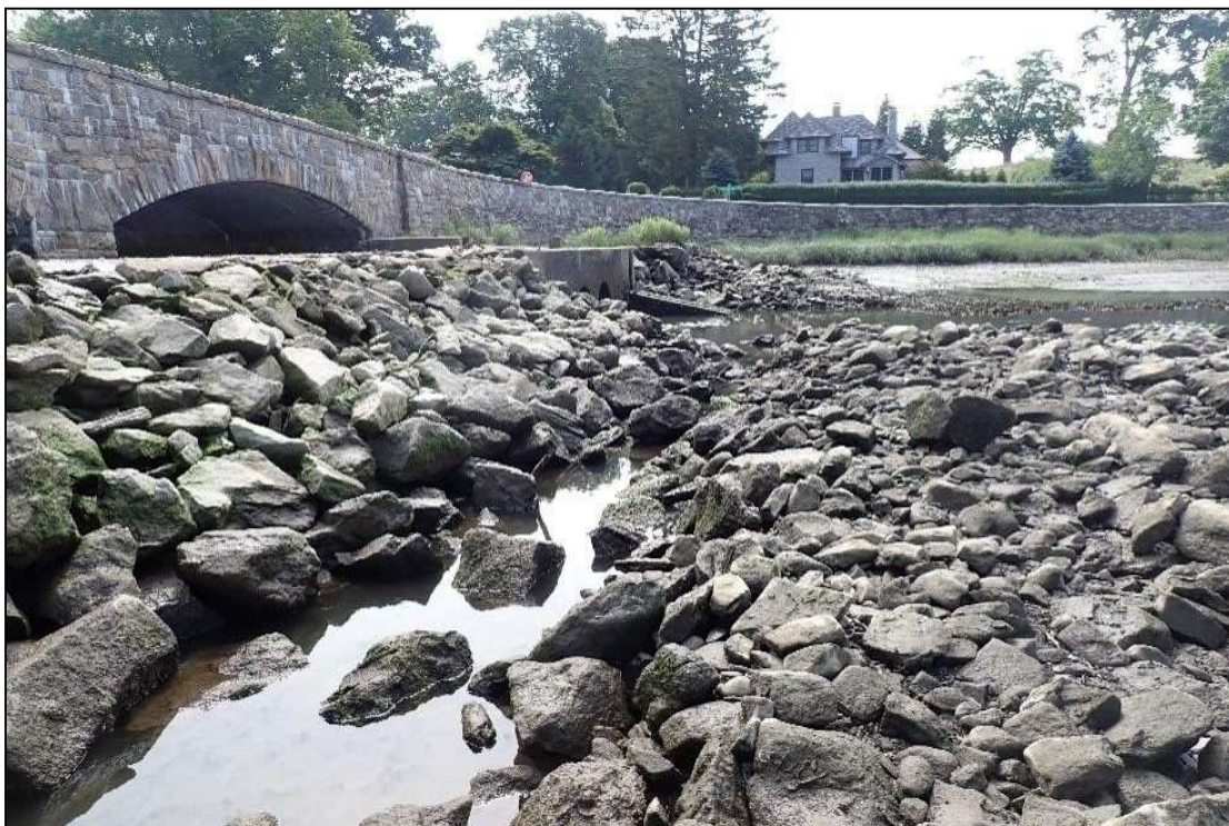
Photo 10: Overview of Scour Hole from Right Abutment
