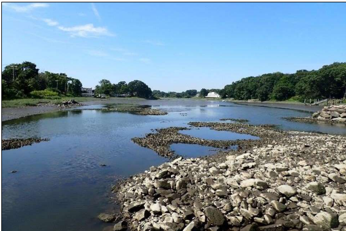
Photo 4: Eroded protective stone downstream of the dam, with shellfish bed beyond. Downstream channel on left.
