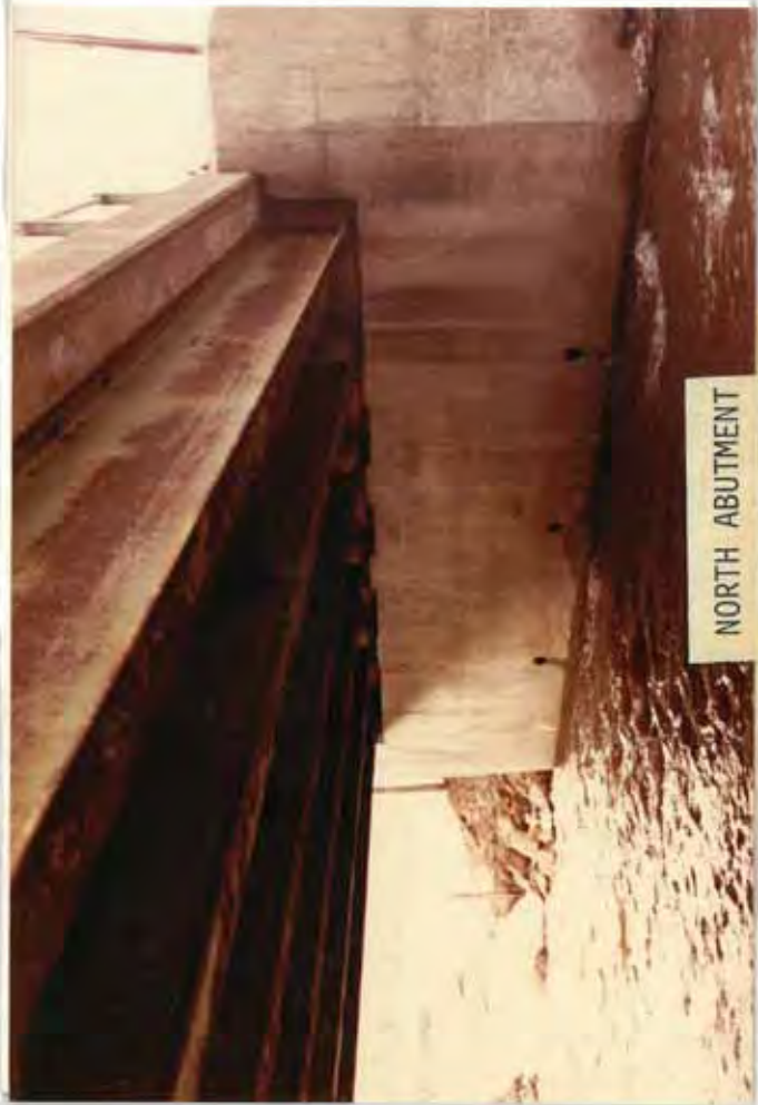
DAMAGED BRIDGE RAILING (WEST SIDE)
