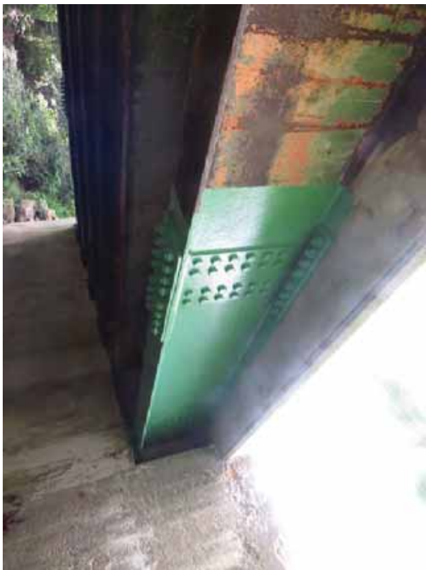
PHOTO 10: Beam 6, west elevation, new beam section and splice plates. Note this photo was taken from the 2017 Special Member Inspection Report.
