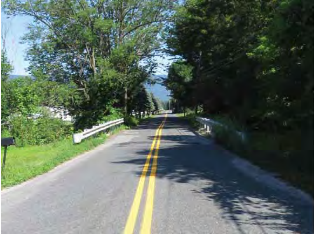
Photo 1: General topside view, looking north.
