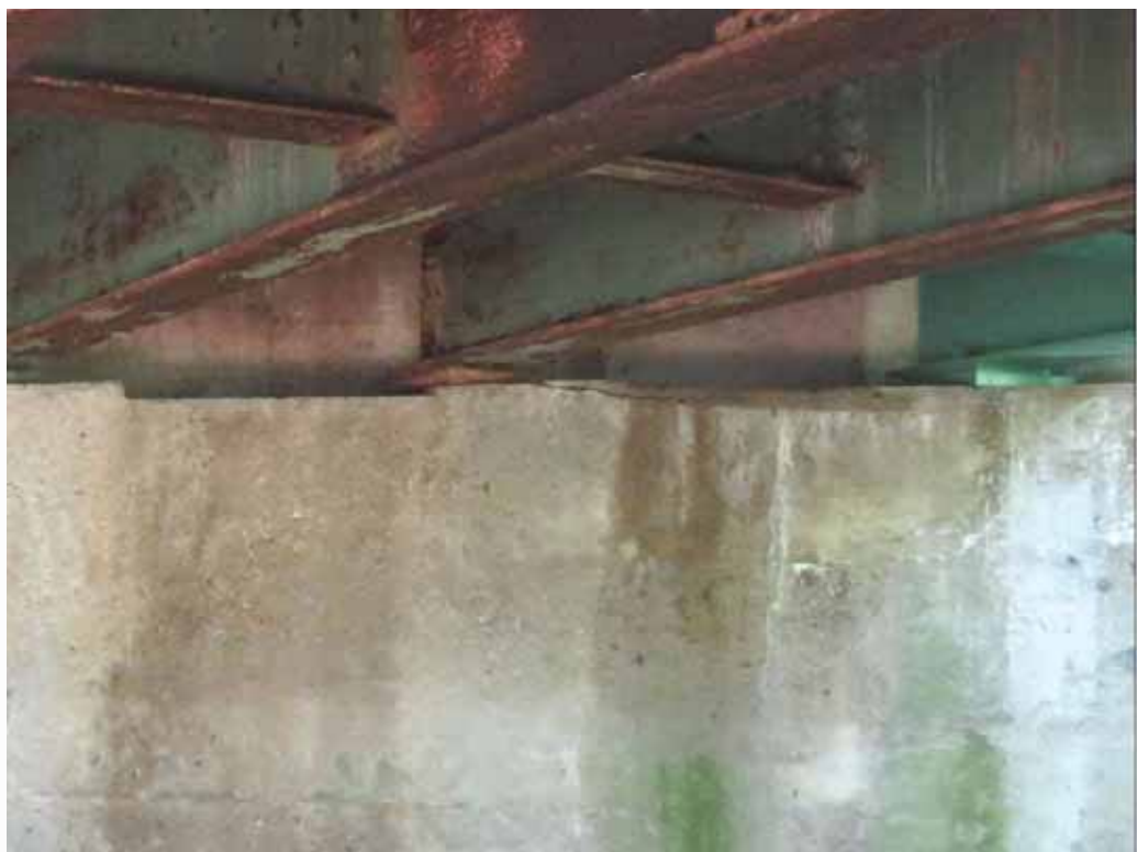
Photo 3: South breastwall. Horizontal crack with delamination through pedestal and upper breastwall in bay 5.
