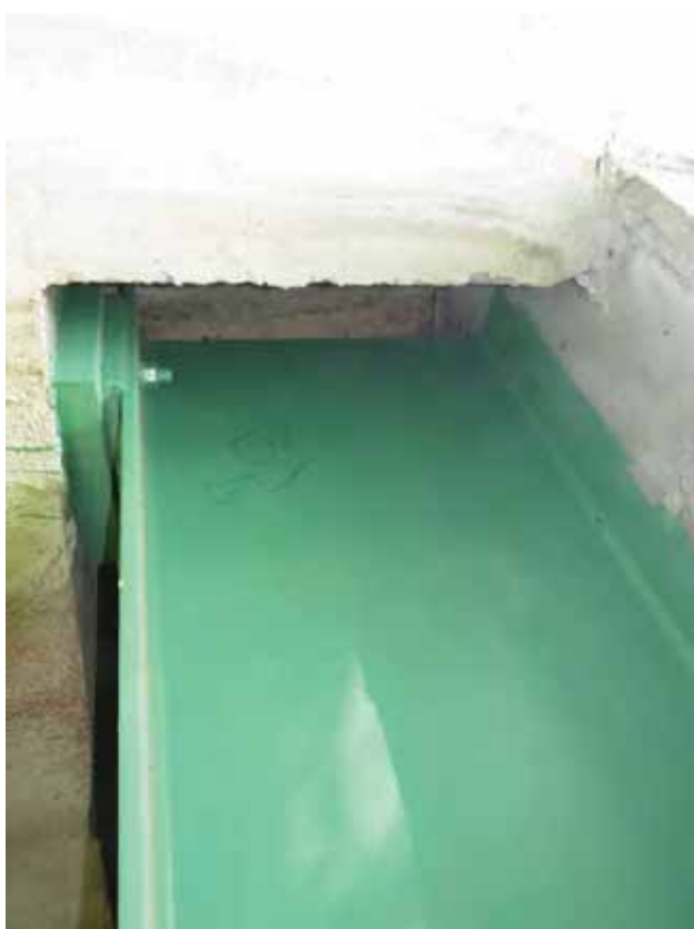
PHOTO 7: Typical bearing repair, beam 1, south end shown. Note this photo was taken from the 2017 Special Member Inspection Report.
