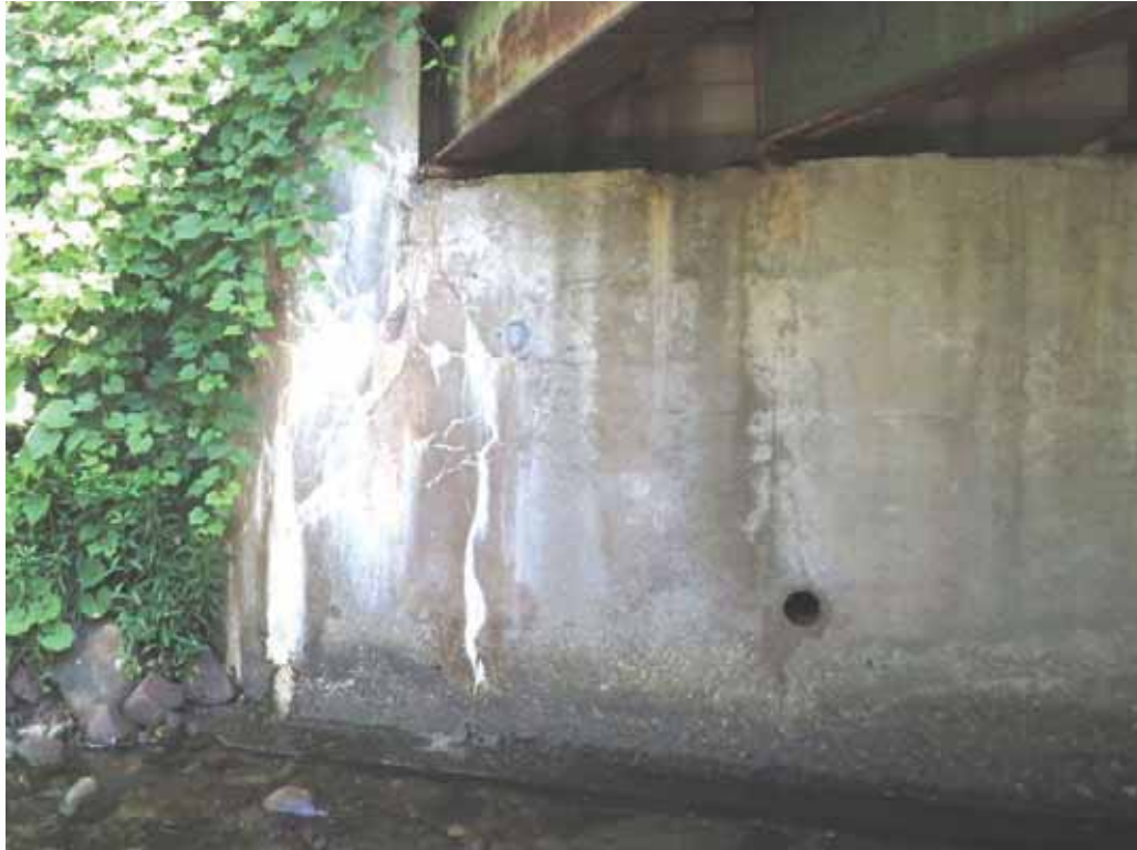
Photo 5: North abutment, west end. Scaling at upper breastwall/bridge seat under beams 5 & 6. Heavy cracking and efflorescence at interface with wingwall. Footing exposed.
