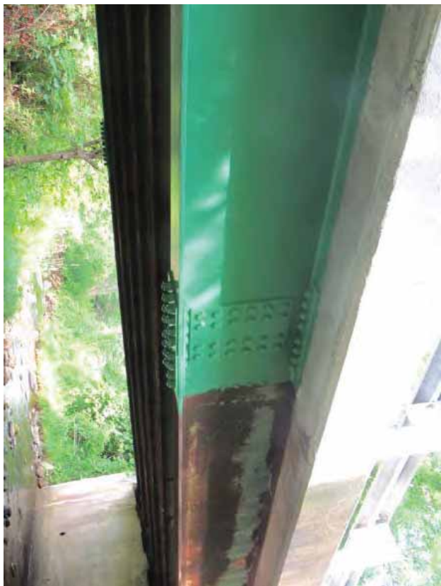
PHOTO 8: Beam 1, east elevation, new beam section and splice plates. Note this photo was taken from the 2017 Special Member Inspection Report.
