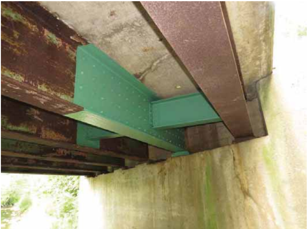
Photo 2: General underside and beam 2, north end repair plate and diaphragms.
