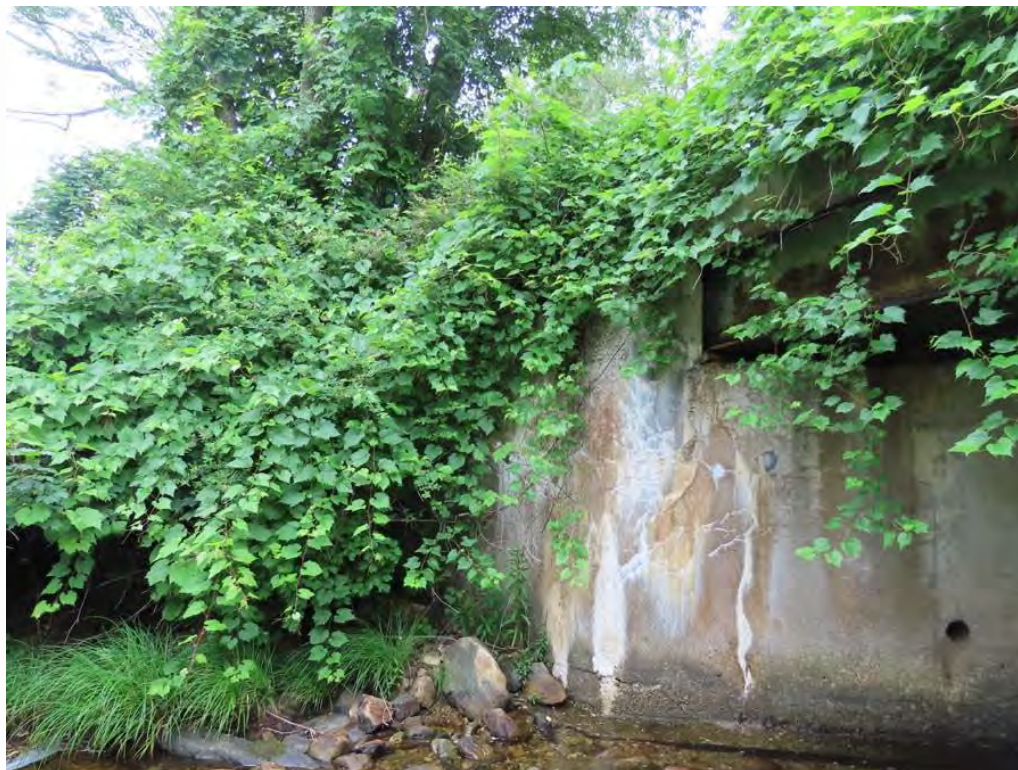
Photo 5: Northwest wingwall with cracking, scaling, and heavy vegetation growth.
