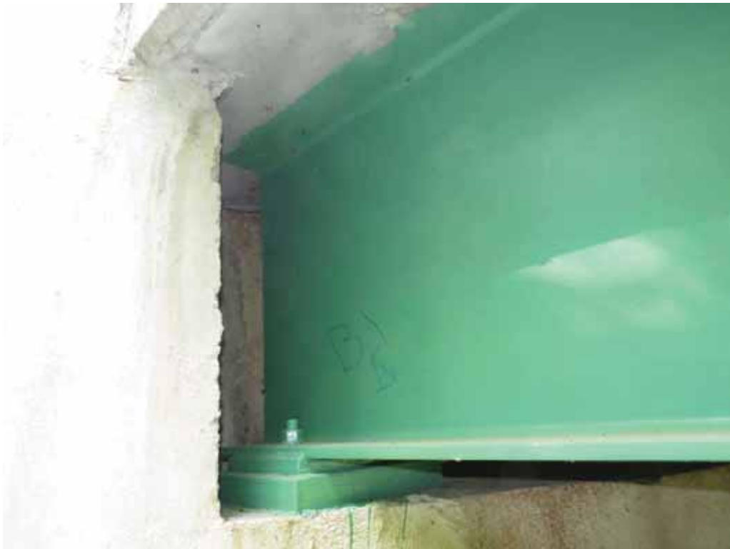
Photo 6: Typical bearing repair, beam 1, south end shown.
