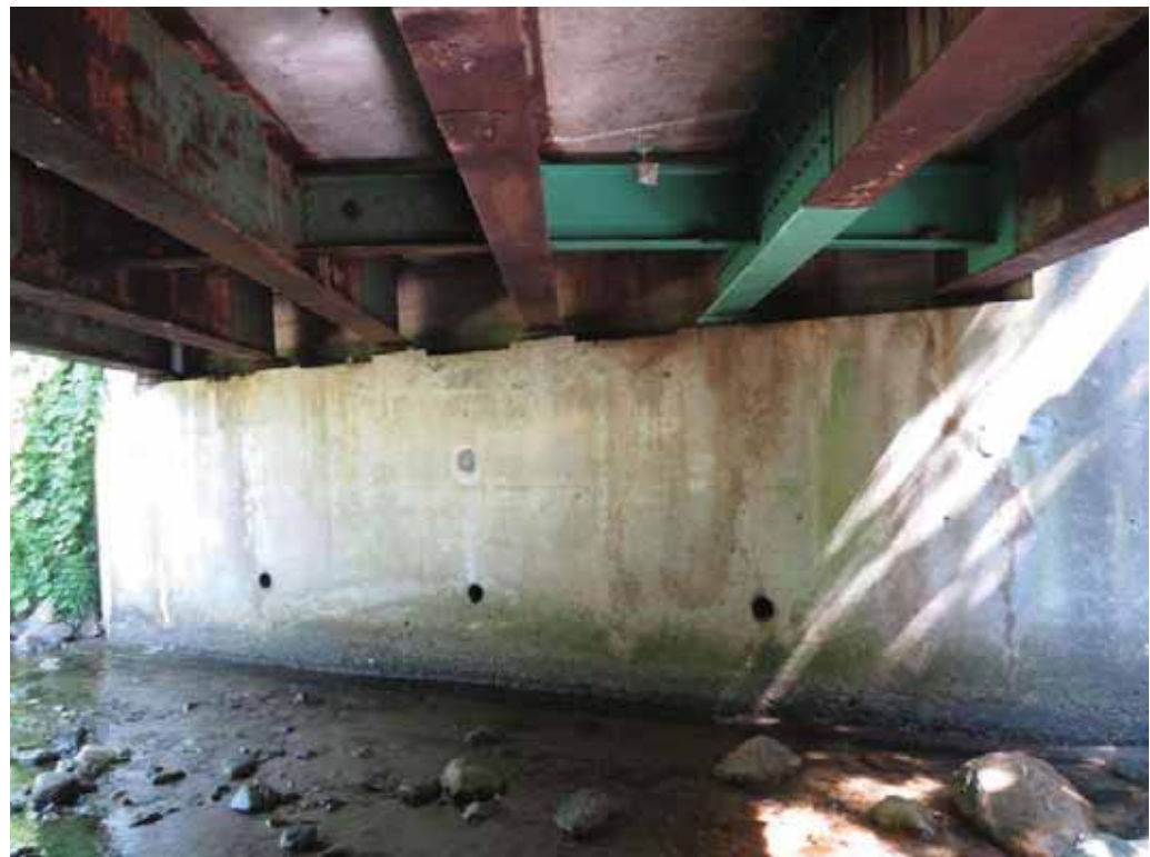
Photo 4: North breastwall has scattered map cracking, efflorescence, and scaling.
