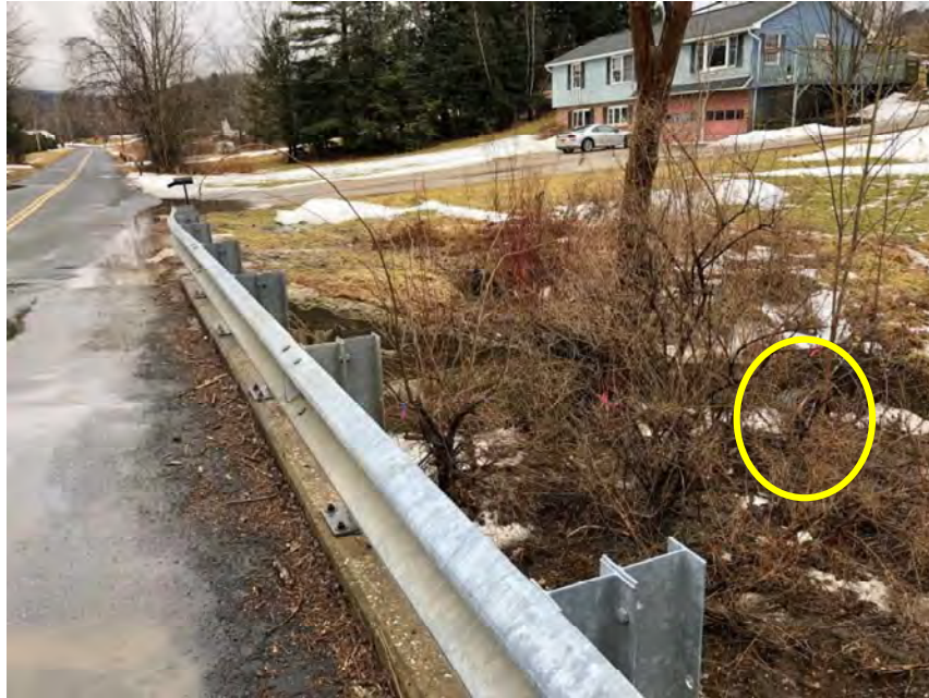
Photo 5 – View of the southwest wingwall and concrete headwall with drainage outfall (outlined) from the bridge deck.
