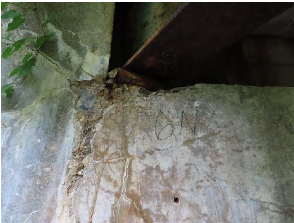
Photo 4: Scaling at the top of the north breastwall under beam 6. Note the undermining of the masonry plate.
