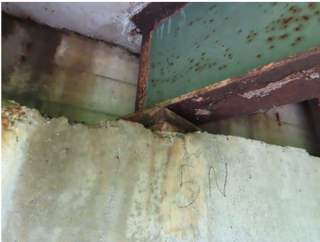
Photo 3: Scaling at the top of the north breastwall under beam 5.
