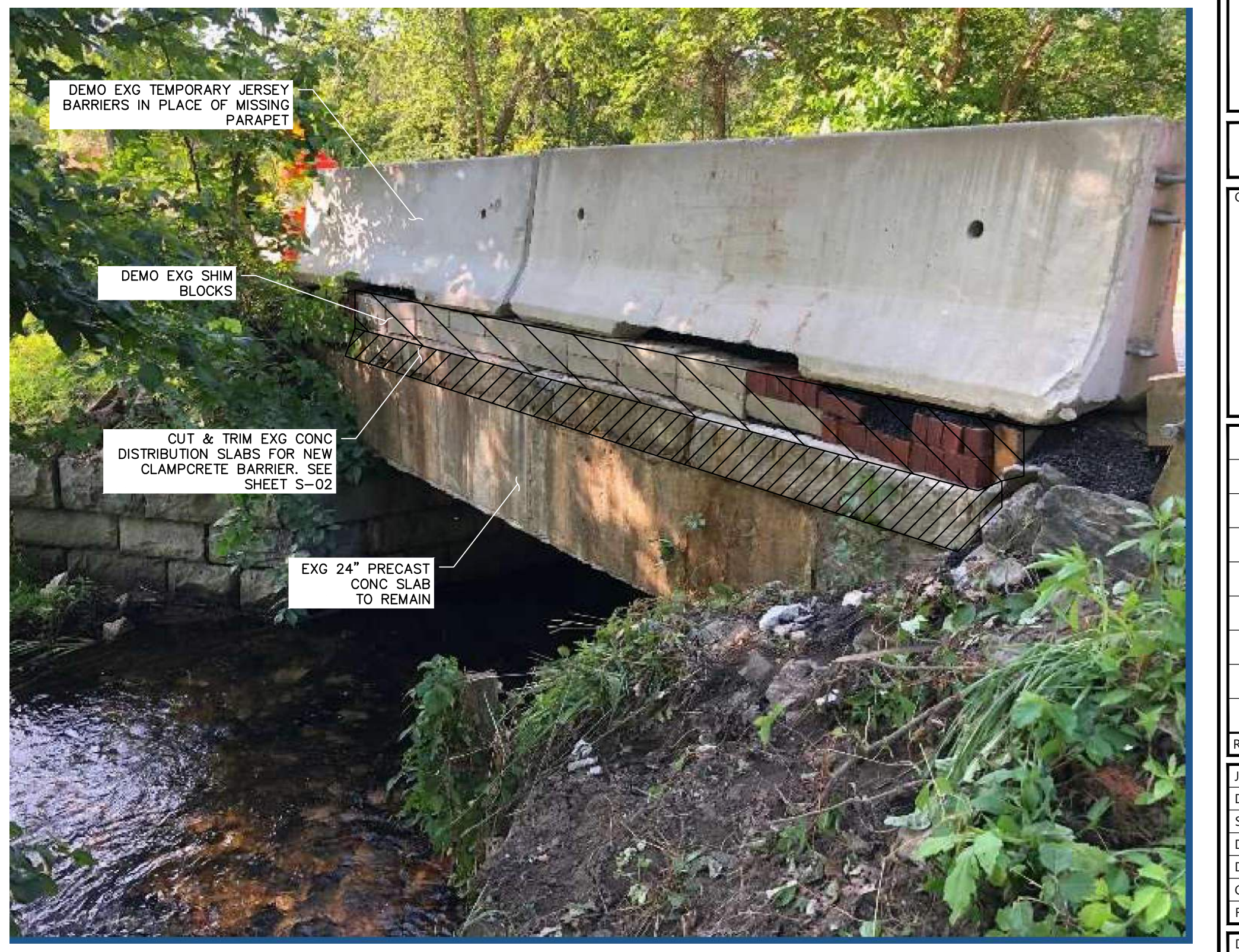
PHOTO 2: EXISTING CONDITIONS - MISSING PARAPET
