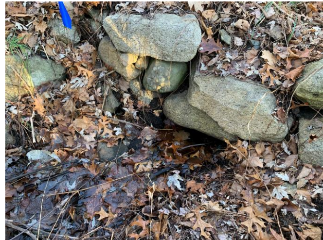
Photograph 2 – Stone headwall Culvert #110 outlet
