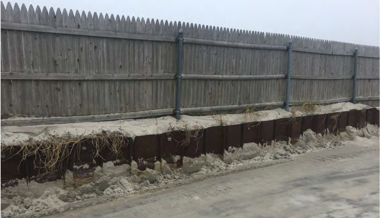
Photo No. 1: Typical view of existing steel sheet pile bulkhead with wooden fence above
