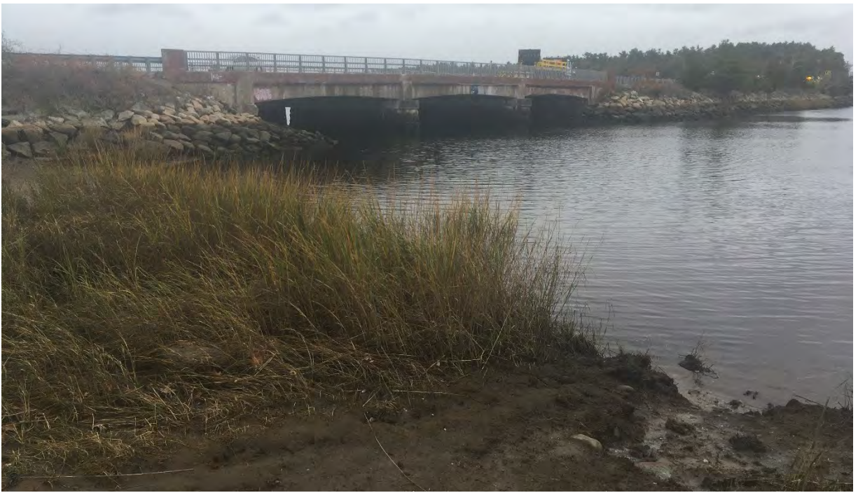
Photo #3: View south from Wareham salt marsh on northwest side of crossing (upstream) to the project area and Bridge # W-06-016.
