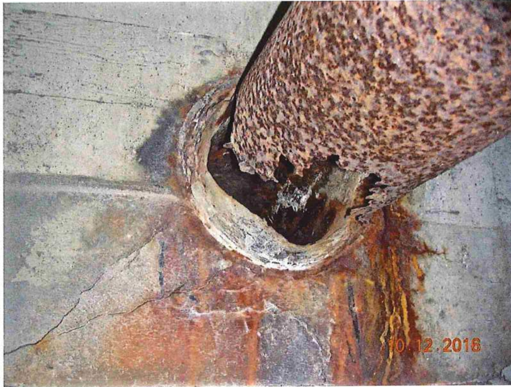
Photo 13: Tee Bay 5 at west abutment, area of 100% section loss to unused utility conduit
