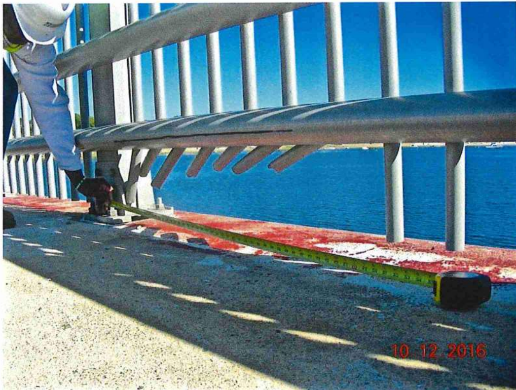
Photo 10: South rail 6th section from east abutment, bent lower sections of pickets
