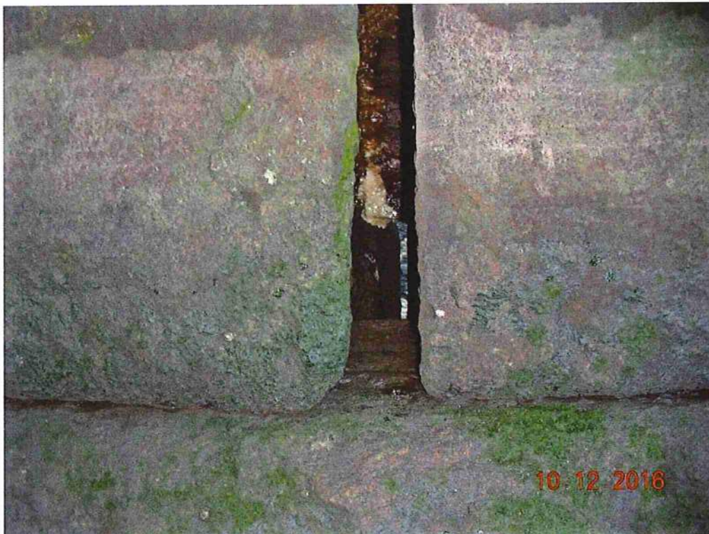
Photo 30: Northeast end of pier wall, void clear through second course
