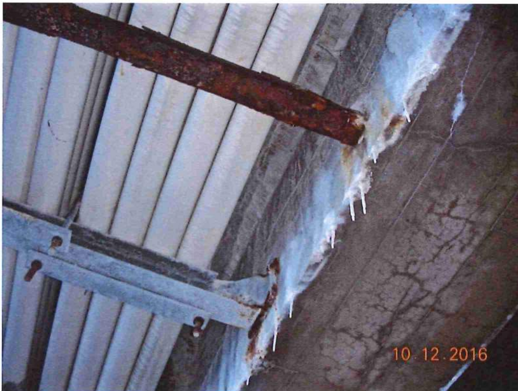
Photo 12: Span 1 Tee Bay 1, corrosion to utility support
