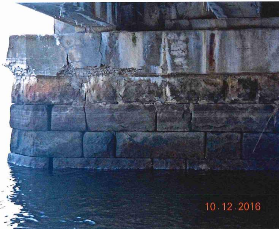
Photo 26: Northwest end of pier, cap spalling & cracked stones in wall
