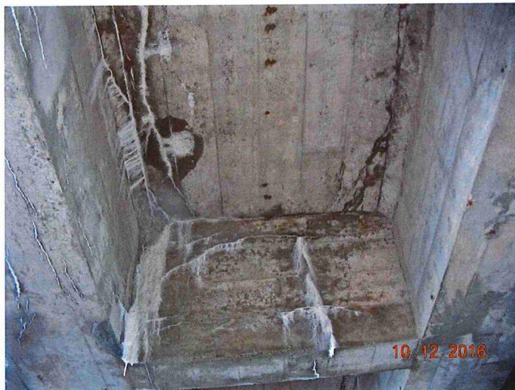
Photo 6: Span 2 Tee Bay 2 looking east, typical cracking w/ efflo
