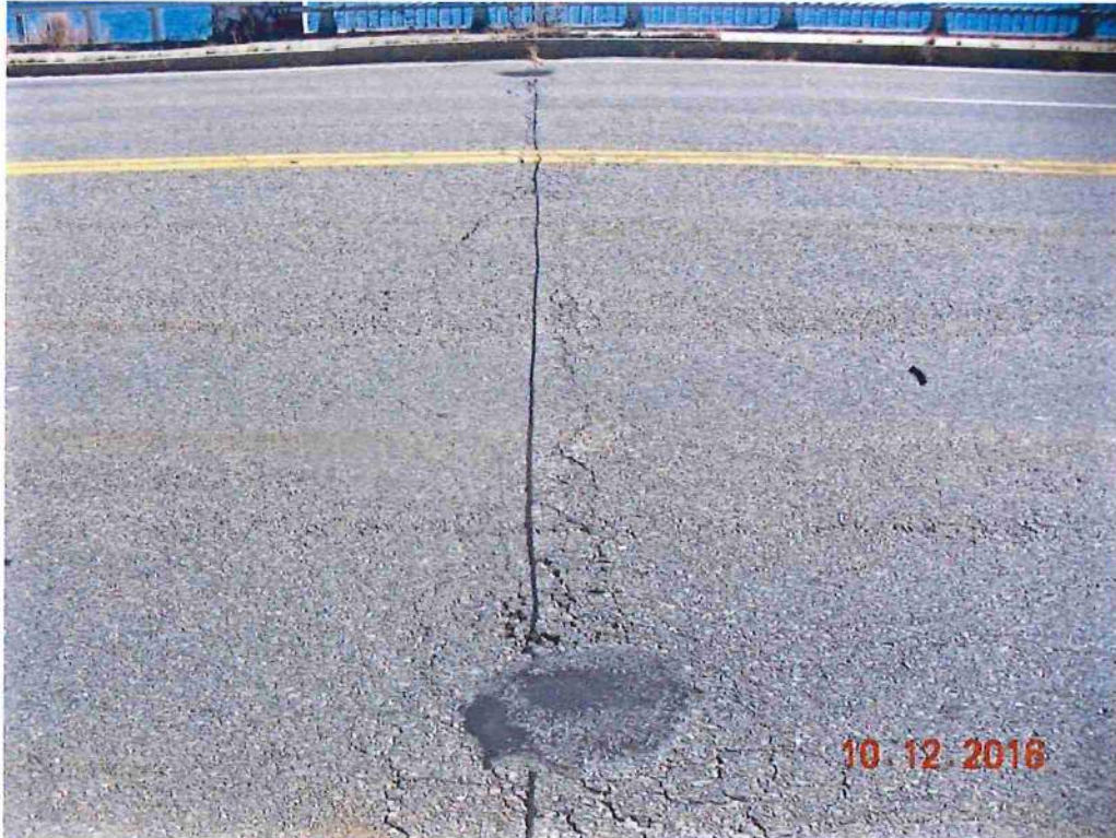
Photo 3: Over east abutment looking south, minor rutting in travel lanes & 2 settled patches in each right lane
