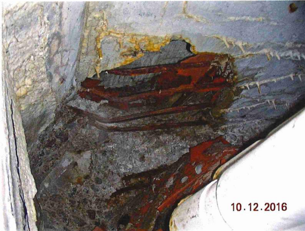
Photo 9: North sidewalk soffit at east abutment, heavy spalling w/ exposed rebar & void
