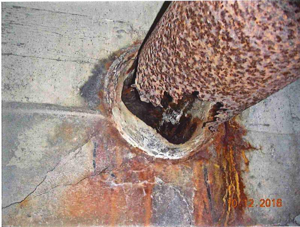
Photo 13: Tee Bay 5 at west abutment, area of 100% section loss to unused utility conduit
