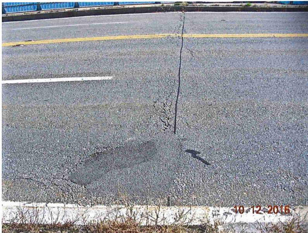
Photo 2: Over west abutment looking south, rutting in travel lanes & settled patch in WB right lane
