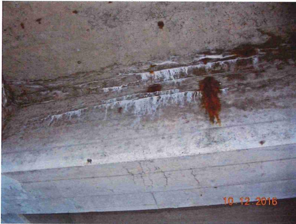
Photo 15: Span 1 Tee Beam 2 north face, horizontal cracking w/ efflo & rust bleed
