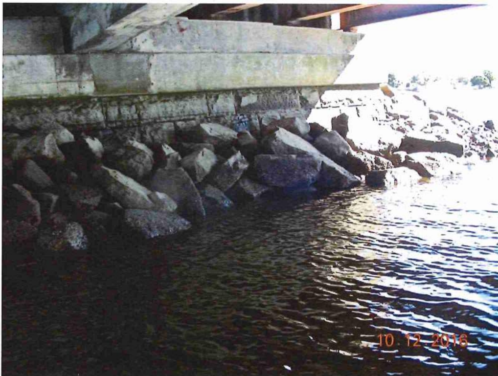
Photo 32: East abutment rip-rap south end, slumped & missing stones
