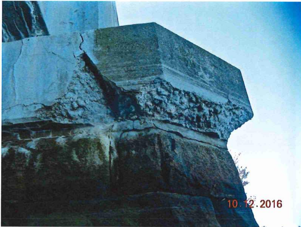
Photo 31: Northeast nose of pier cap, spalling
