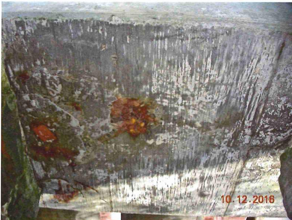
Photo 28: Pier cap soffit below Steel Bay 1, cover spalls w/ rust bleed
