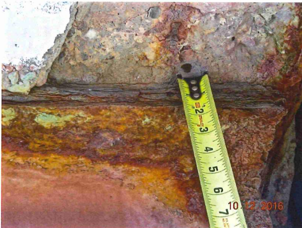
Photo 20: Span 2 Steel Beam 4 at east abutment, south top flange pack rust
