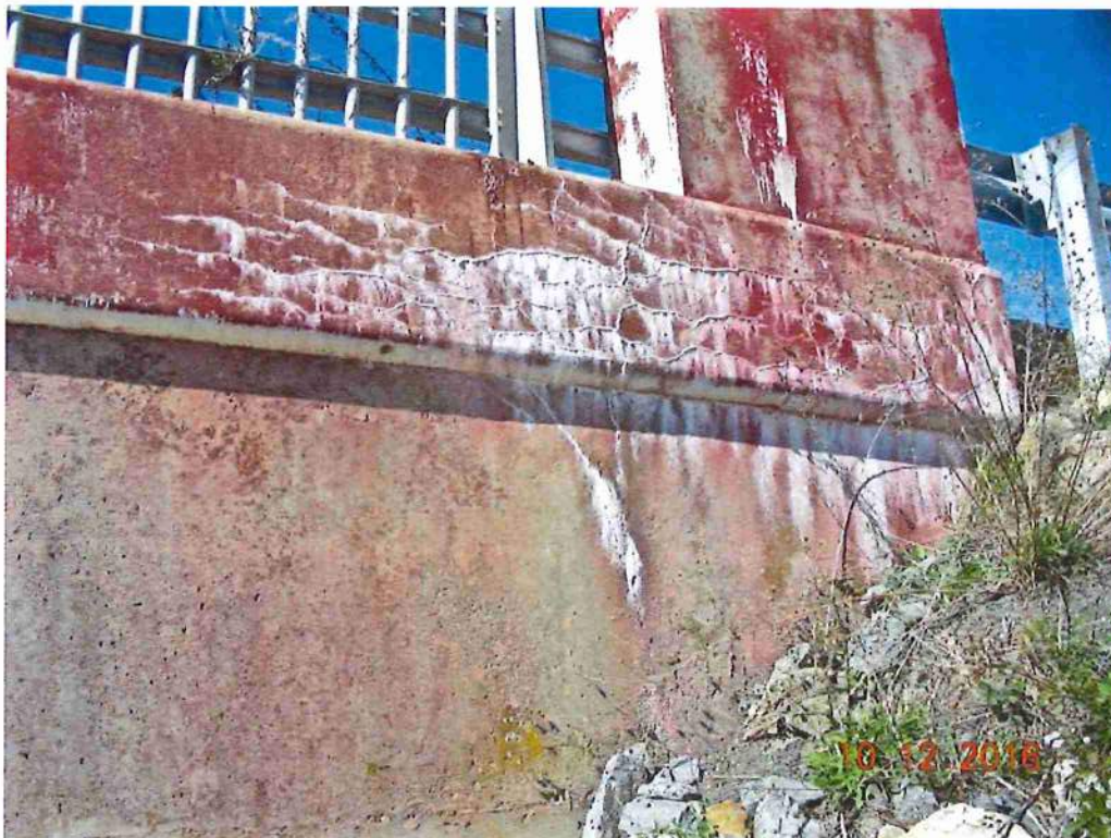
Photo 24: Southeast wingwall, horizontal cracking w/ efflo
