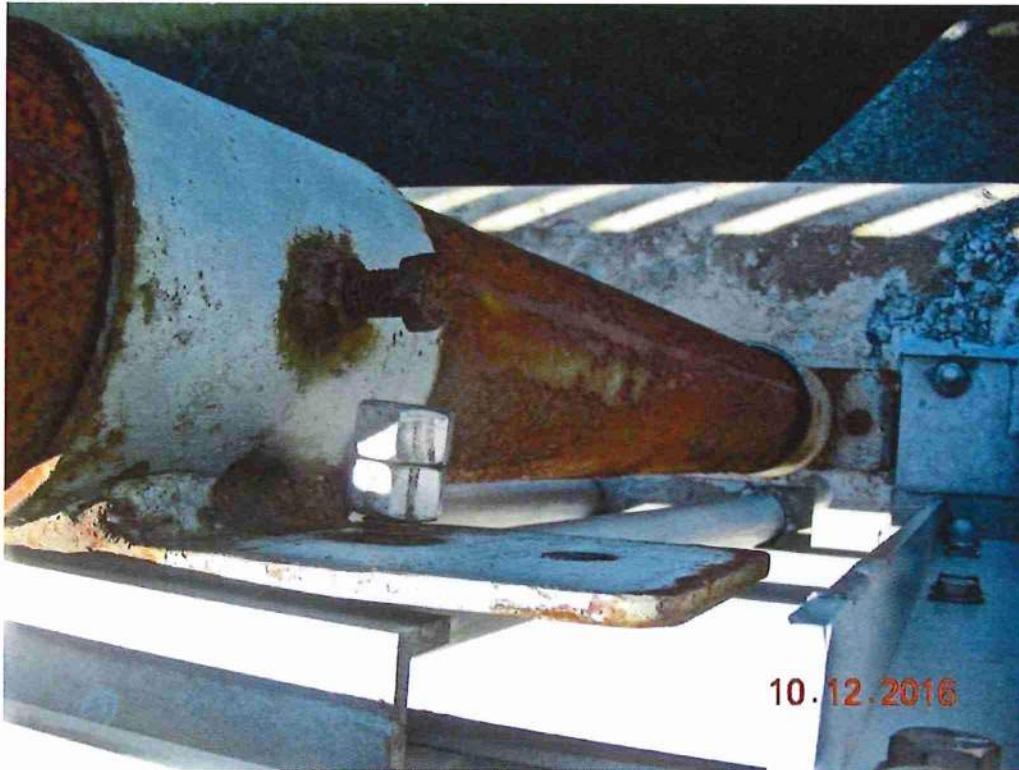
Photo 11: Town line sign attached to north rail at midspan, loose fasteners & small areas of 100% section loss at base
