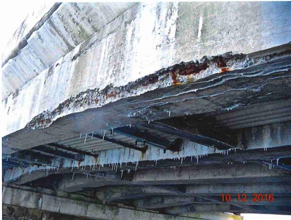
Photo 14: Span 1 Tee Beam 1 looking east, spalling w/ exposed rebar
