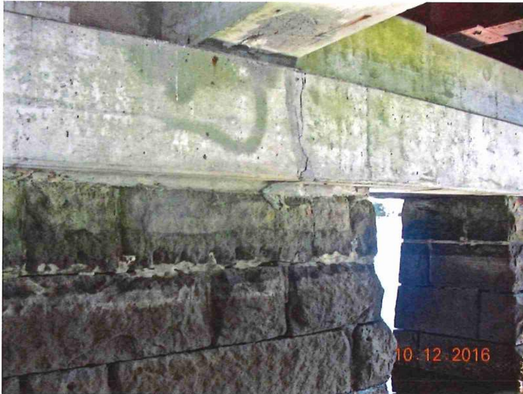
Photo 27: Pier cap west face below Tee Beam 6, vertical crack
