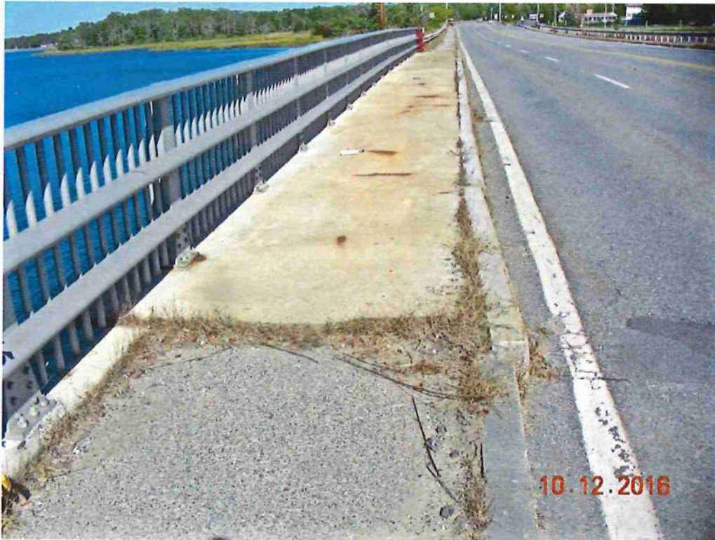
Photo 7: North sidewalk looking east, curb displaced towards roadway & approach sidewalk/curb settlement
