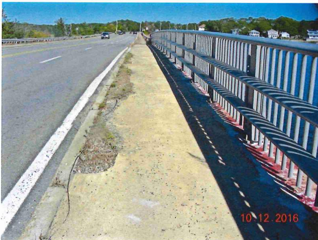
Photo 8: South sidewalk looking east, debris impacted scaling/spalling along curb
