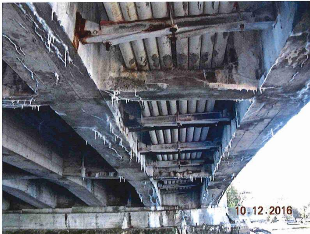
Photo 18: Span 2 Tee Beams 1 & 2 looking west, longitudinal cracking w/ efflo
