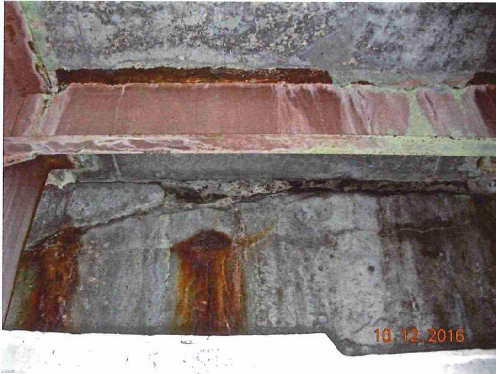
Photo 23: Steel Bay 1 at east abutment, backwall spalling/cracking w/ rust bleed
