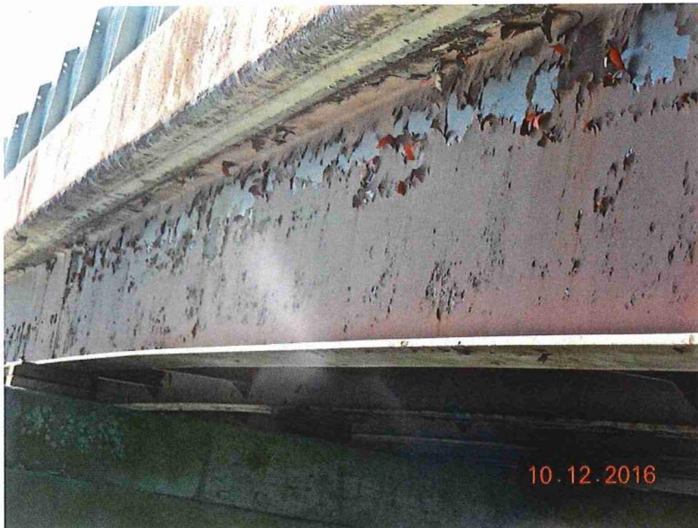
Photo 22: Span 2 Steel beam 4 looking west, paint failure
