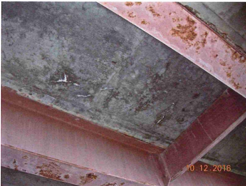
Photo 4: Span 1 Steel Bay 2 looking east, typical minor cracking w/ efflo
