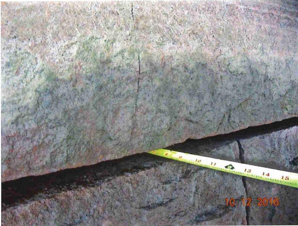
Photo 29: Pier wall east face below Steel Bay 3, vertical crack in top course stone & missing mortar
