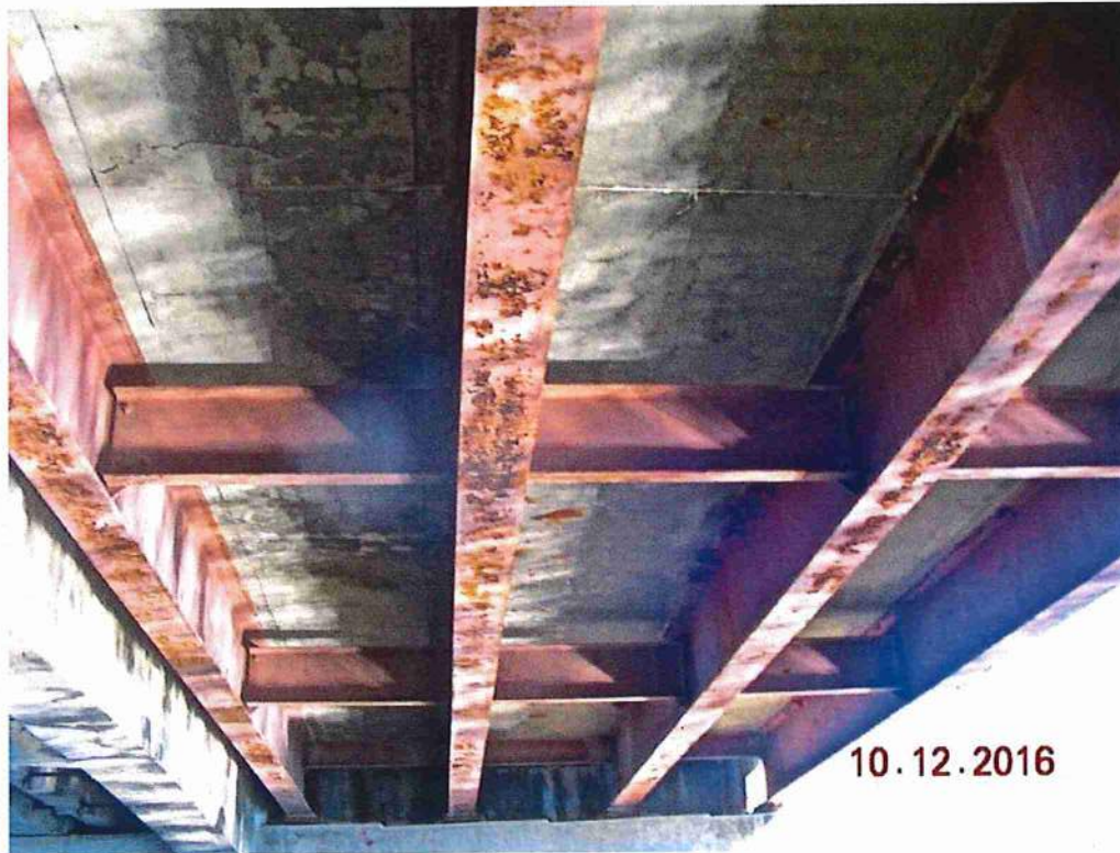
Photo 5: Span 2 Steel beam bays looking east, minor delams/cracking & corrosion to bottom flanges
