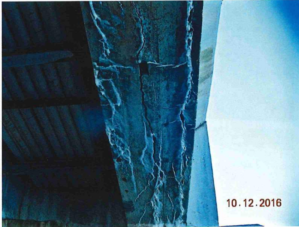
Photo 17: Span 2 Tee Beam 1 looking west, longitudinal cracking w/ efflo
