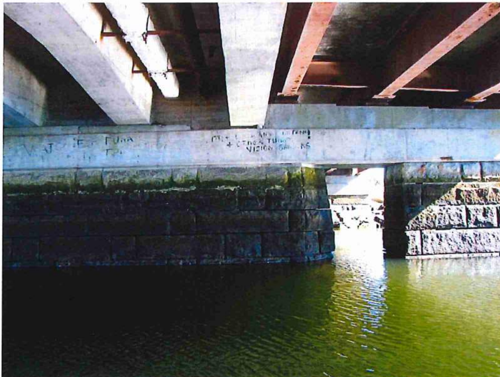
Photo 56: Overview of pier 2 and south widening pier (L to R), west face. Missing pointing
