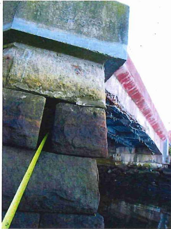
Photo 59: Close up of previous photo. Gap up to several inches wide
