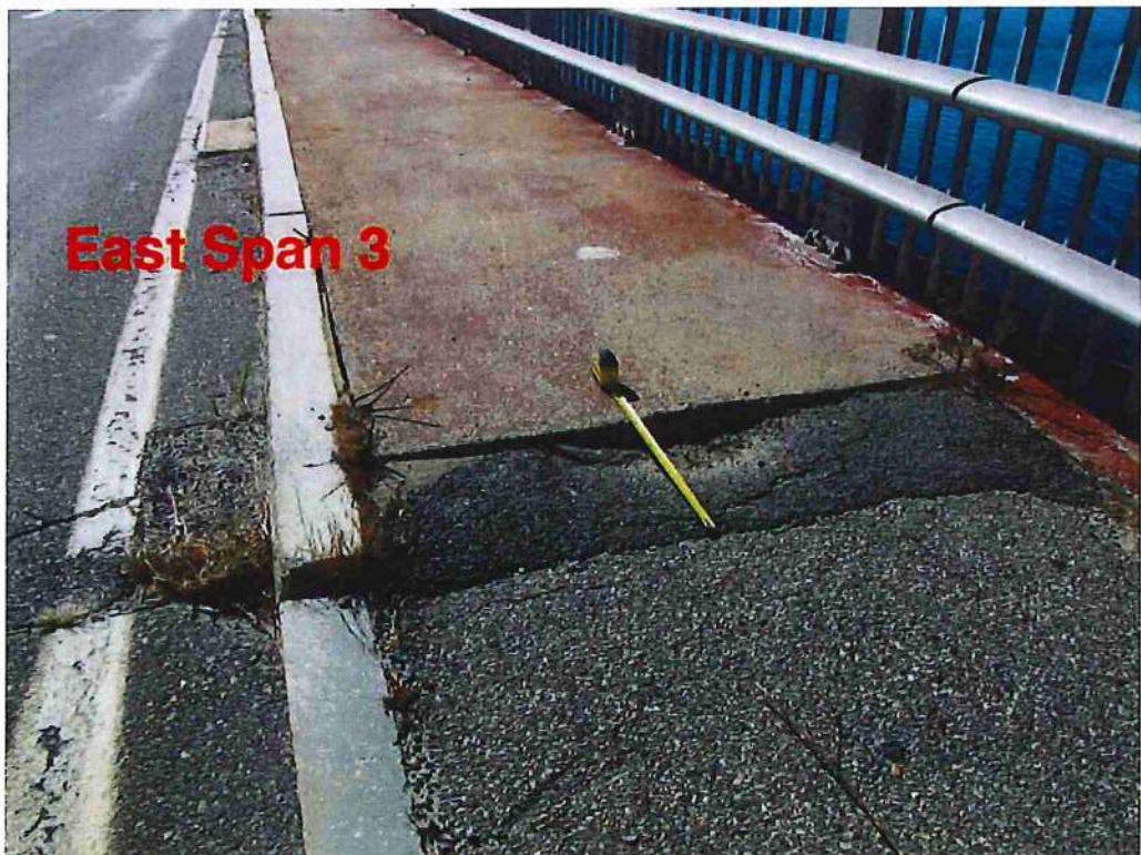
Photo 10: Overview of north wearing surface and sidewalk looking west. Approach sidewalk settlement up to 3" at middle. Previous concrete and asphalt patches in gutter
