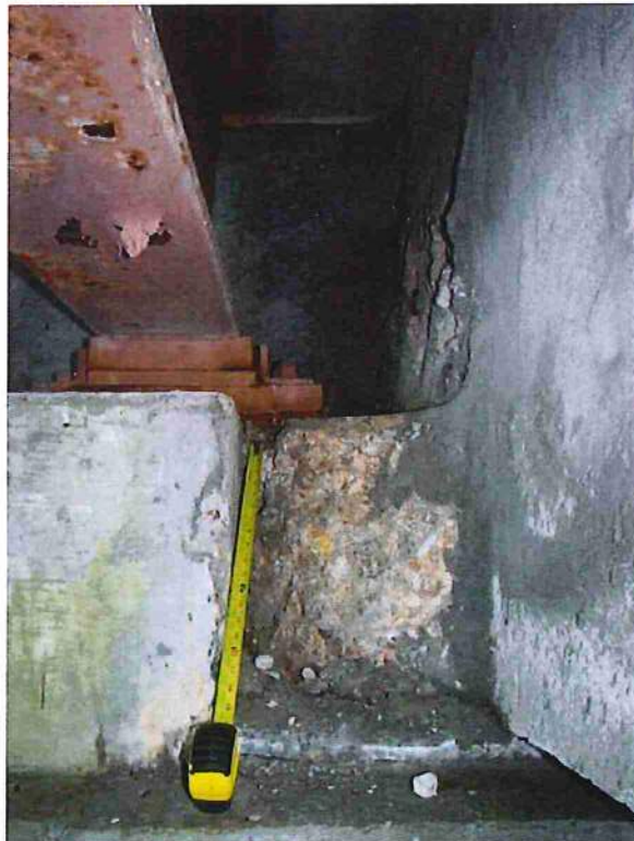
Photo 48: West abutment, at BM1 (South extension). Spall extends back to masonry plate
