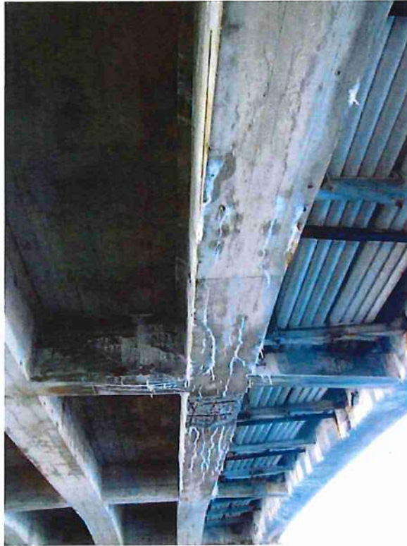
Photo 17: Span 2, bays 2 and 1 (L to R) looking west. Previous deck patch in foreground of bay 2
