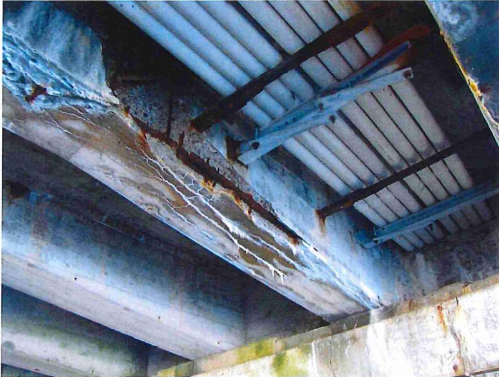
Photo 45: Span 3, BM 2 near pier 2, full height spall with exposed and debonded rebar at bottom edge
