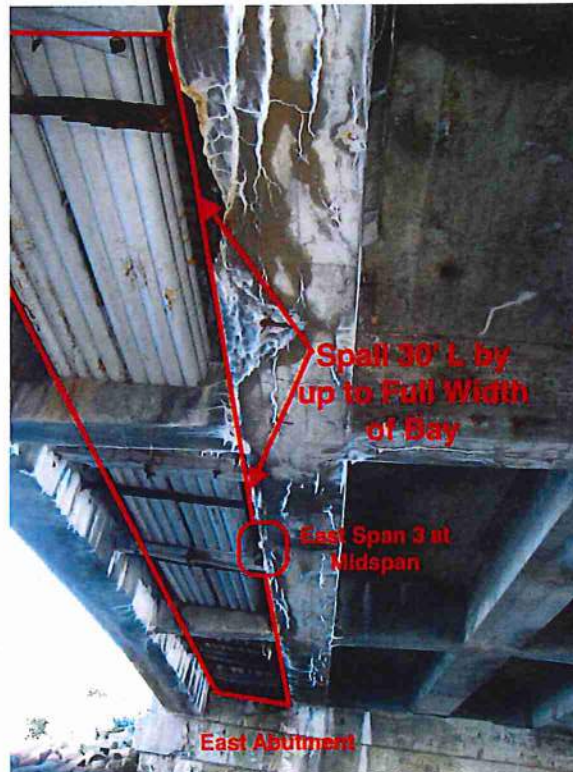
Photo 13: Underside of previous photos 10, 11 and 12 looking east. Span 3, bay 1, spall extending from midspan to east abutment
