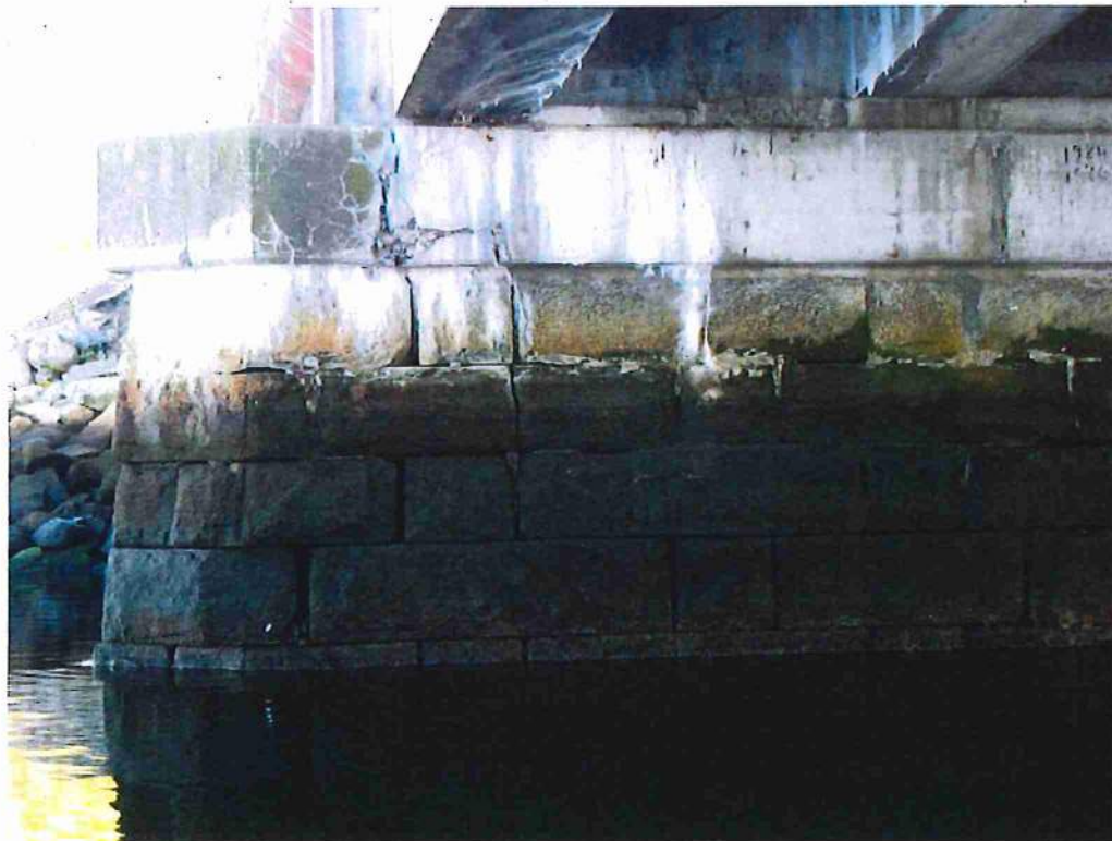
Photo 54: Overview of pier 2, NW. Vertical cracks in cap and into blocks below. Missing pointing
