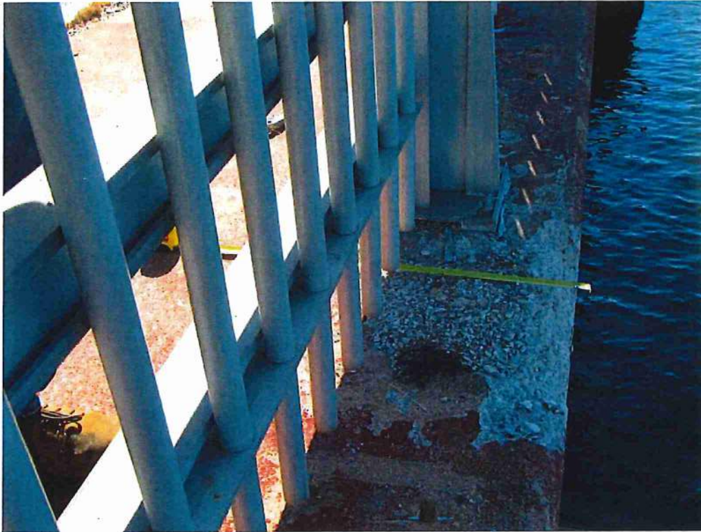
Photo 33: North sidewalk, span 3 north edge spall/scale
