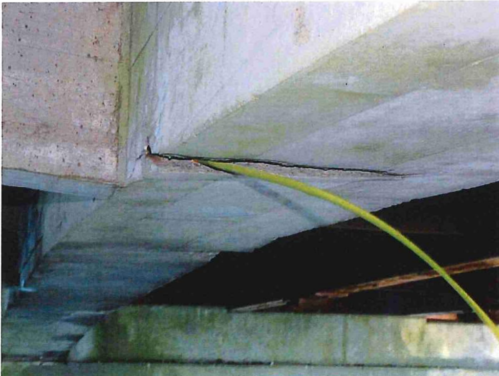
Photo 40: Span 1, BM 6 at midspan. spall with adjacent delam
