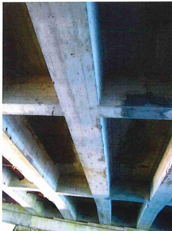
Photo 18: Span 2, bays 5, 4, and 3 (L to R) looking west. Previous deck patches in bays 4 and 3
