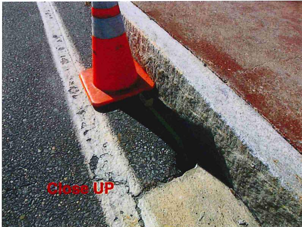
Photo 12: Close up of previous photo. Through hole to underside
