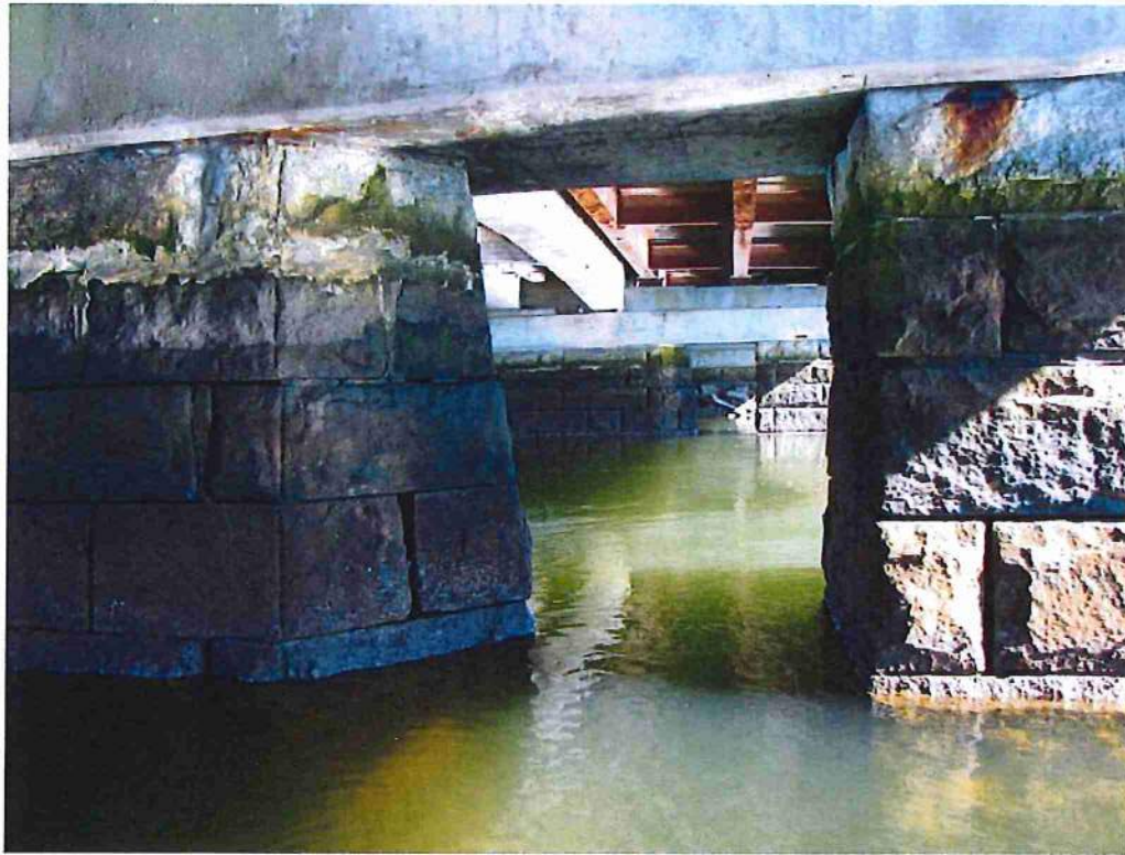
Photo 61: Pier 1 and south extension pier, west face. Missing pointing
