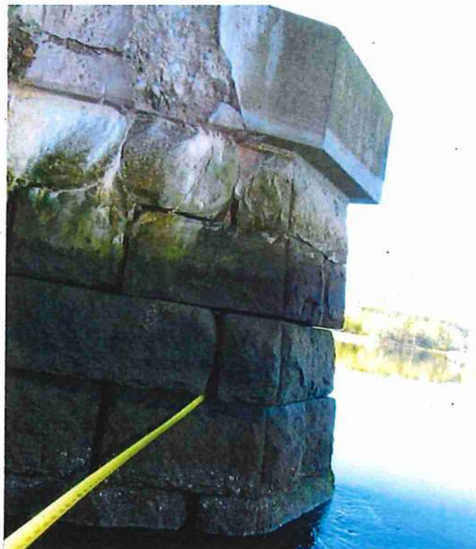
Photo 60: Pier 1, NE face - Typical of missing mortar and pointing
