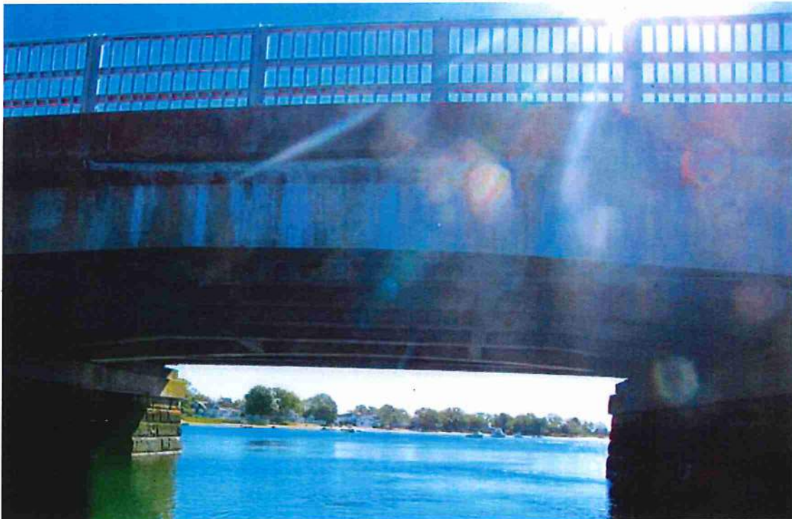
Photo 30: Span 2 north face spall
