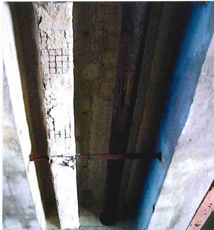
Photo 34: Span 2, bay 5 utilities. Utility pipe on right with holes, apparently abandoned
