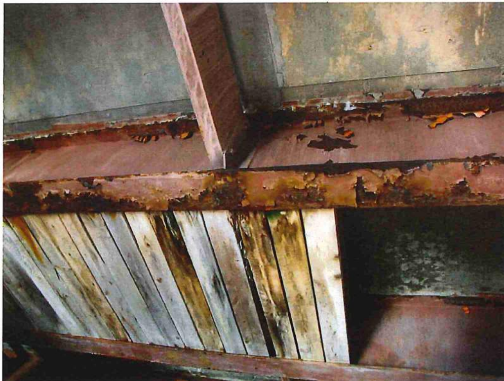
Photo 28: Similar to previous photo. Beam 3 with active corrosion along bottom flange
