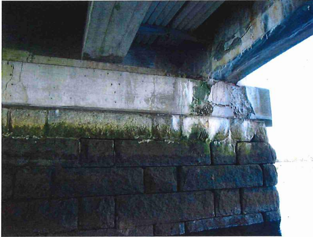
Photo 53: Close up of previous photo at NE end of pier. Missing pointing
