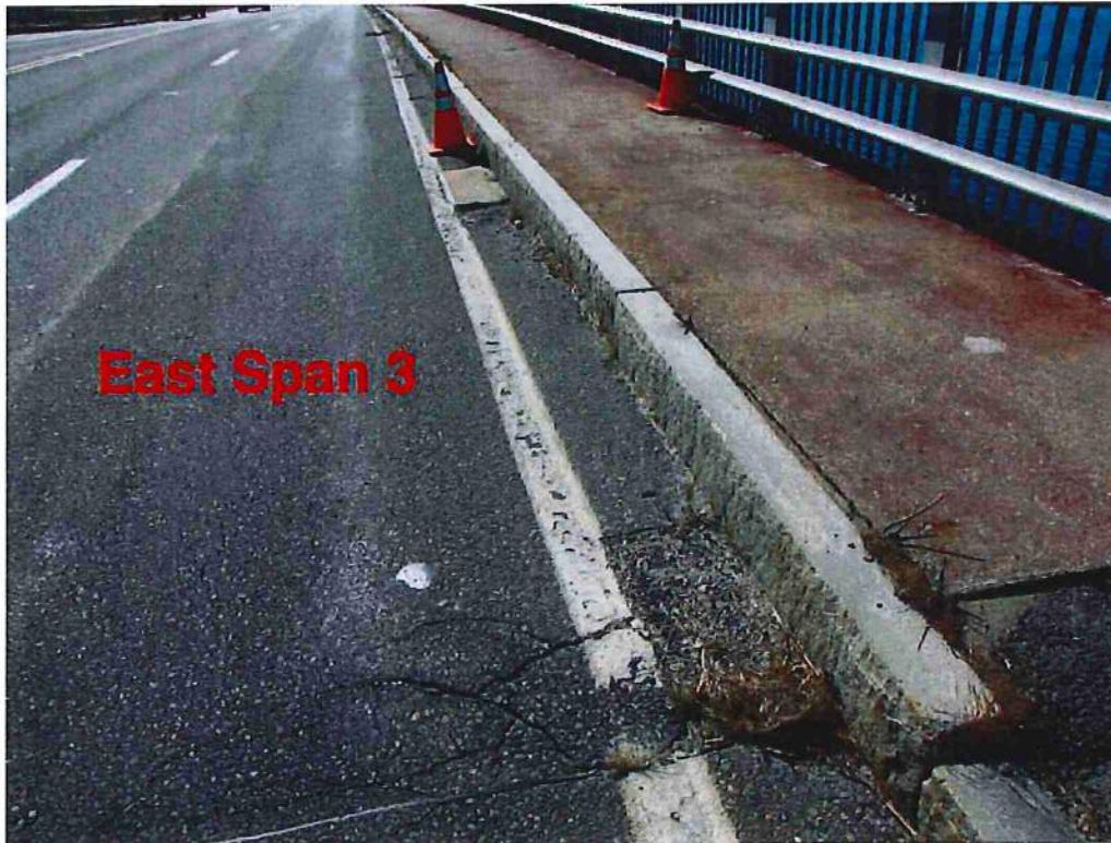
Photo 11: Similar to previous photo. Previous concrete and asphalt patches in gutter line
