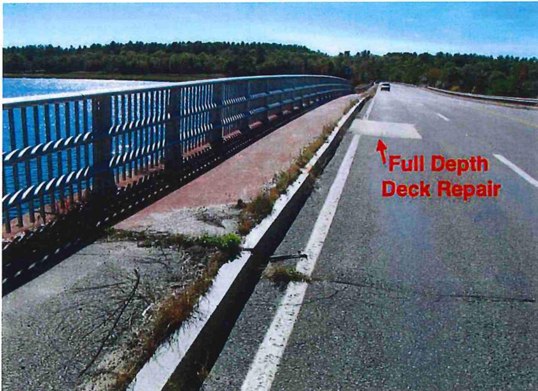
Photo 2: Overview of south wearing surface and sidewalk looking west. Previous full depth deck repair in span 3, bay 2.
