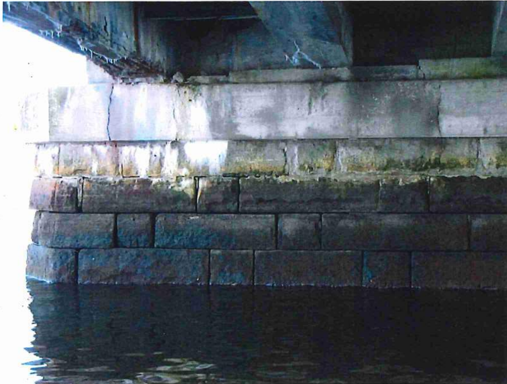
Photo 51: Overview of pier 1, NW. Vertical cracks in cap. Missing pointing
