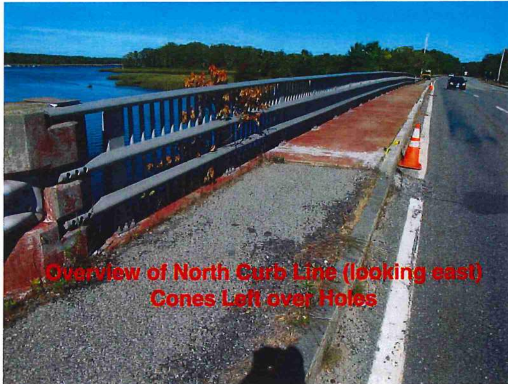
Photo 3: Overview of north wearing surface and sidewalk looking east. Cones are located at holes in wearing surface
