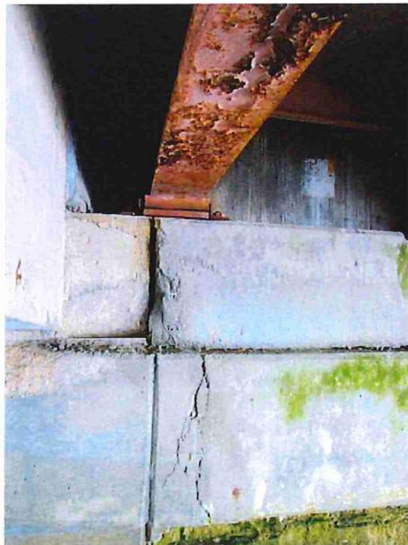
Photo 50: East abutment, at BM1 (South extension). Vertical irregular cracking
