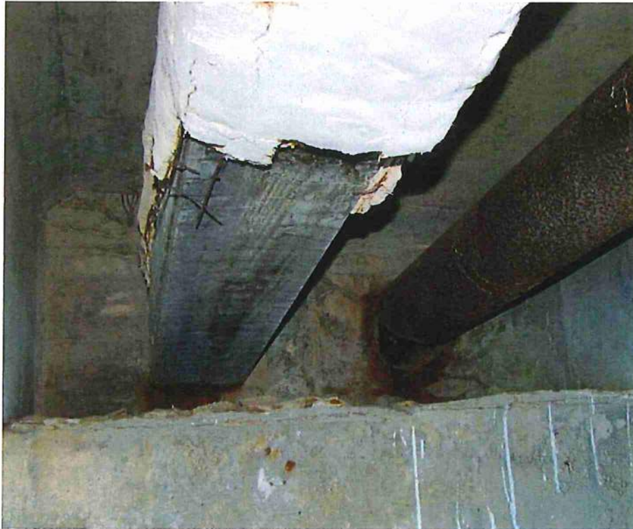
Photo 35: Same utilities as previous photo, span 3 at east abutment. Utility pipe on right with a hole, apparently abandoned
