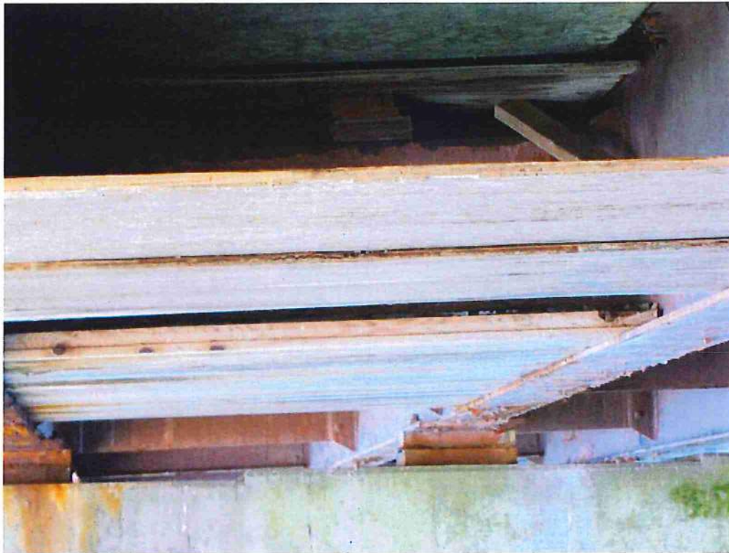
Photo 27: Close up of photo 24. View of wood shielding and formwork left in place at bay 2. Formwork located below full depth deck repair
