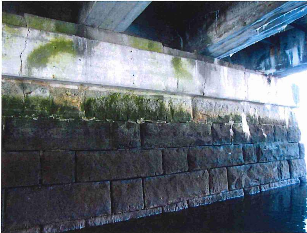
Photo 55: Overview of pier 2, NE. Vertical cracks in cap. Missing pointing
