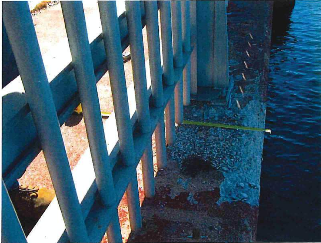
Photo 33: North sidewalk, span 3 north edge spall/scale
