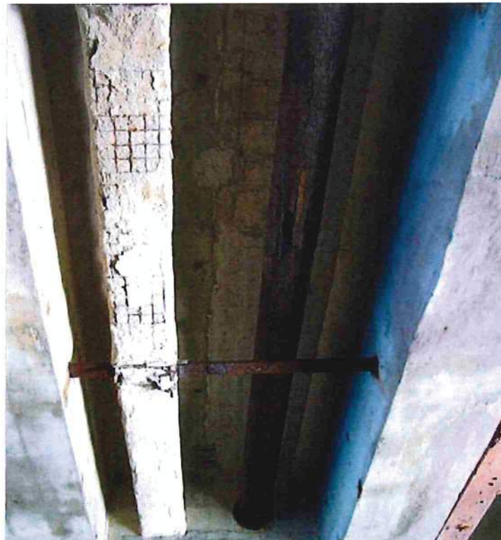
Photo 34: Span 2, bay 5 utilities. Utility pipe on right with holes, apparently abandoned
