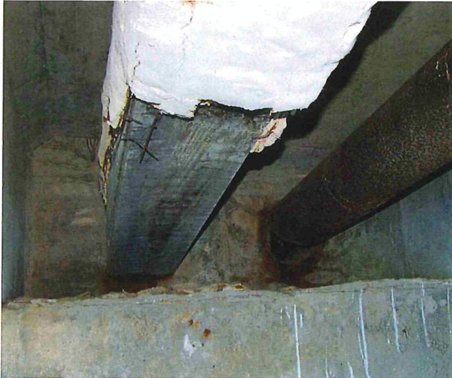
Photo 35: Same utilities as previous photo, span 3 at east abutment. Utility pipe on right with a hole, apparently abandoned
