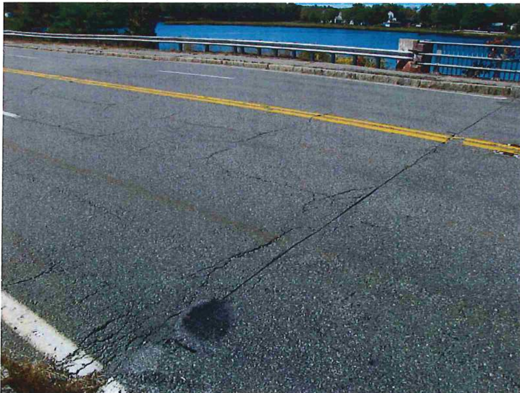
Photo 36: Overview of west approach pavement and sawcut joint. East approach pavement and sawcut joint is similar
