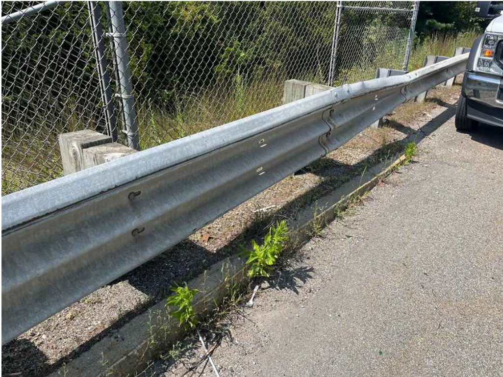
Photo 14: Typical minor scrapes to the approach guardrail. Southwest approach shown.
