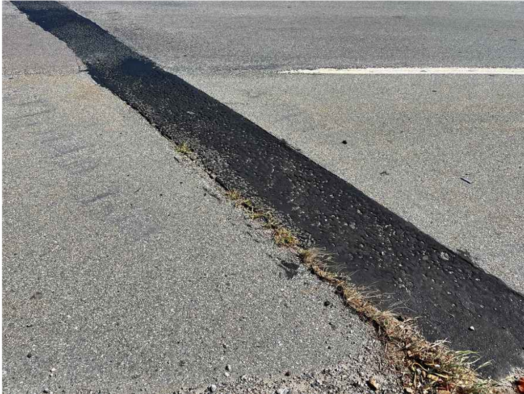
Photo 3: Separation at the plug joint at the south end.
