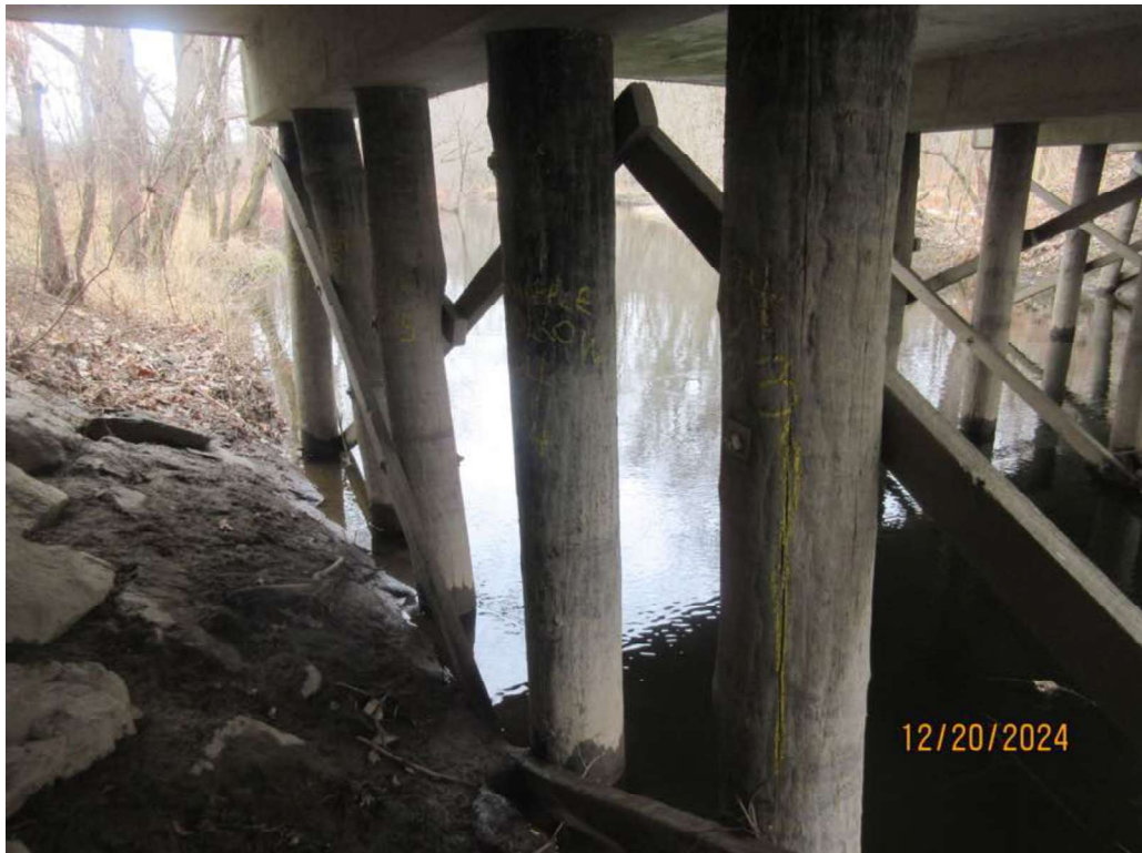
Photo 12: Bent 4, Pile 4 is hollow.
