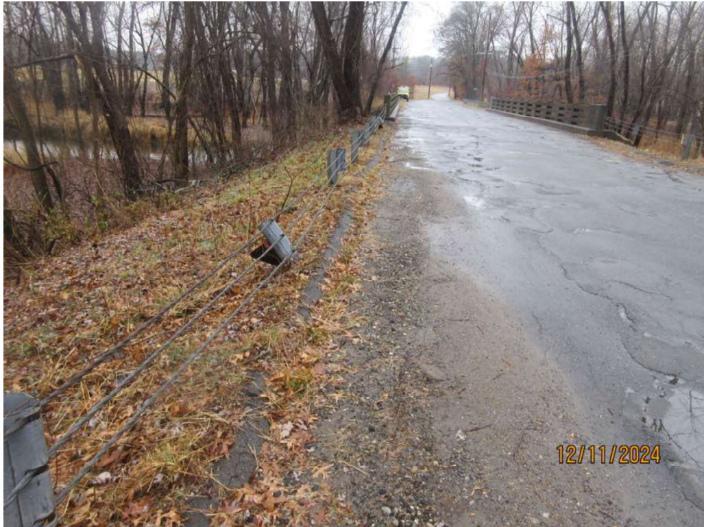
Photo 19: Southwest Approach has 2 blocks out of plum.
