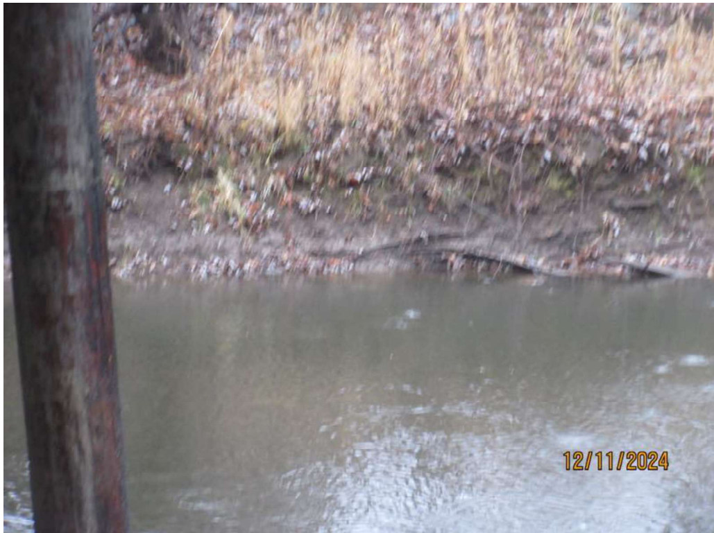
Photo 16: Northeast Embankment has erosion.
