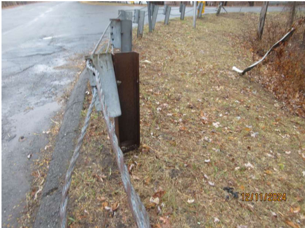
Photo 20: Northeast Approach guardrail post has rust hole at ground level.
