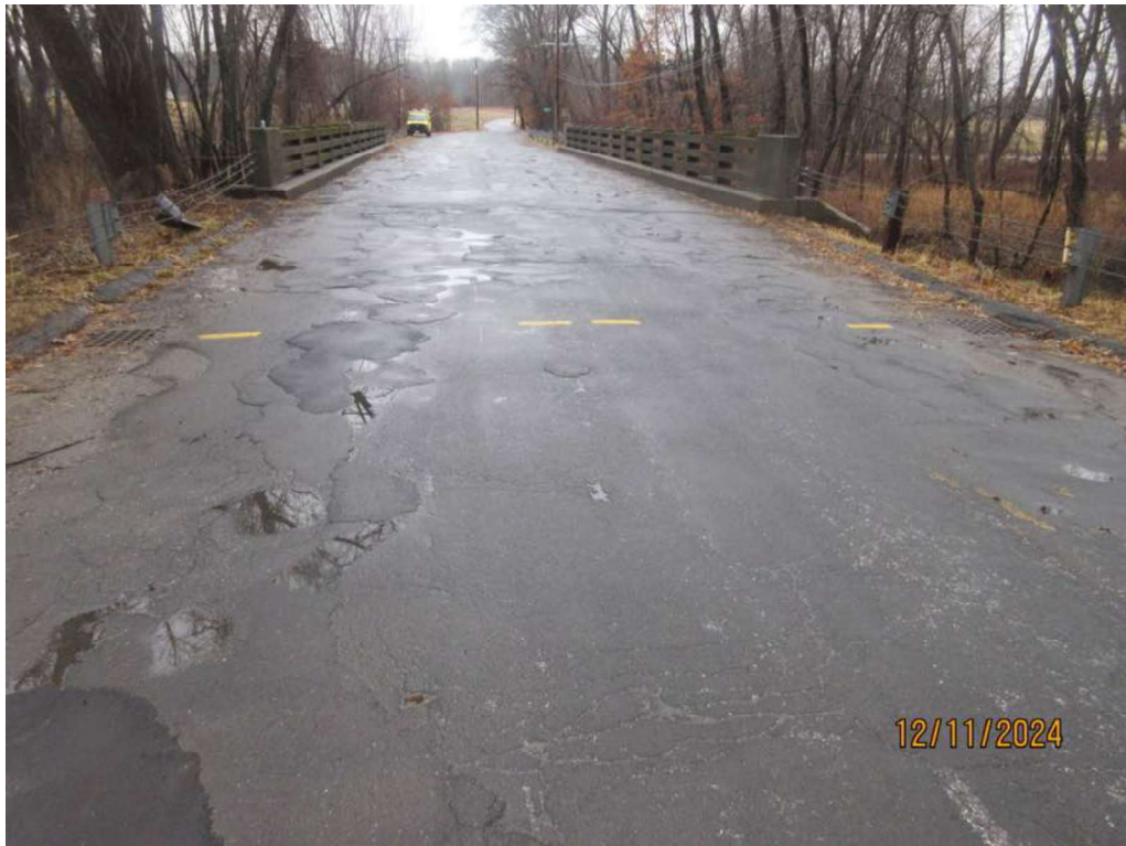
Photo 8: South Approach roadway has multi-cracking with several HMA patches with uneven profile.
