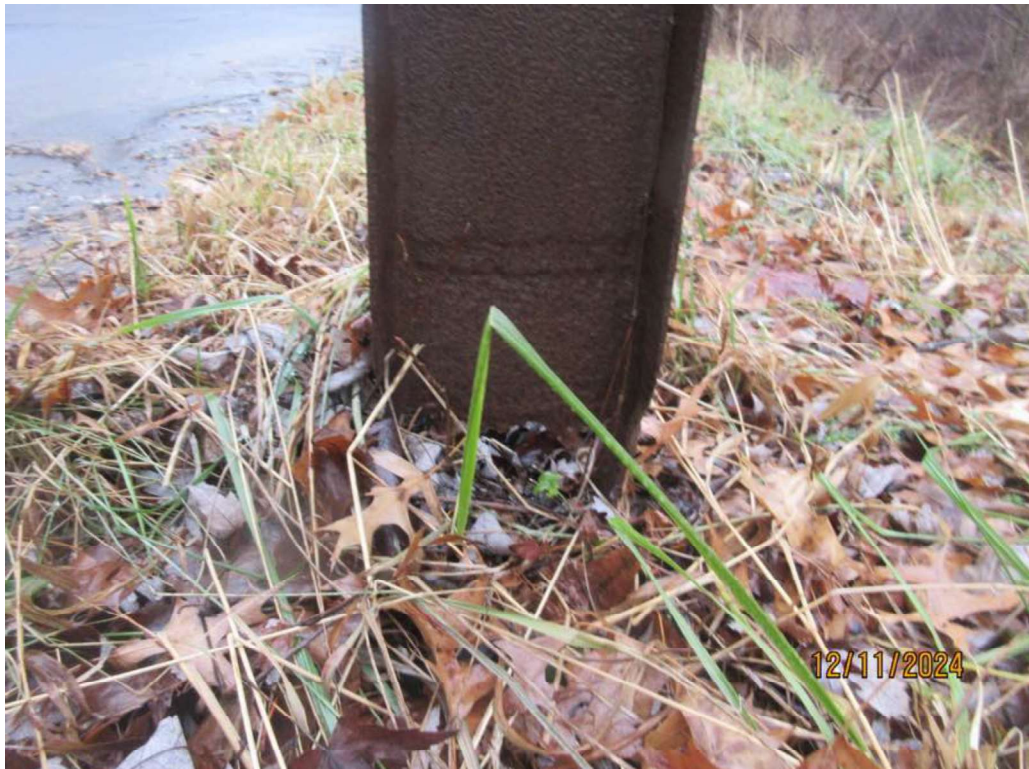
Photo 18: Southwest Approach guardrail post has hole in post at ground level.
