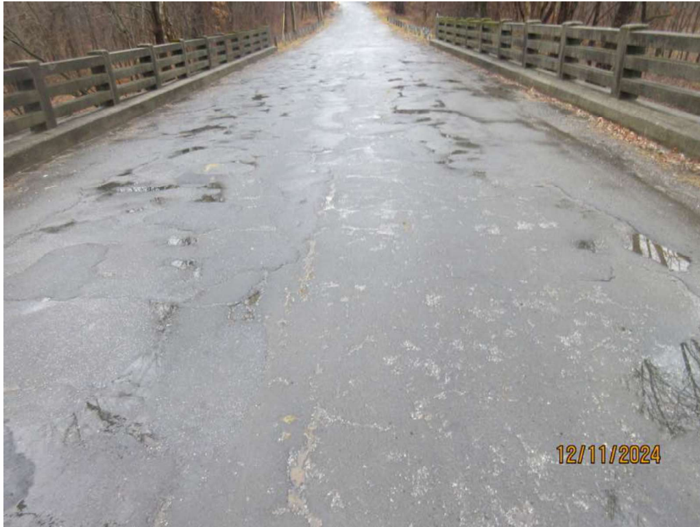
Photo 1: Wearing Surface has several HMA patches with an uneven profile.
