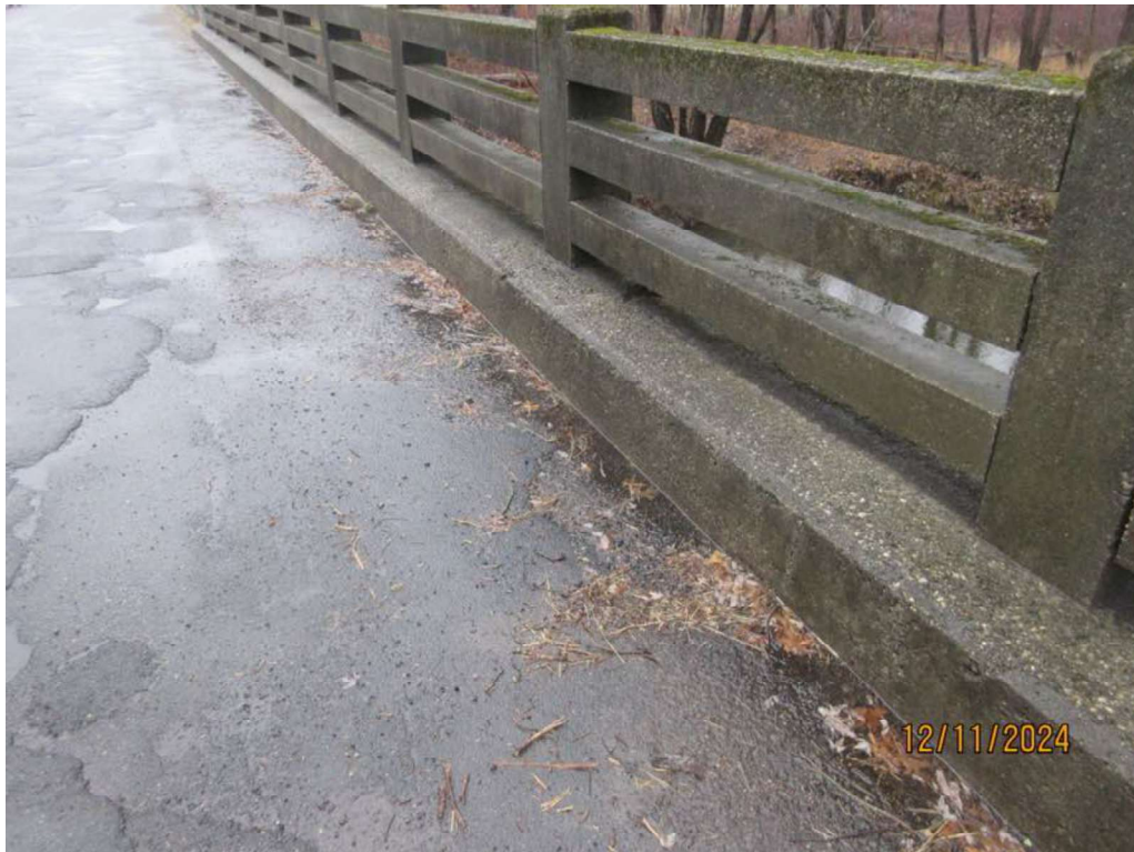
Photo 4: East concrete curbs has minor scaling and random vertical hairline cracks.
