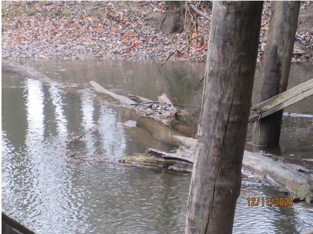
Photo 17: Logs built up against Bent 3.
