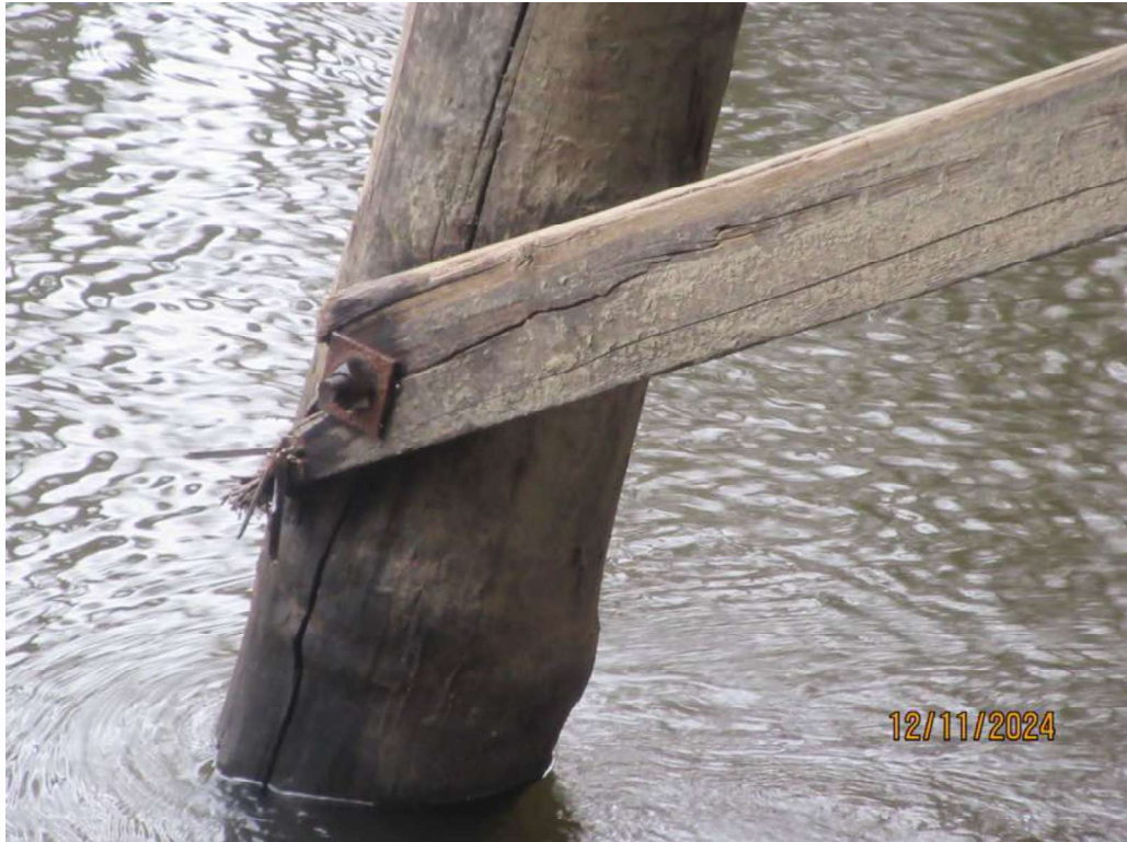
Photo 13: Bent 2, Pile 1 at lower bolt, brace is split.
