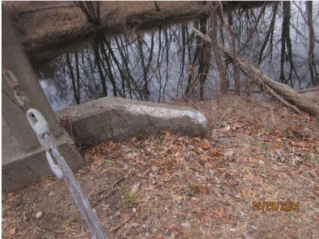
Photo 9: Southeast Wingwall is spalled 3' long x 6" wide x 6" deep.
