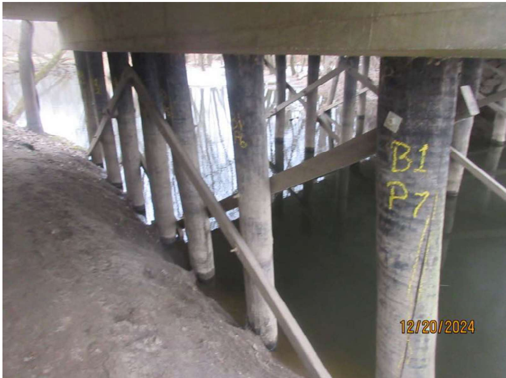
Photo 10: Bent 1 has deterioration.
