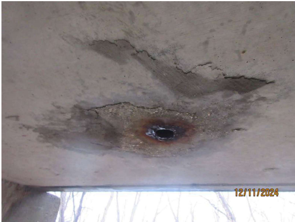
Photo 2: Deck Underside, concrete around these drain pipes are delaminated with some having mortar patching.
