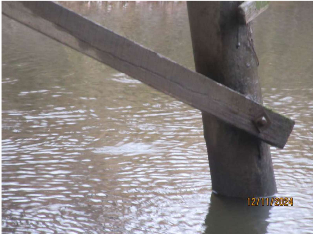
Photo 15: Bent 3, Pile 6, at lower bolt, the brace is split.
