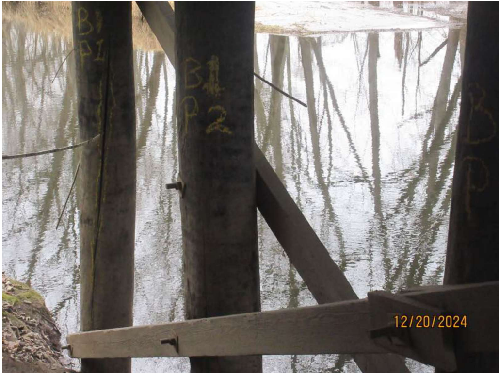
Photo 11: Bent 1, Pile 1, has split 1/2" wide x 5" deep x up to 8" high.
