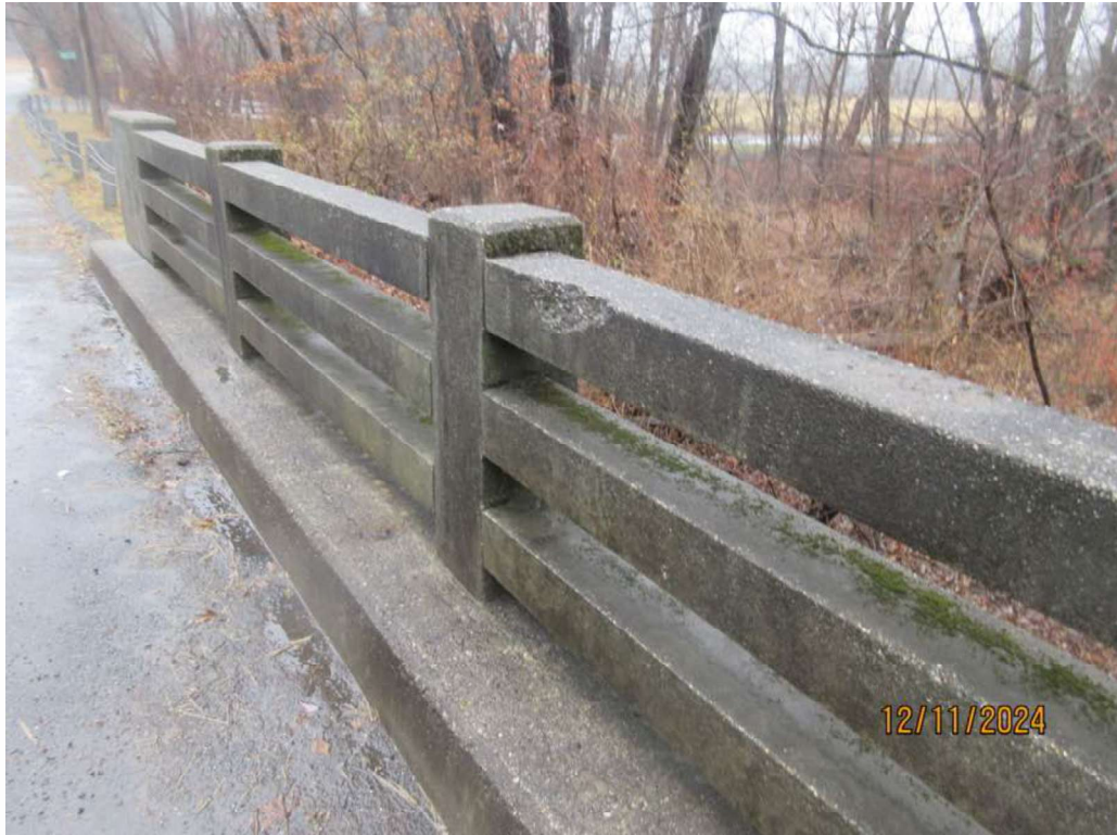
Photo 5: East top Concrete Railings have minor spall.
