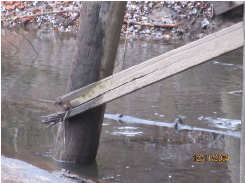
Photo 14: Bent 3, Pile 1, at lower bolt, the brace is split.
