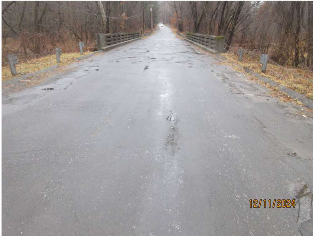
Photo 7: North Approach roadway has multi-cracking with several HMA patches with uneven profile.
