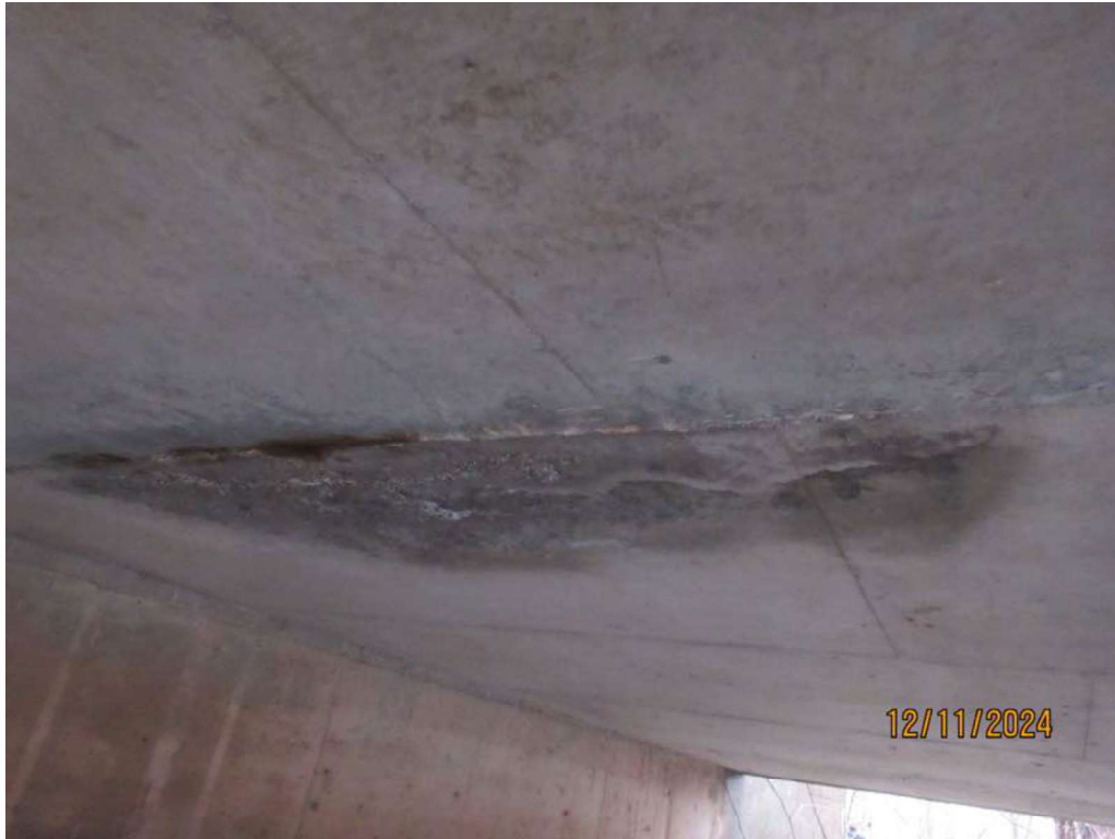
Photo 3: Deck Underside, Span 1, has heavy efflorescence, rust staining & minor scaling. Center construction joint has a hollow area.
