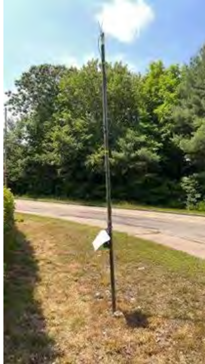
Figure C-6. Project 609440, Segment 1: Detector Facing West
