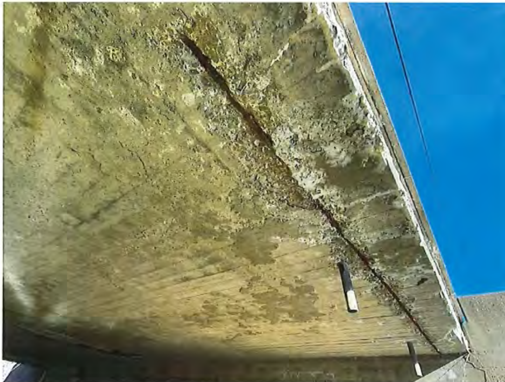
Photo 10: Span 3 deterioration at the south end.
