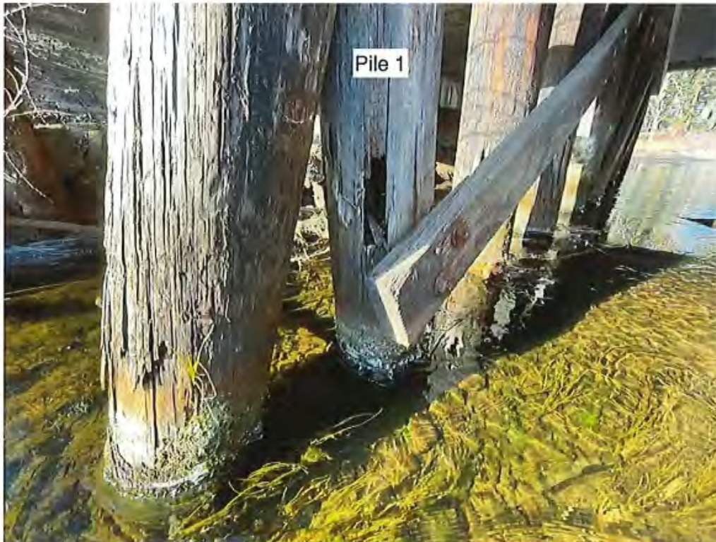
Photo 20: Bent 2 pile 1 deterioration.
