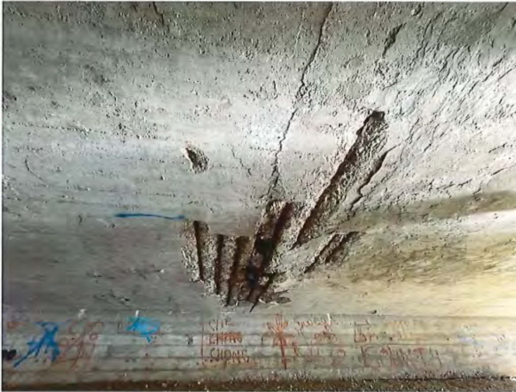
Photo 9: Span 3 deterioration at the center construction joint.
