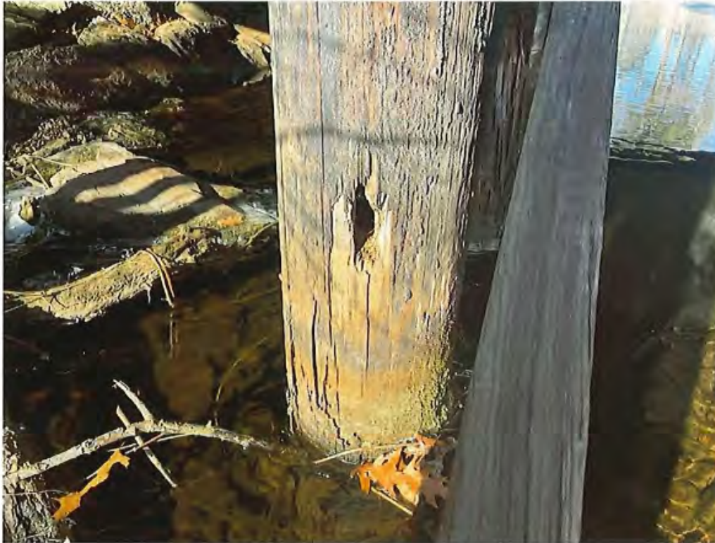
Photo 21: Bent 2 pile 2 deterioration.
