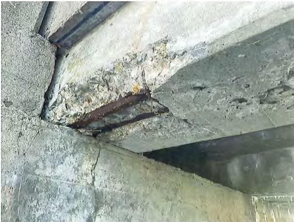
Photo 16: Span 3 sidewalk beam deterioration at the east end.
