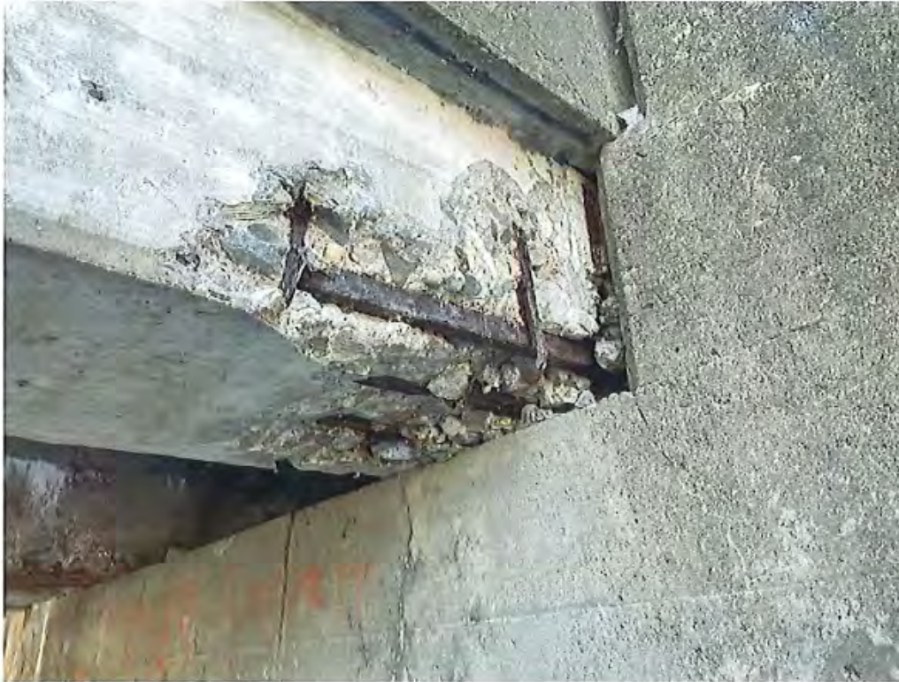
Photo 13: North sidewalk beam deterioration at the west end in span 1.
