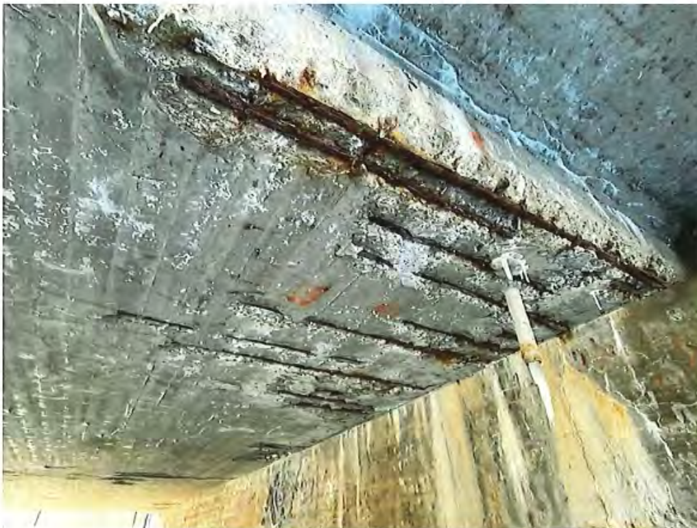
Photo 6: Span 1 deterioration at the northwest corner.
