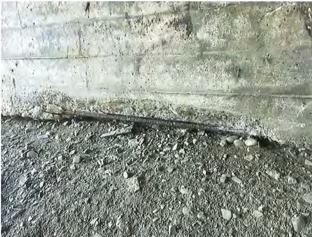
Photo 18: East abutment bent deterioration under the north sidewalk.
