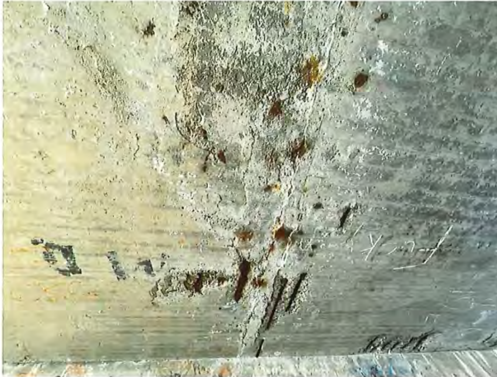
Photo 5: Span 1 deterioration at the center construction joint.
