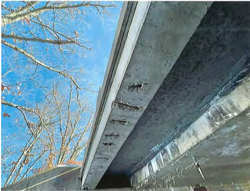
Photo 15: Span 3 sidewalk beam deterioration.
