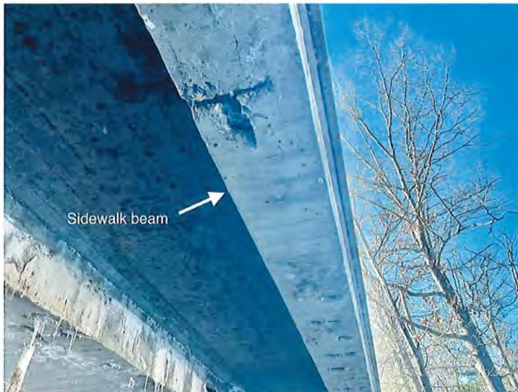
Photo 14: Span 2 sidewalk beam deterioration.
