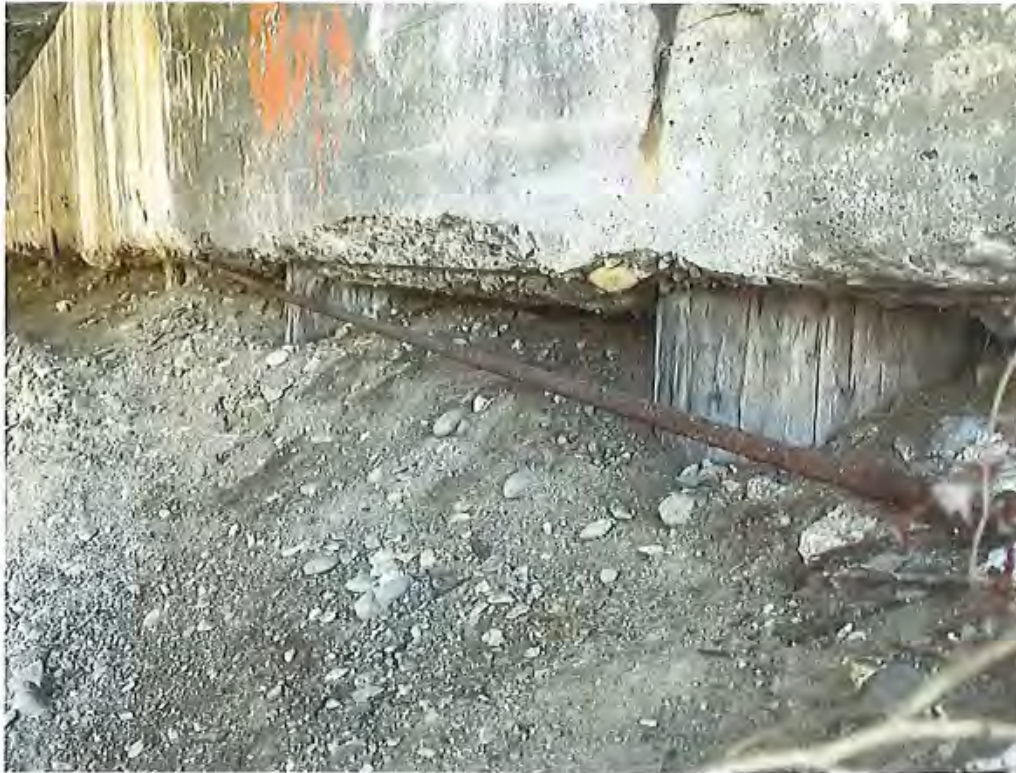
Photo 17: West abutment bent deterioration. Note the embankment erosion exposing the piles.
