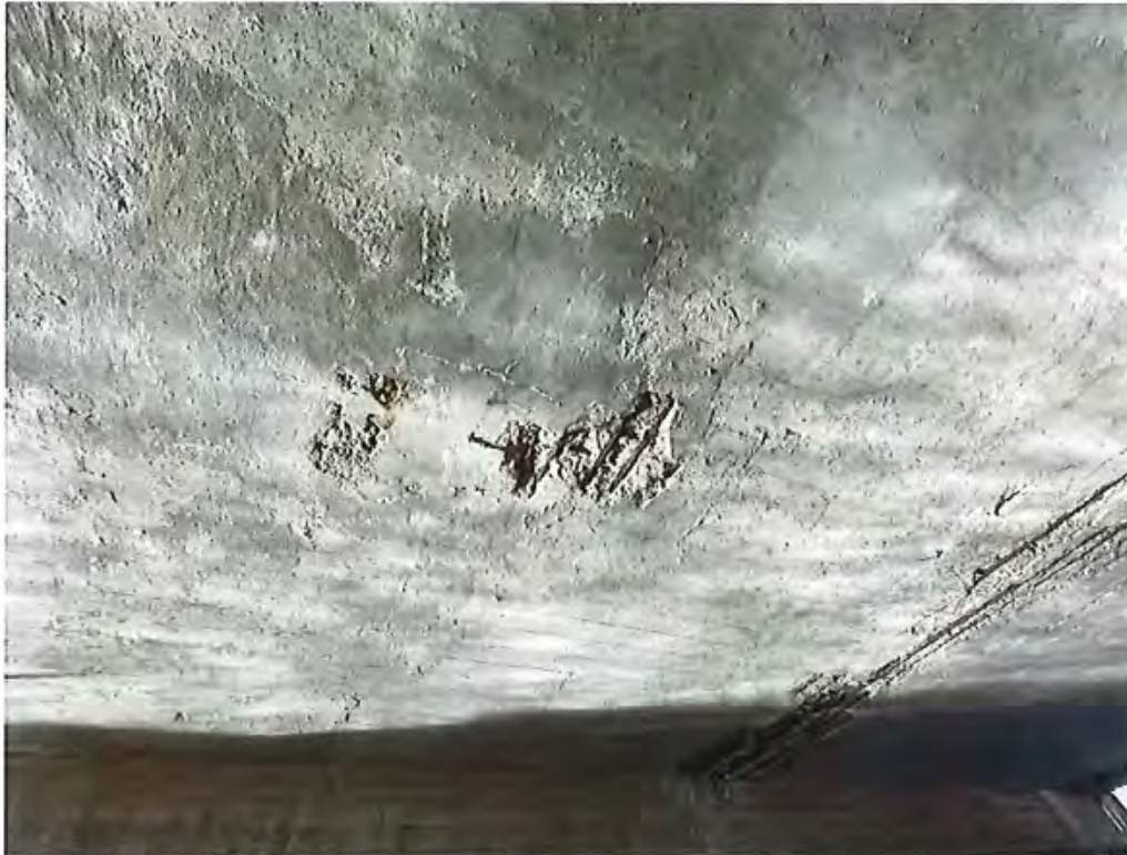
Photo 7: Span 2 deterioration to the south half at center.
