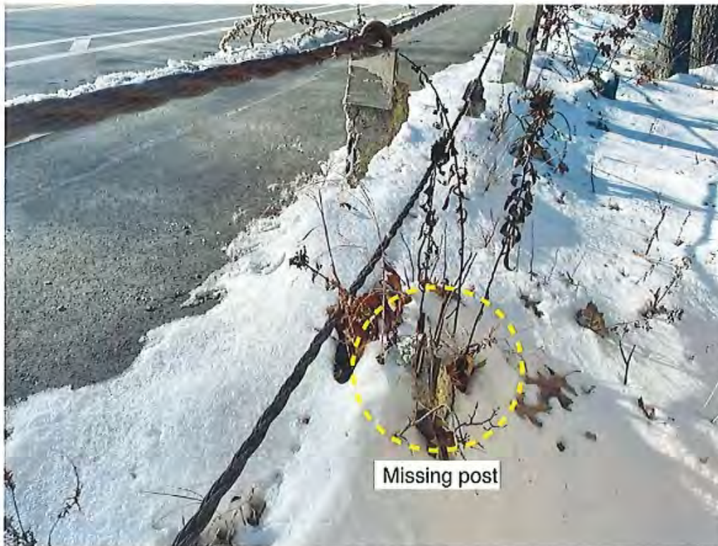
Photo 25: Southwest approach traffic safety feature missing post.
