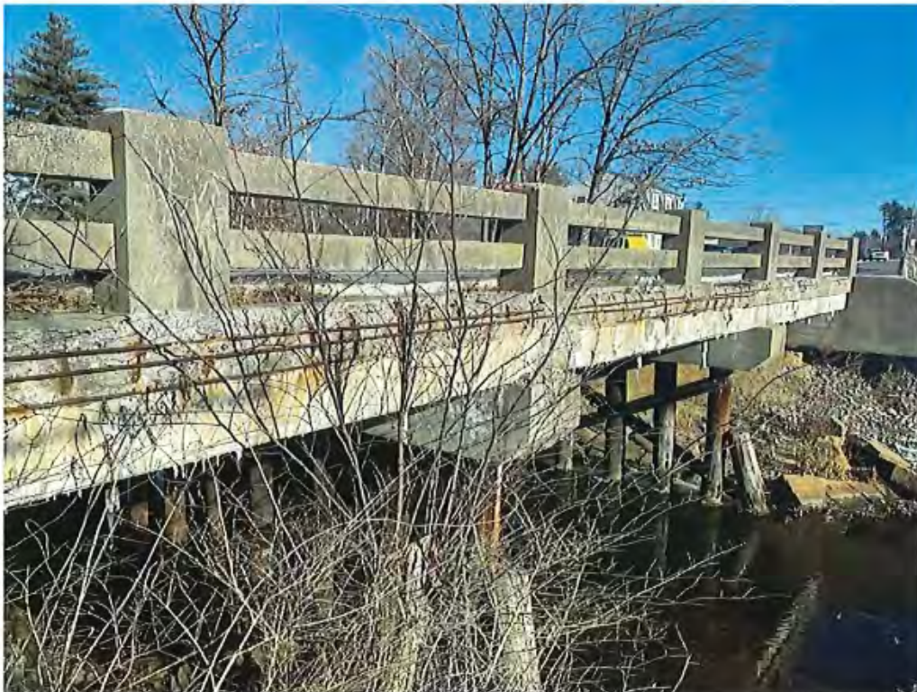
Photo 2: South fascia and railing base deterioration.
