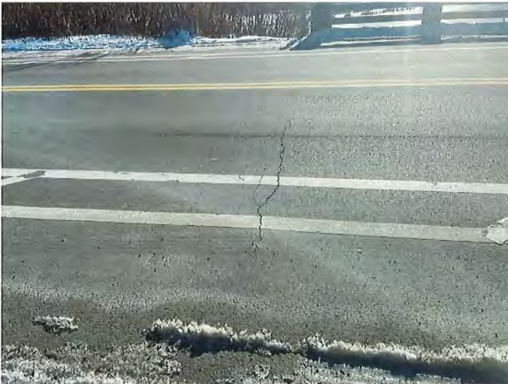
Photo 12: Transverse cracking in the westbound lane at the east deck transition.
