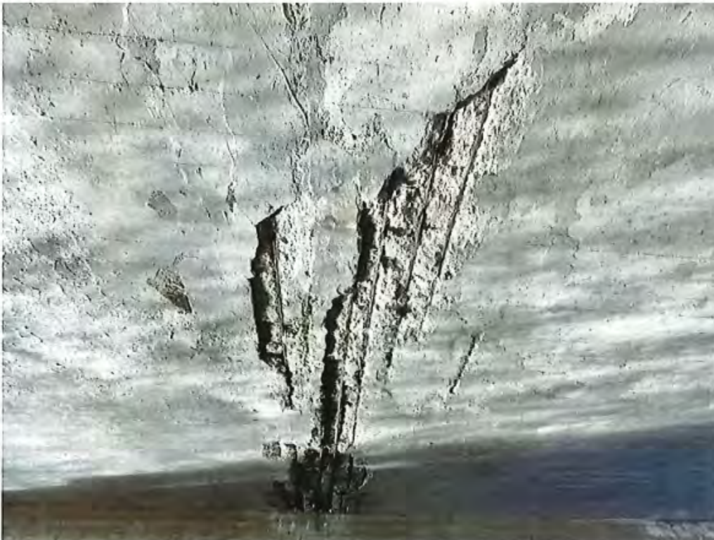
Photo 8: Span 2 deterioration at the center construction joint.
