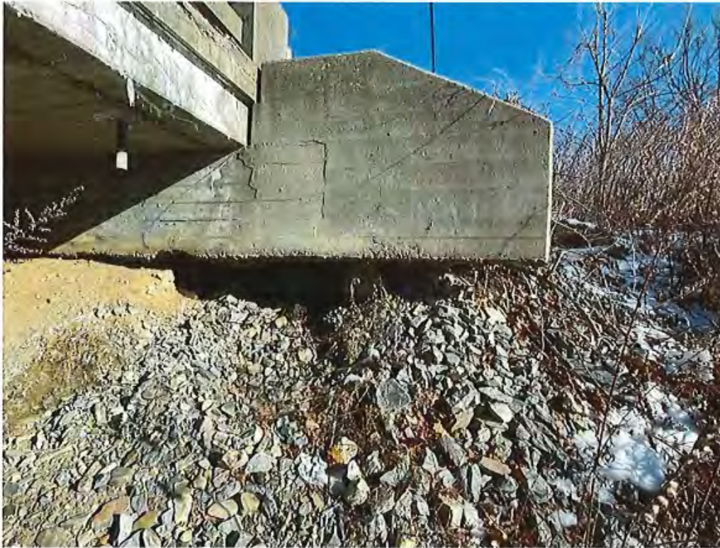
Photo 19: Embankment erosion at the southeast wingwall.
