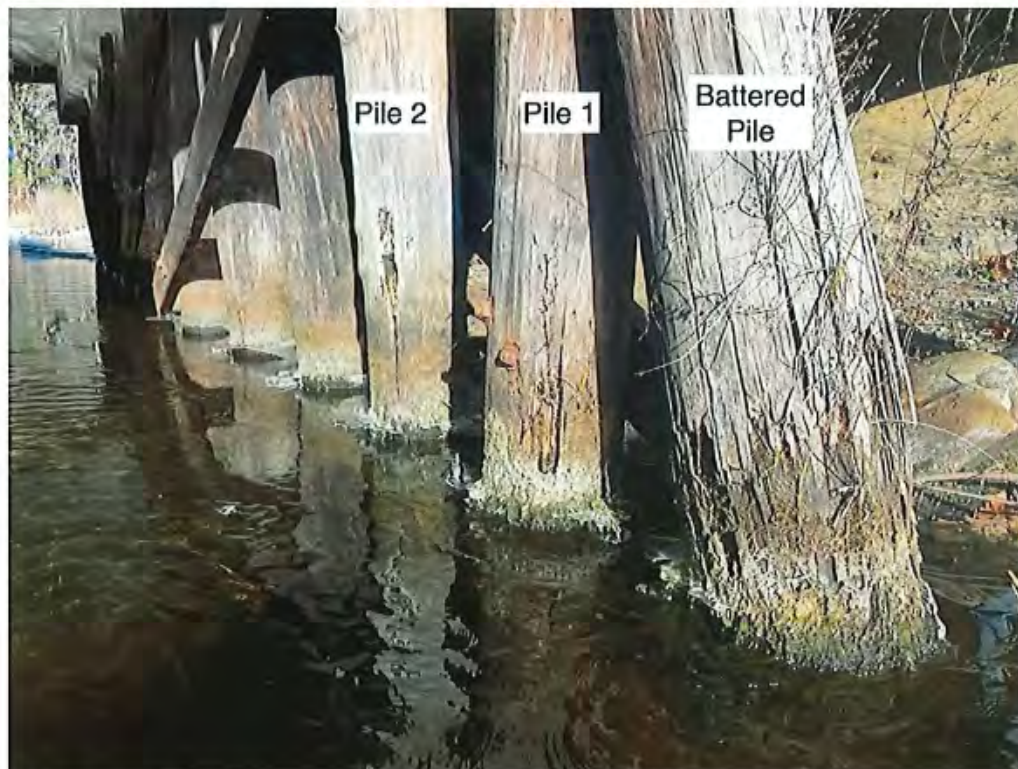
Photo 22: Bent 3 pile deterioration at the waterline.
