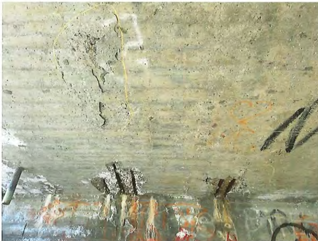
Photo 4: Span 1 spalls and delamination at the southwest corner.
