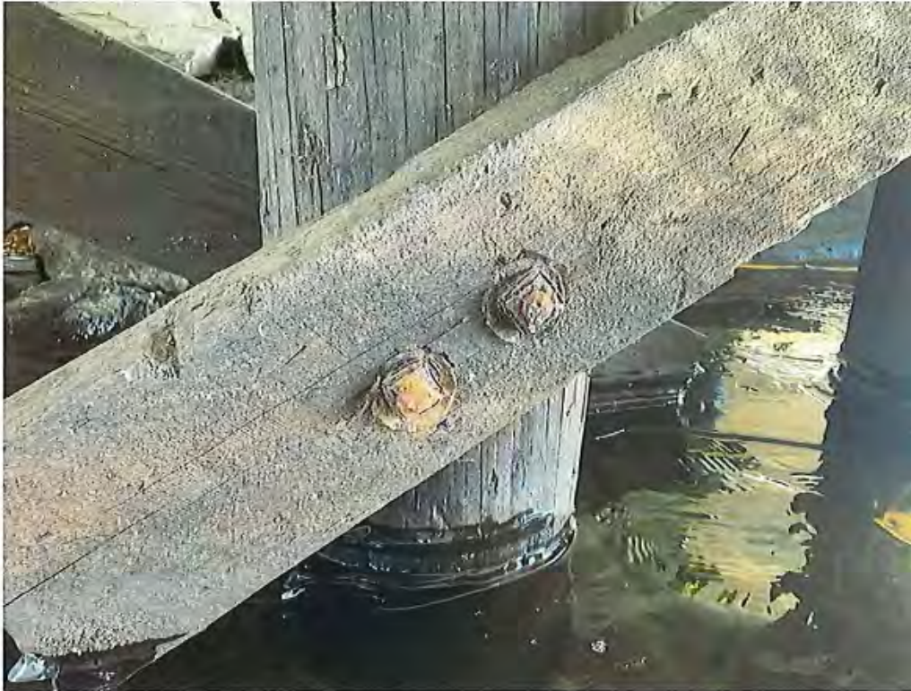
Photo 23: Typical condition of the bents 2 and 3 fasteners at the waterline.
