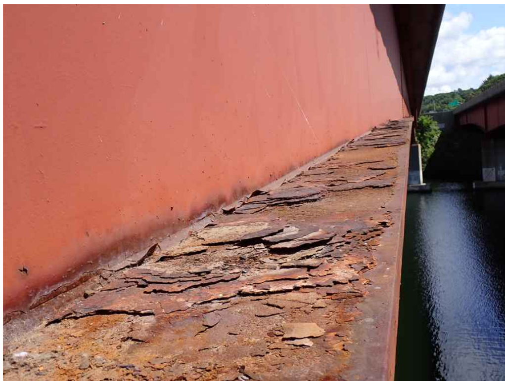
Photo 17: Span 3 girder 4 at splice 1, looking east. Typical girder 4 bottom flange flaking in spans 2 & 3.
