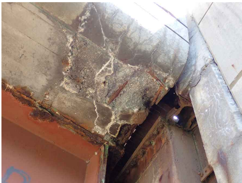
Photo 4: Span 4 south soffit east end, looking northeast. Note missing drain at right and missing drainage trough.
