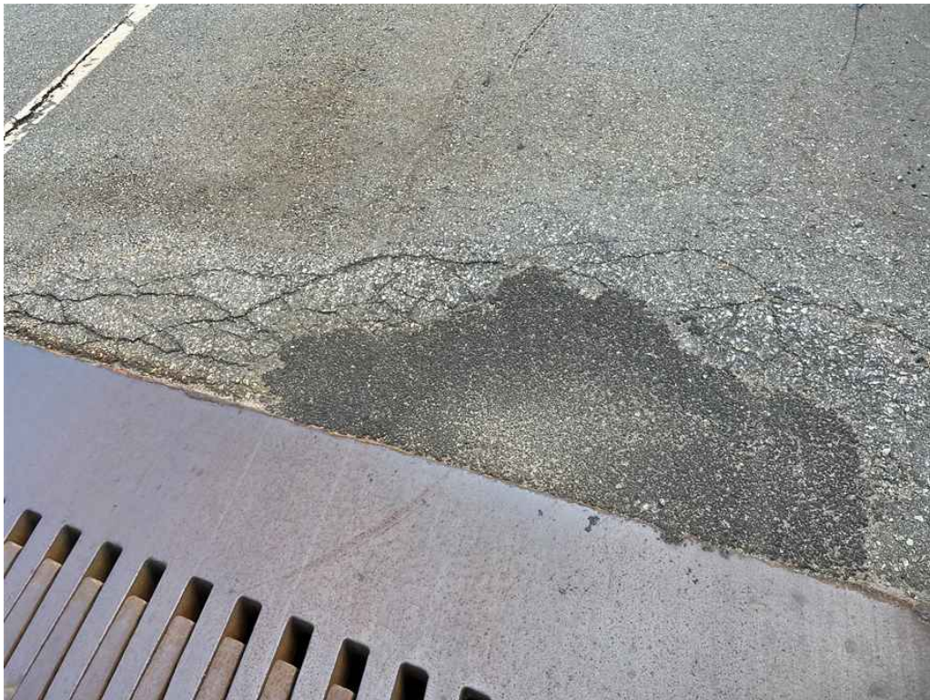
Photo 16: Patch at the east approach adjacent to the south end of the east joint.
