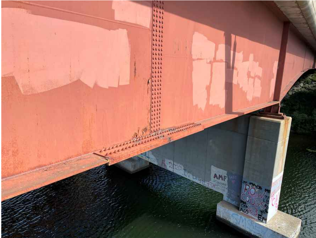
Photo 23: Typical paint condition and painted over graffiti. Span #3, girder #8 shown.
