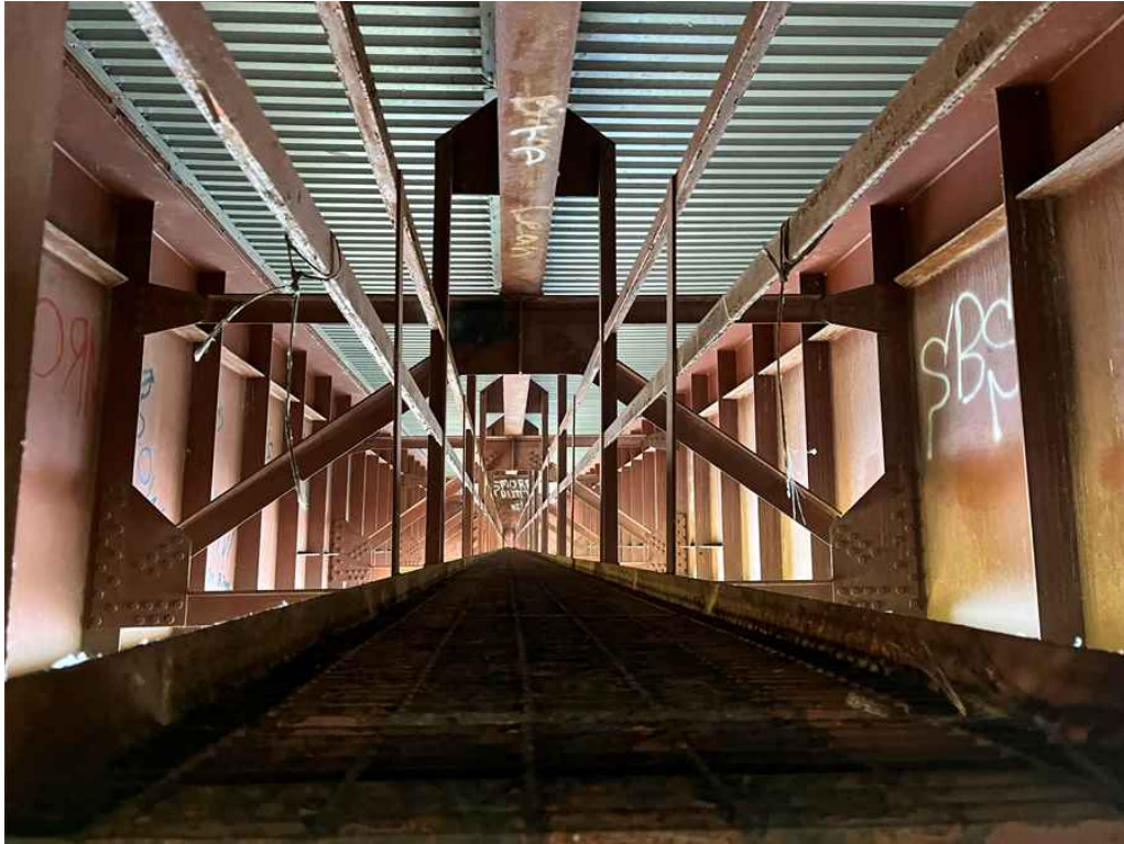
Photo 29: Unsecured east end of the catwalk in span #4.
