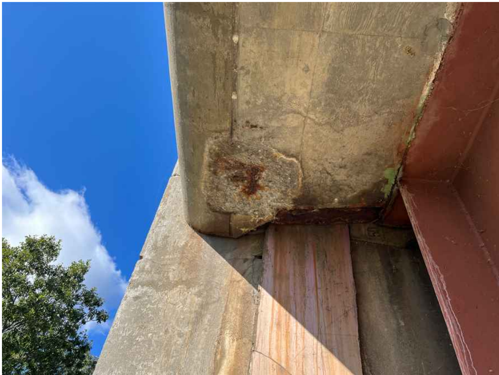
Photo 4: Spall to the south soffit at the west end.
