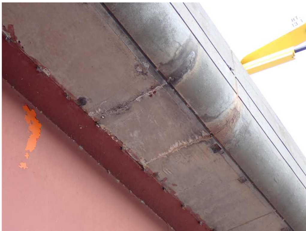
Photo 3: Span 4 north fascia/soffit near pier 3, looking southwest. Typical cracking with efflorescence.
