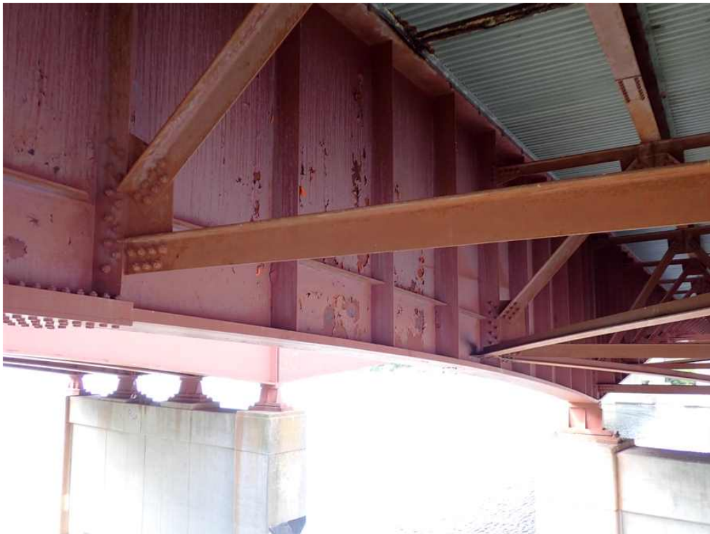
Photo 32: Span 4 girder 4 west end north face. Typical paint peel.
