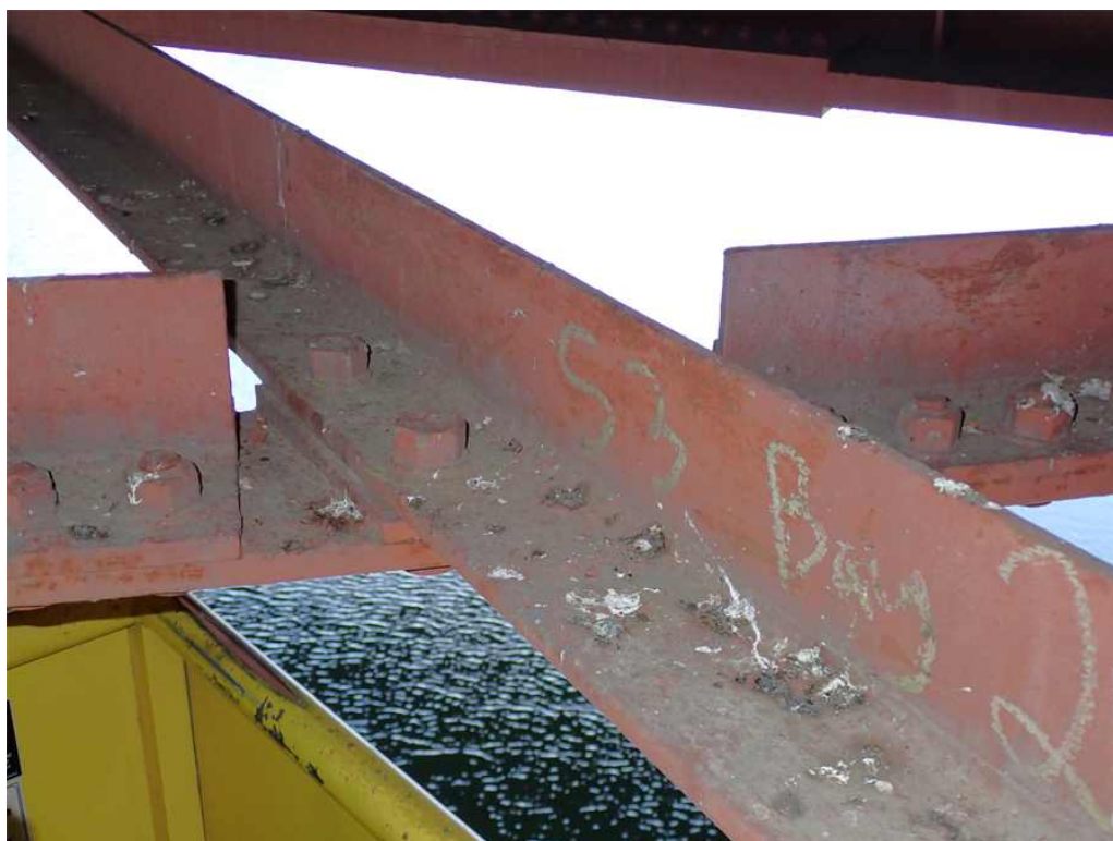
Photo 28: Span 3 cross brace 2 between girders 2 & 3, looking southeast. Note nuts not fully threaded at left.
