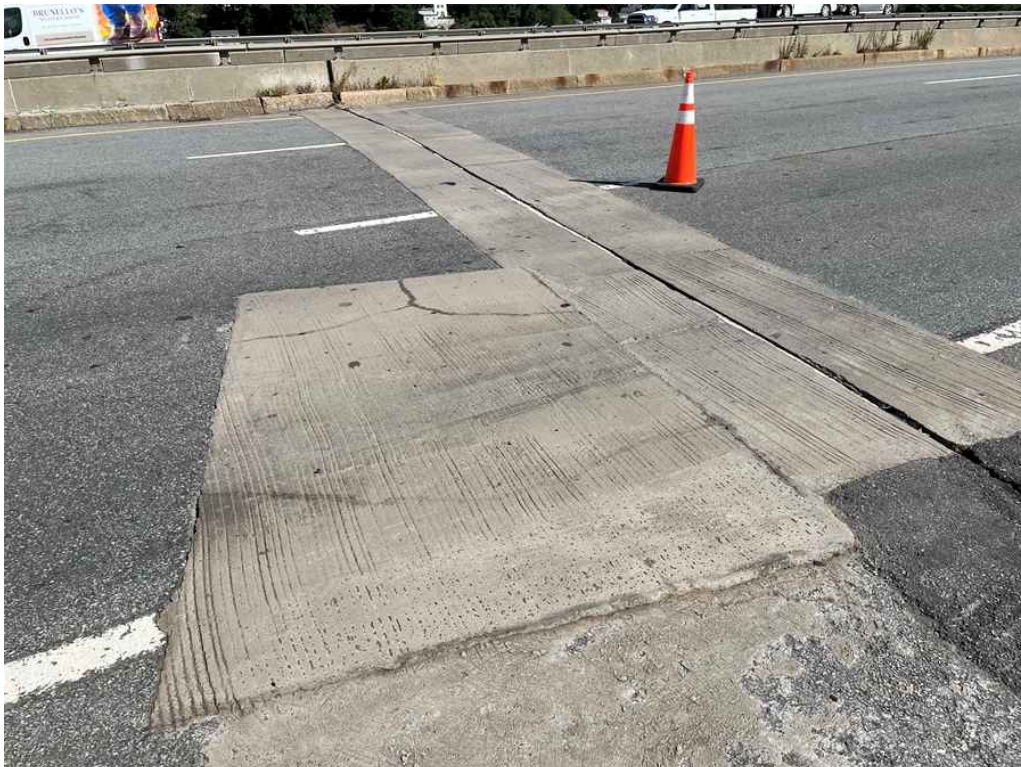
Photo 2: Concrete patch in span #1 adjacent to pier #1 joint. Note pier #1 joint.
