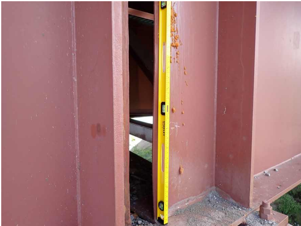
Photo 20: Span 1 girder 9 east end north face at pier 1, looking southwest. Note southward web bottom distortion.
