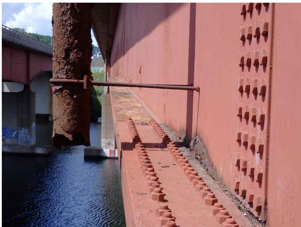
Photo 18: Span 3 girder 4 splice 3, looking west. Note minor rust flaking at web bottom.
