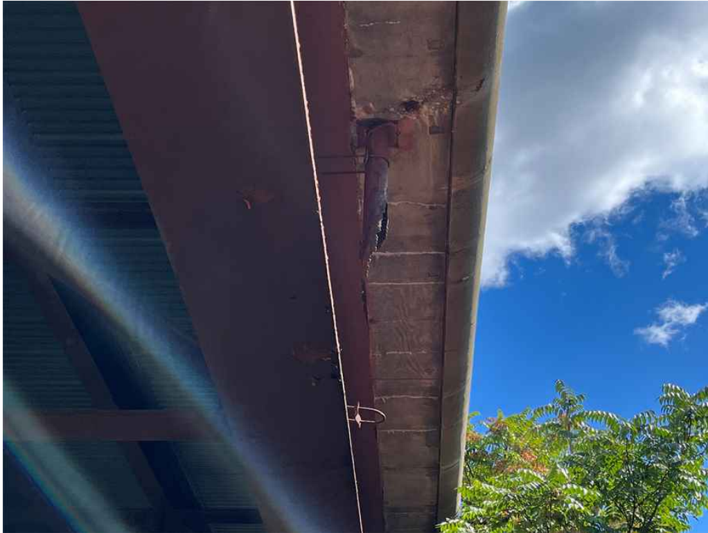
Photo 13: Span #4, south scupper with 100% section loss.
