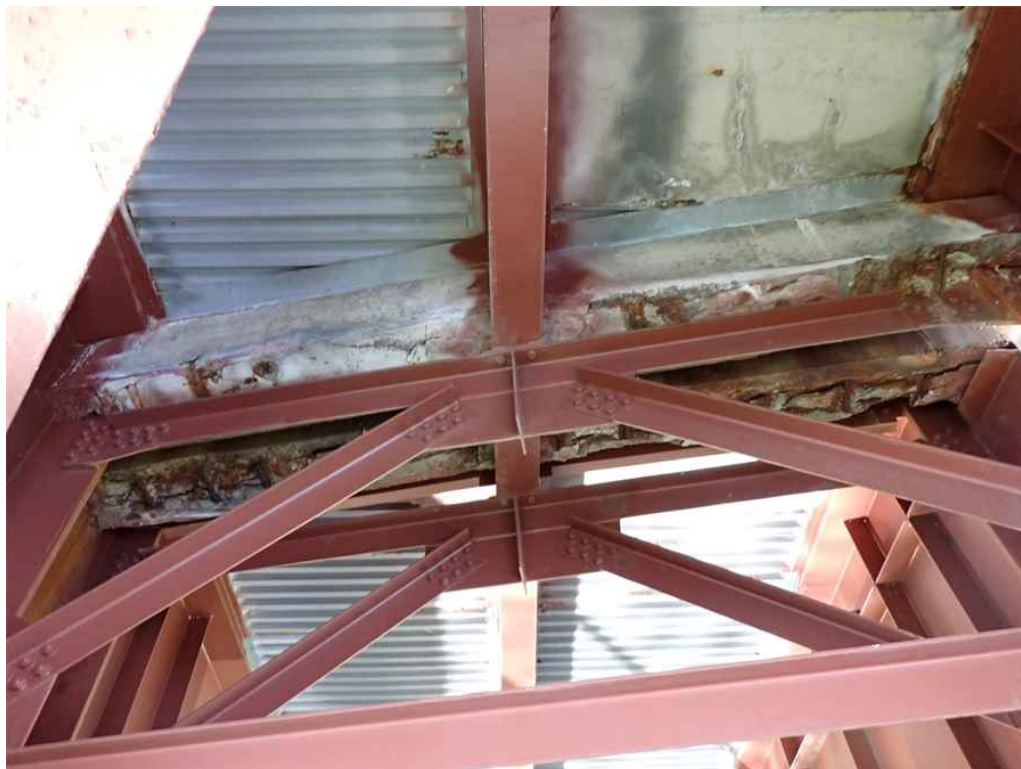
Photo 24: Pier 1 bays 1 & 2, looking west. Typical pier 1 end diaphragm condition.
