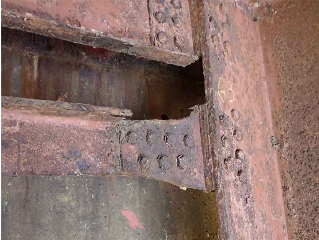
Photo 25: Span 4 girder 2 east end north face top connection plate, looking southeast (below open joint).
