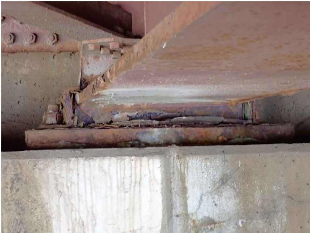
Photo 22: Span 1 girder 2 west abutment end. Note typical bent/rusted keeper plate at left.
