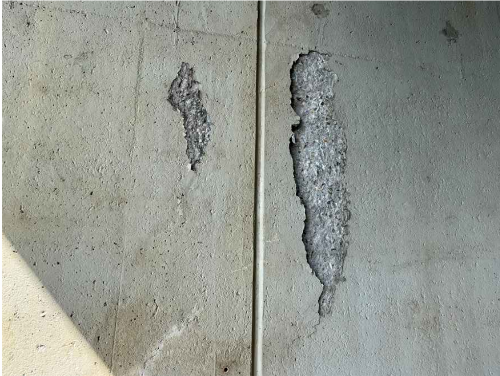
Photo 31: Pier #1, east face at the top.
