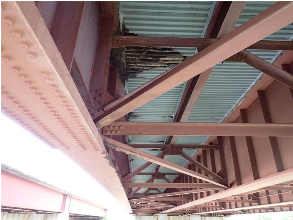
Photo 6: Span 2 bays 5 & 6, looking west. Typical SIP form corrosion.
