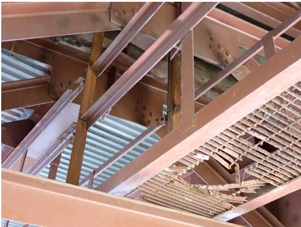
Photo 34: Catwalk at pier 1, looking southeast. Note 100% section loss at platform and rail.
