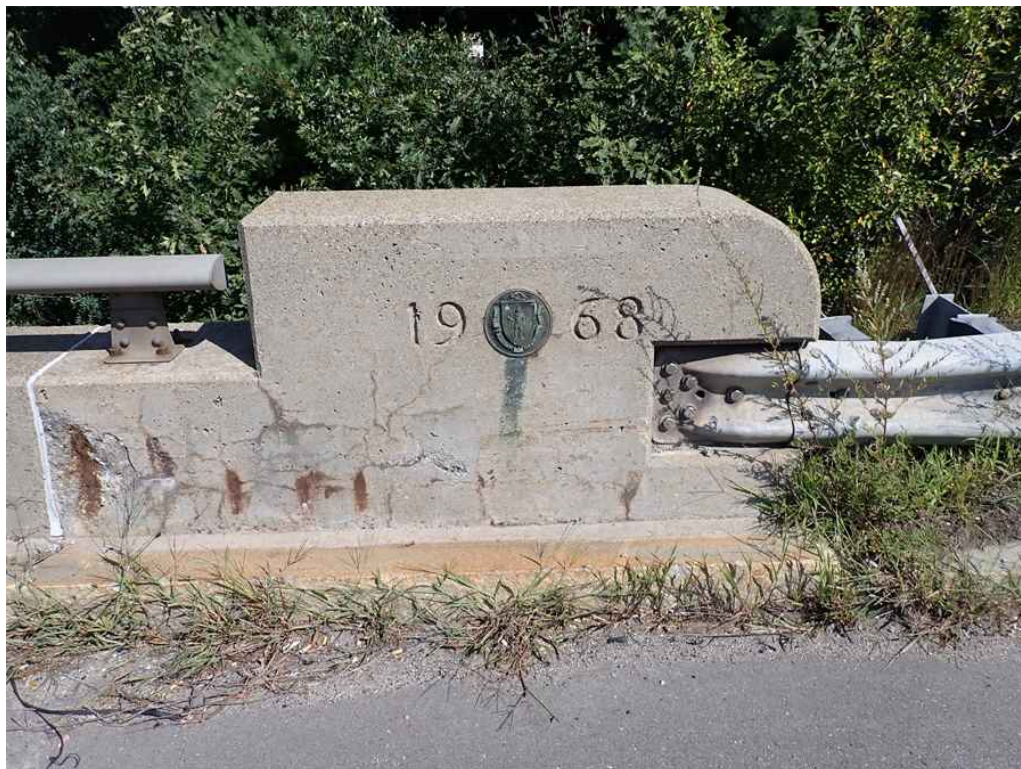
Photo 36: Northeast transition, looking north. Note typical missing connector panel bolt.
