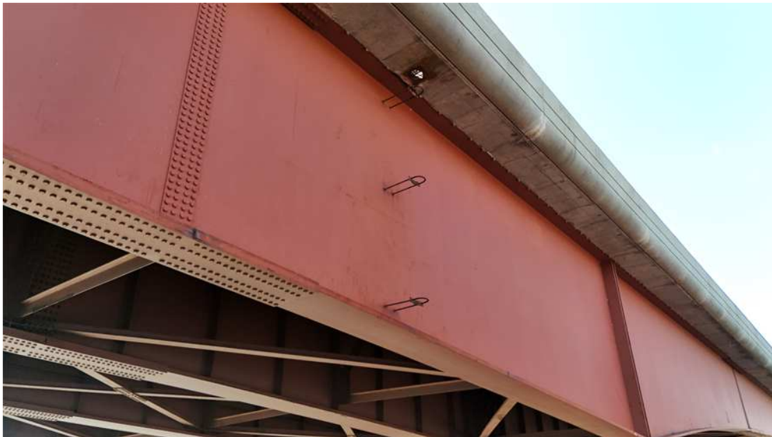
Photo 12: Missing north scupper pipe in span #4.
