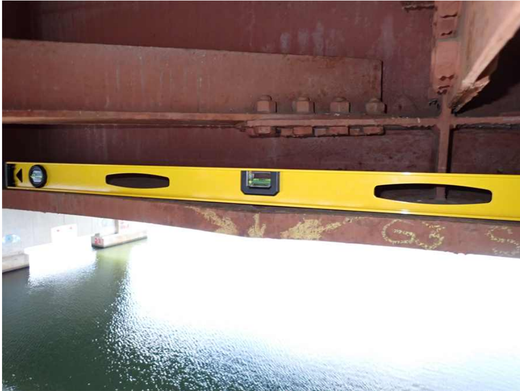
Photo 21: Span 2 girder 2 at 1/4 point from pier 1, looking southeast. Note isolated bottom flange distortion.
