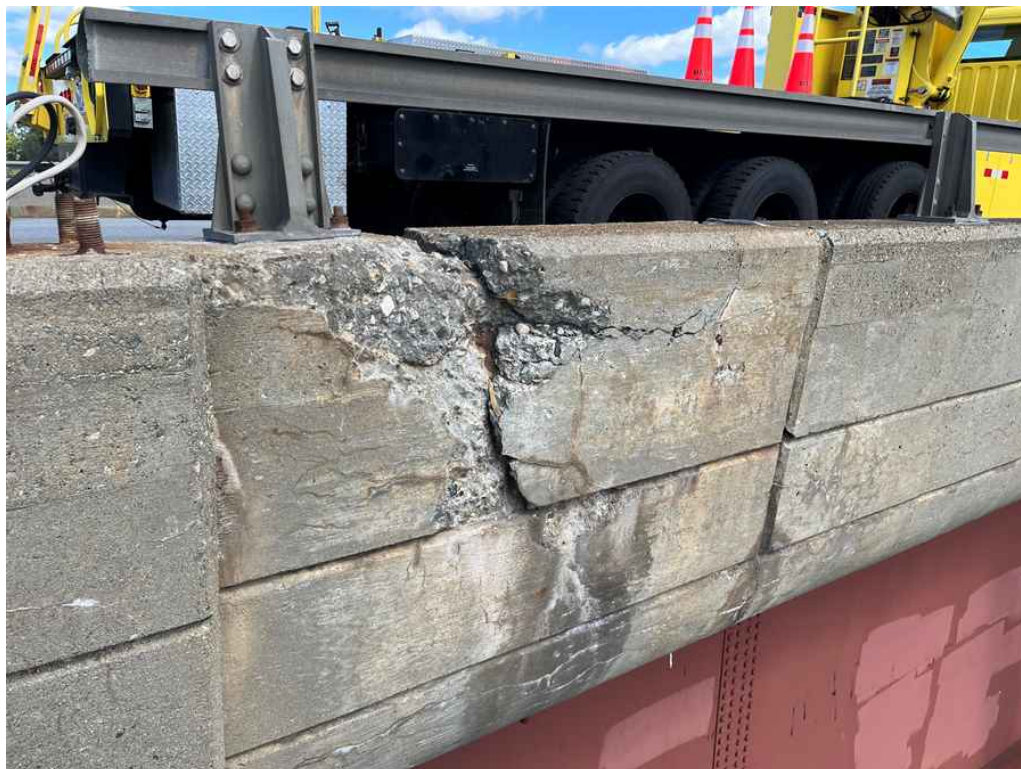
Photo 10: Condition of the south parapet at the utility box. Span #3 shown.
