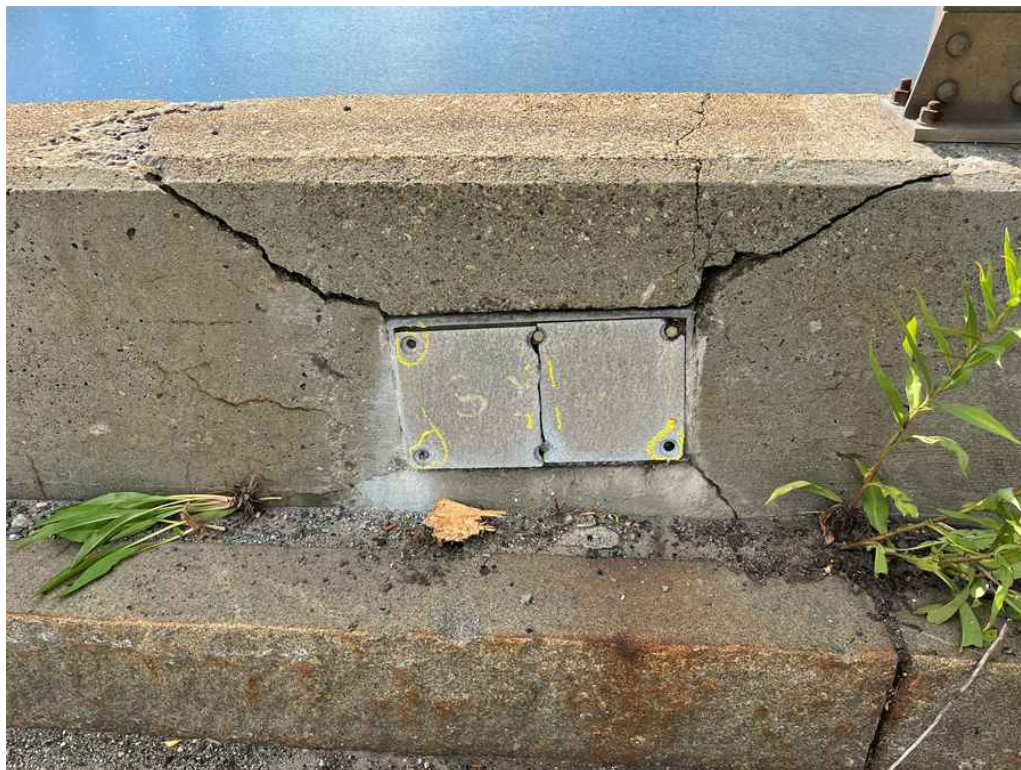
Photo 9: Utility junction box at the south parapet in span #1. Note condition of the utility box.
