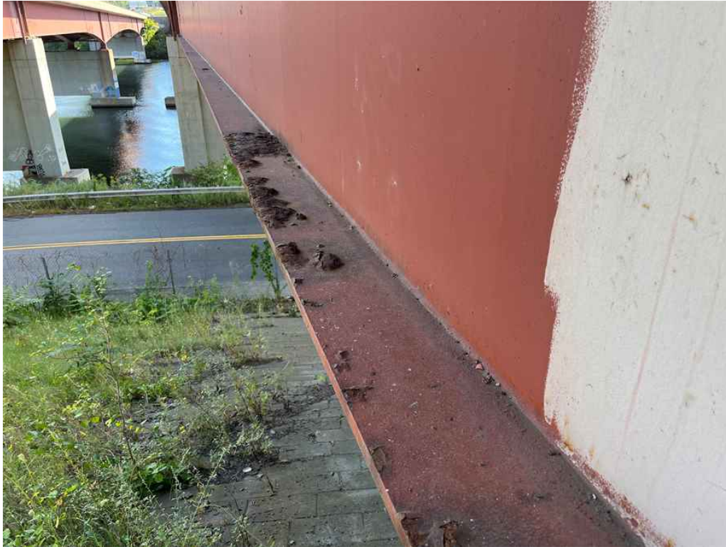
Photo 17: Corrosion to the bottom flange of girder #13 in span #1.
