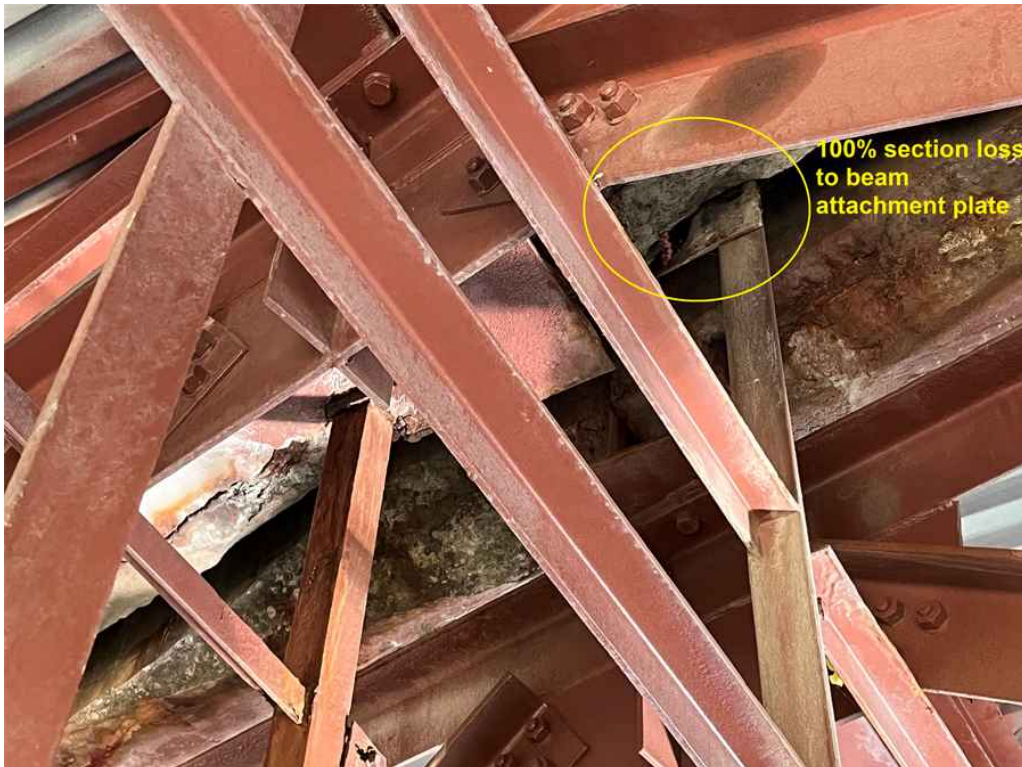
Photo 28: Section loss to the vertical connections over pier #1.
