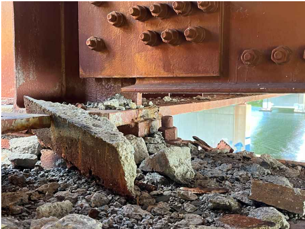
Photo 20: Missing keeper plate to girder #5 bearing at pier #1.
