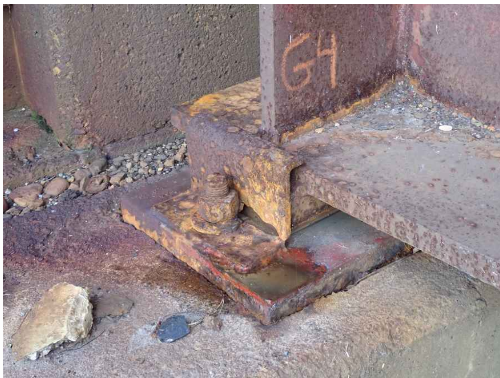
Photo 23: Span 4 girder 1 east abutment end north face. Note typical 100% section loss at keeper plate.
