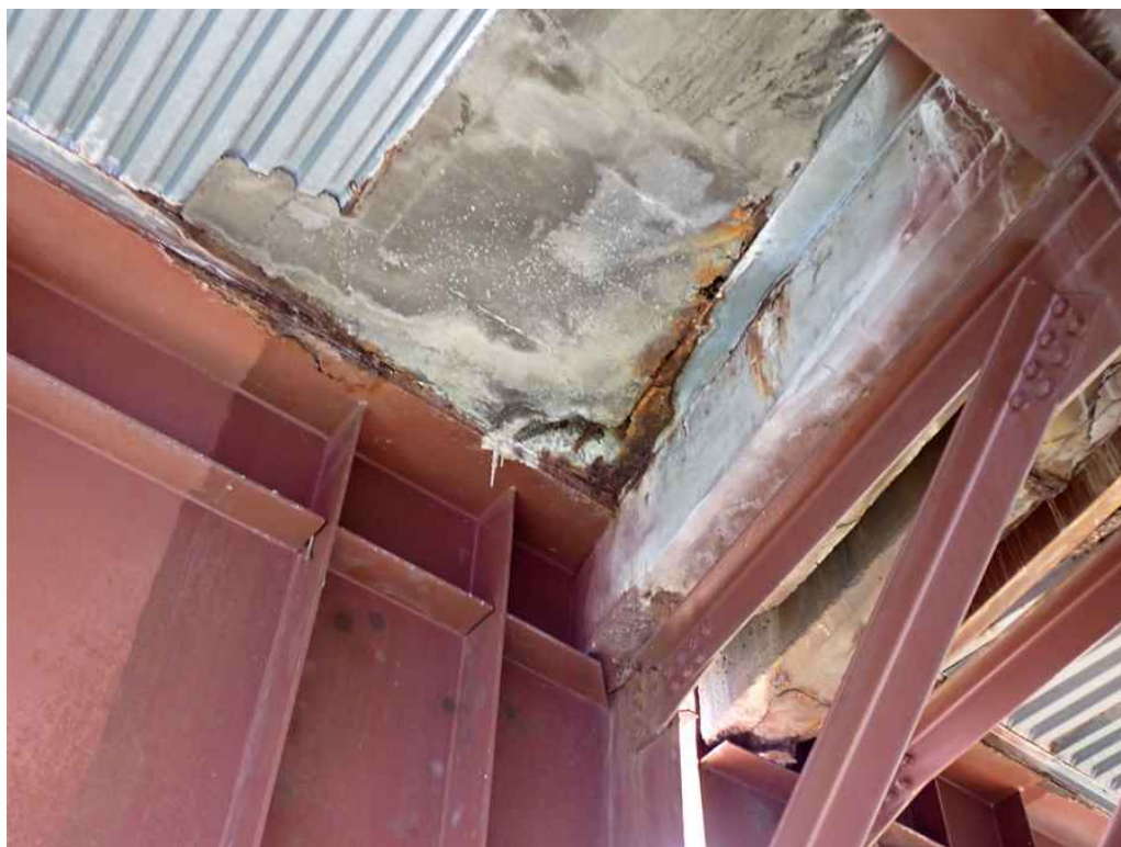
Photo 9: Span 2 bay 6 west end at pier 1, looking southwest. Note bay 6 corner spall.
