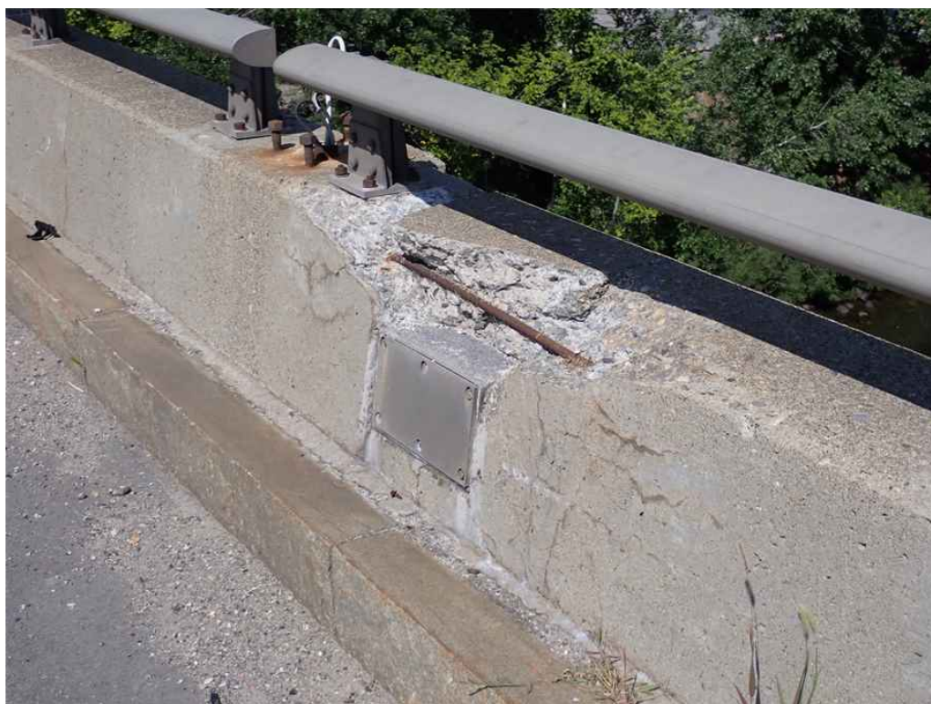
Photo 10: Span 2 north parapet near west end, looking northwest. Typical condition at utility pull boxes.
