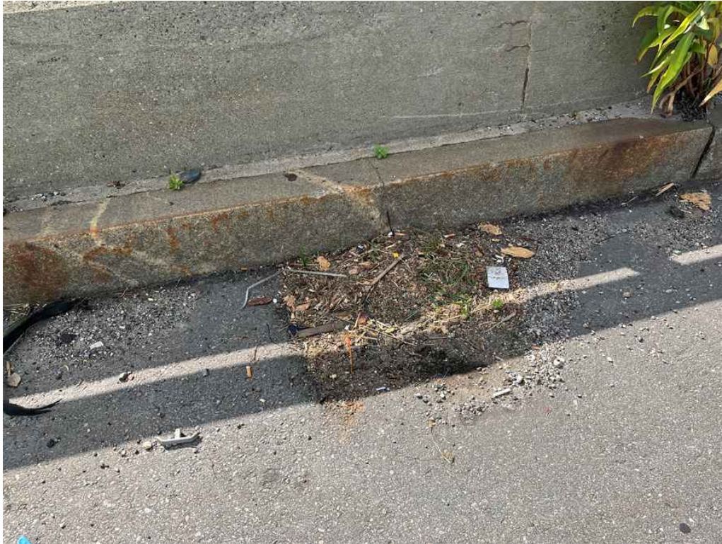
Photo 11: Typical clogged scupper.
